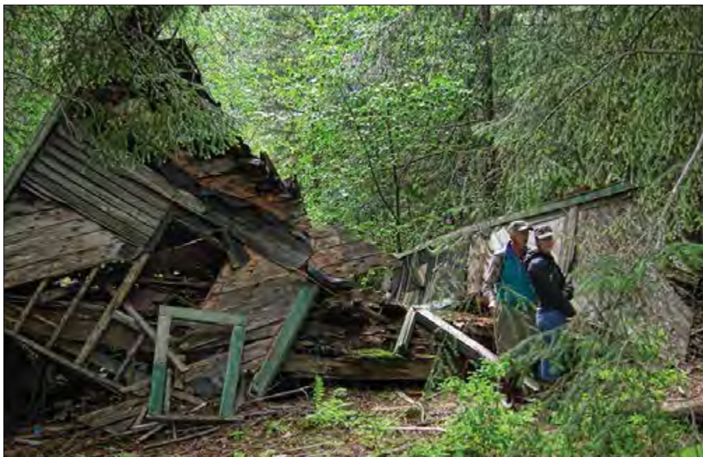
Figure 37. A large two-story building ruin is all that remains of the cannery-era Filipino bunkhouse.
