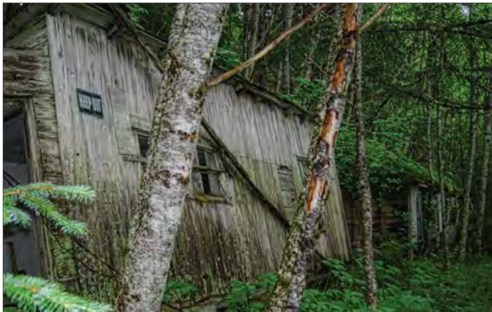
Figure 88. Building B at left lists inland due to a failing foundation. At right are the pair of hip-roofed cabins – Buildings C and D.
