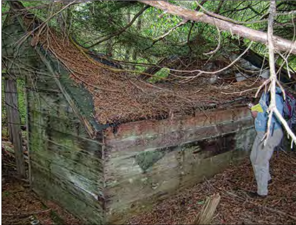
Figure 40. The most intact Aleut cabin is simply constructed of horizontal 1"x8" planks covered with tarpaper, with a central door on a gable wall and few windows.
