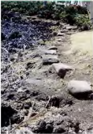
Wave action has eroded the soil around the 'alā stepping stones.
