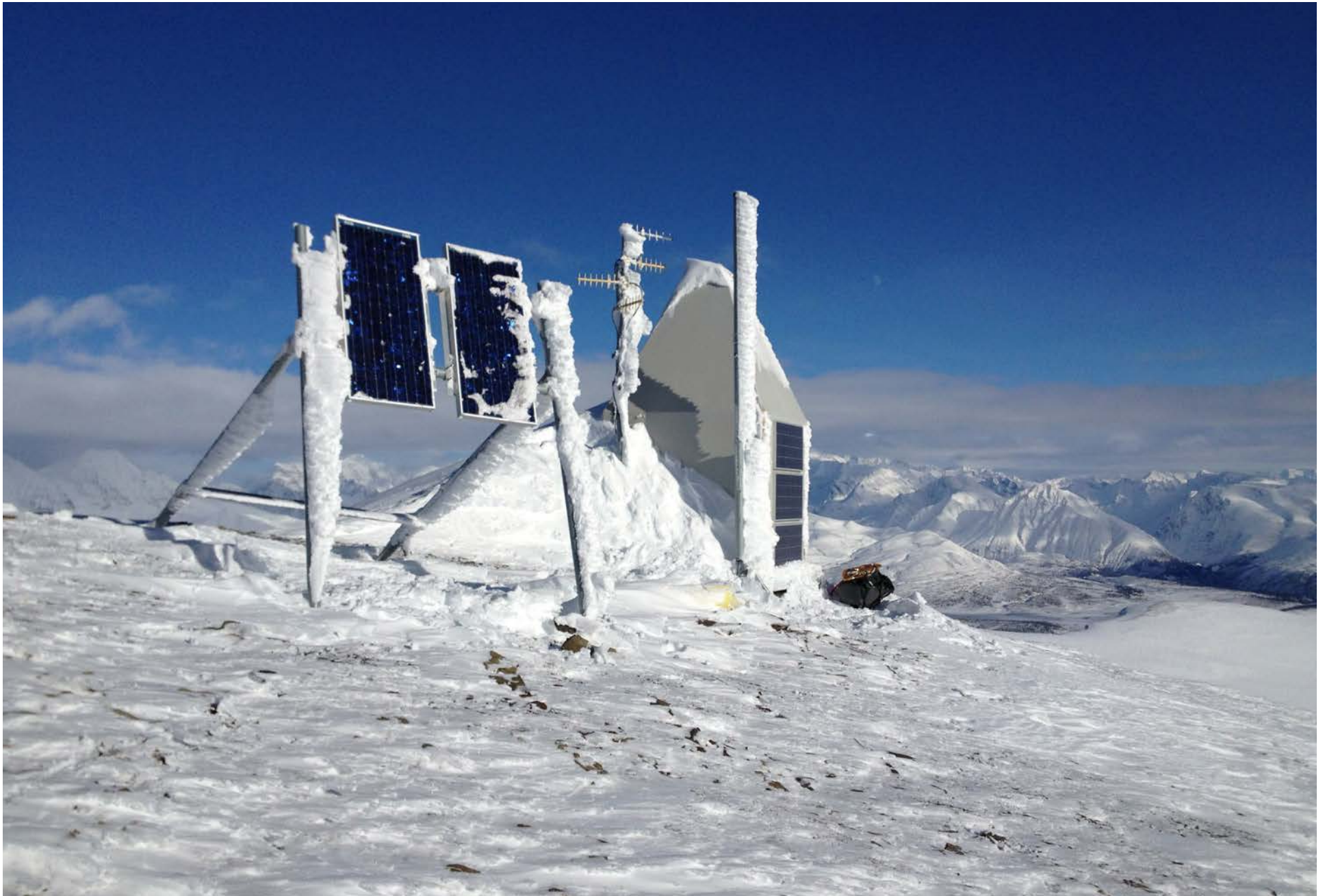
An Earthquake Center seismic station and communications hub on MacColl Ridge in Wrangell-St. Elias National Park and Preserve. The park seismic network not only monitors earthquakes and helps forecast tsunamis, it can detect large landslides and glacial calving events. Photo courtesy of Chris Bruton, Alaska Earthquake Center
