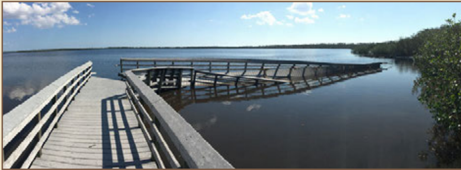
In 2020, the Denver Service Center was managing 193 ongoing hurricane recovery projects, like this one at Everglades National Park. The half-mile boardwalk trail at West Lake was damaged by Hurricane Irma in 2017.
