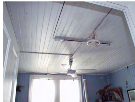
Figure 24 View of ceiling in Room 102. (NPS-SERO-CR, 2002)
