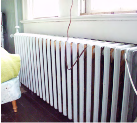
Figure 35 View of radiator in Room 203, which was typical of those installed in the 1930s. (NPS-SERO-CR, 2002)
