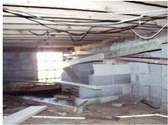
Figure 3 View north in crawl space, showing lattice block used to allow floodwater to pass through the building. (NPS-SERO-CR, 2002)
