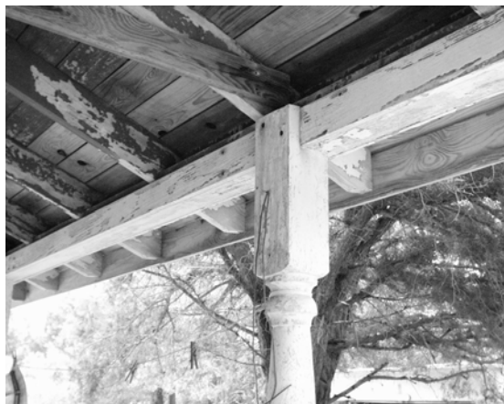
Figure 58 View of typical post, header and roof framing on rear porch. (NPS-SERO-CRS, 2002)
