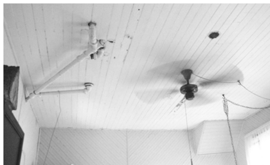
Figure 70 View of ceiling in Room 102, showing cast-iron waste lines (c. 1920) from upstairs bathroom. (NPS-SERO-CRS, 2002)
