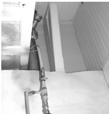
Figure 73 View of large bracket behind and above shower, installed to support water tank at second floor. Note original cornice on rear wall. (NPS-SERO-CRS, 2002)
