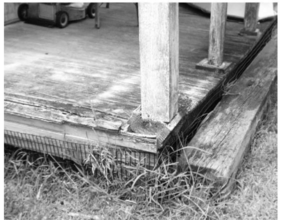
Figure 60 View of northeast corner of front porch, showing corner post seriously destabilized by deterioration of the sills at that location. (NPS-SERO-CRS, 2002)
