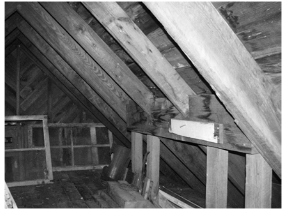
Figure 48 View of roof framing at northeastern end of the building. Rafter at upper right is original; the next two, which are smaller, infill the original opening for the lookout. (NPS-SERO-CRS, 2002)
