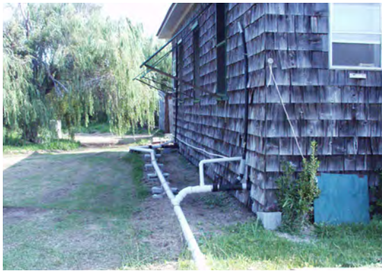
Figure 39 View of waste lines at rear of house. (NPS-SERO-CR, 2003)
