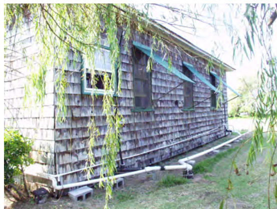
Figure 27 View of rear (northwest) side of house, showing typical exterior finishes. (NPS-SERO-CR, 2002)
