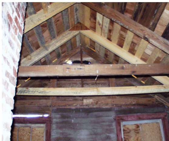
Figure 12 View to northwest Room 202. Historic ceiling has been removed. (NPS-SERO-CRS, 2002)
