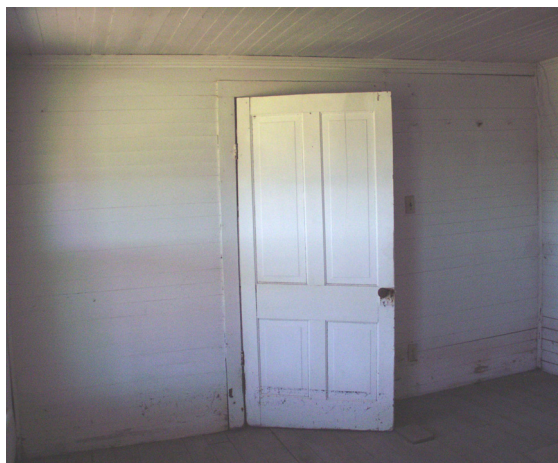
Figure 17 View of south wall of Room 101, showing typical door in house. (NPS-SERO-CRS, 2002)
