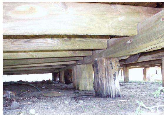
Figure 11 View northeast of front sill, showing typical joist/sill connections and wooden piers. (NPS-SERO-CRS, 2002)
