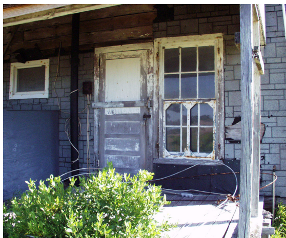
Figure 13 View of original, 6/6 window with typical wood frame for screening. Original location for back door opening was at window at extreme left in this image. (NPS-SERO-CRS, 2002)
