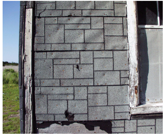
Figure 14 View of added asphalt siding. Note part of shutter hinge on adjacent window casing, which is original. (NPS-SERO-CRS, 2002)
