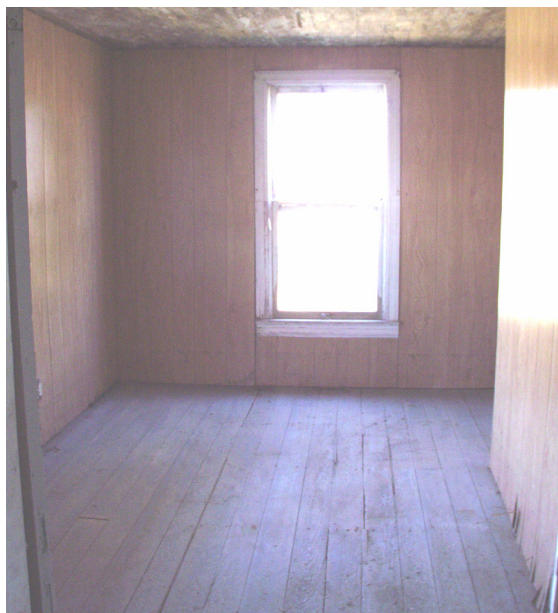
Figure 20 View north in Room 101, showing window that infills earlier door to now-missing kitchen wing. (NPS-SERO-CRS, 2002)
