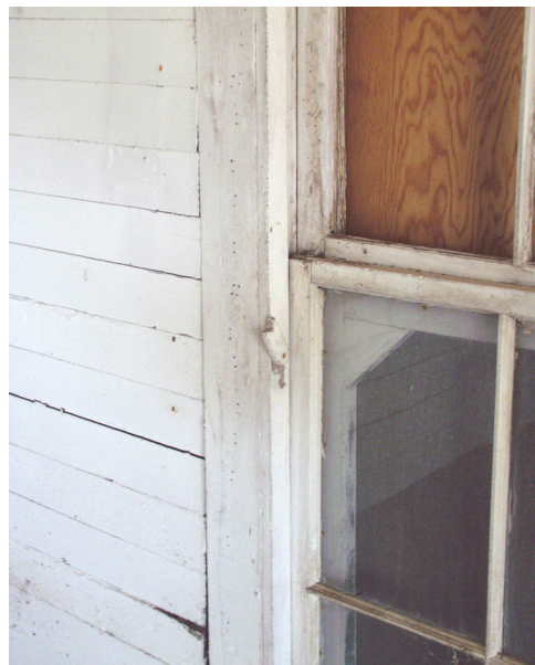
Figure 19 View of typical window casing and wall paneling. Note pivoting sash stay at center, typical of original windows. (NPS-SERO-CRS, 2001)
