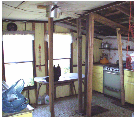
Figure 35 View west in Room 103, showing deteriorated shed-roofed addition that was combined with this room after World War II. (NPS-SERO-CR, 2003)
