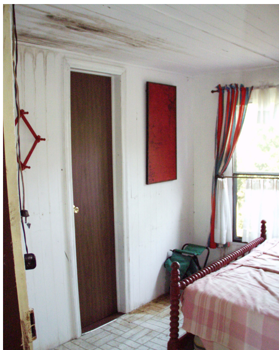
Figure 34 View north of Room 102, showing door added for bathroom. Note water damage to ceiling. (NPS-SERO-CR, 2003)
