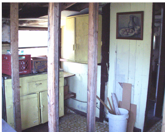
Figure 38 View to north in Room 103. Posts in foreground have been added to stabilize roof structure where wall was removed. (NPS-SERO-CR, 2003)
