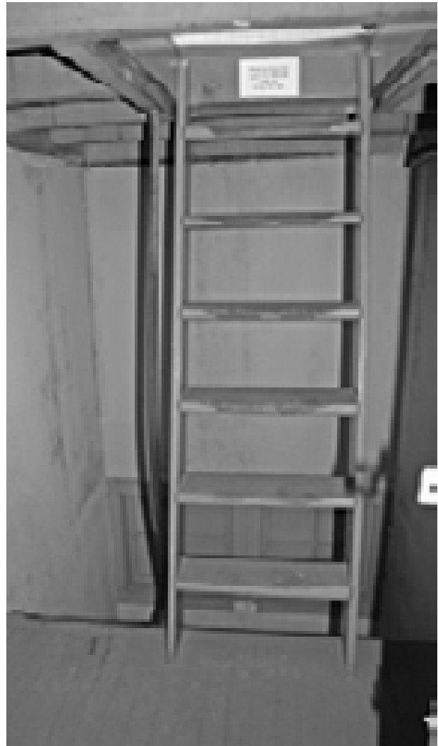
FIGURE 148. View north of attic landing and stairs to watch room from attic door. (T. Jones, NPS, 2005)
