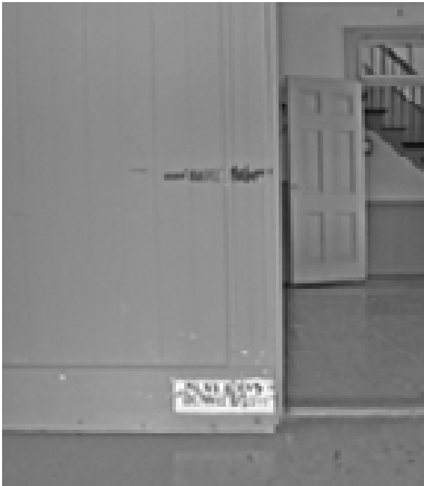
FIGURE 103. View of marks showing high-water marks for recent hurricanes. (T. Jones, NPS, 2005)
