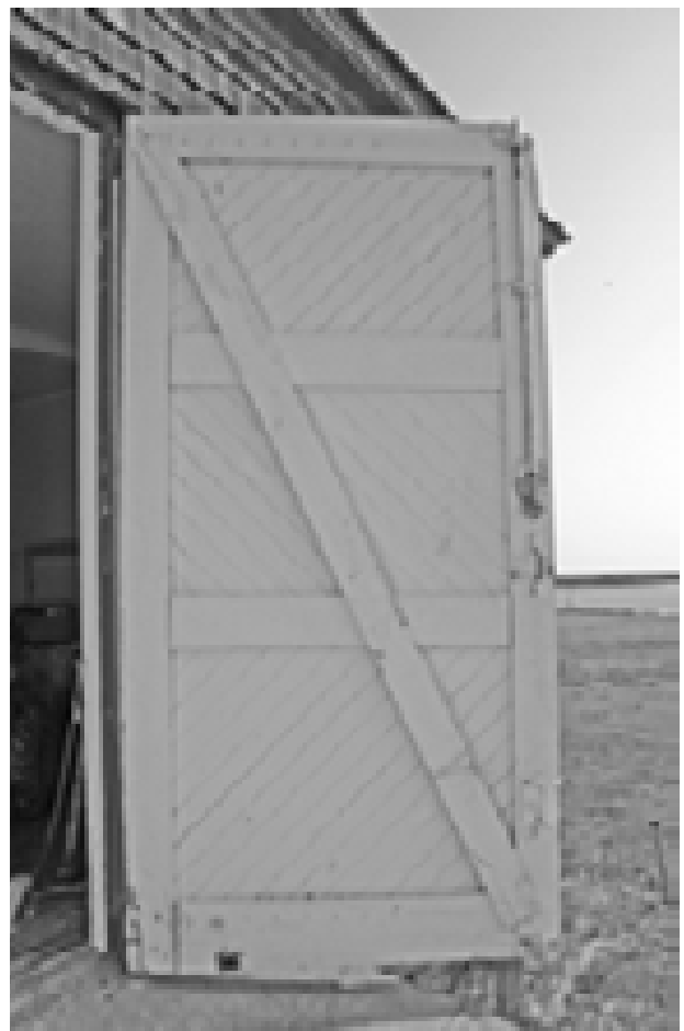
FIGURE 82. View of one leaf of Boat Room door D-3. The diagonal brace is not an historic feature. (T. Jones, NPS, 2005)
