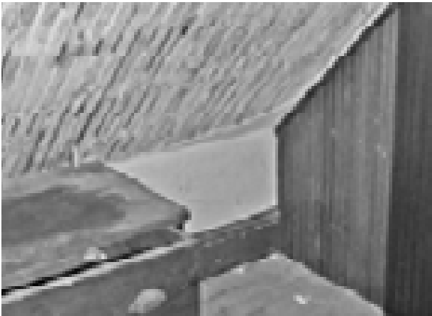
FIGURE 88. View of original plaster on wood lath in one of the closets in Room 201. (T. Jones, NPS, 2005)
