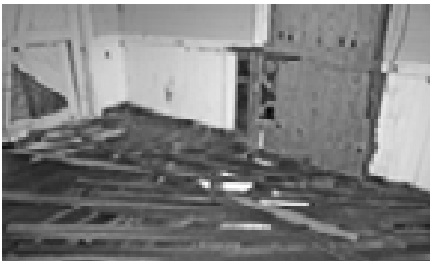
FIGURE 121. View of flooring damaged by storm surge in 1993. (T. Jones, NPS, 2005)
