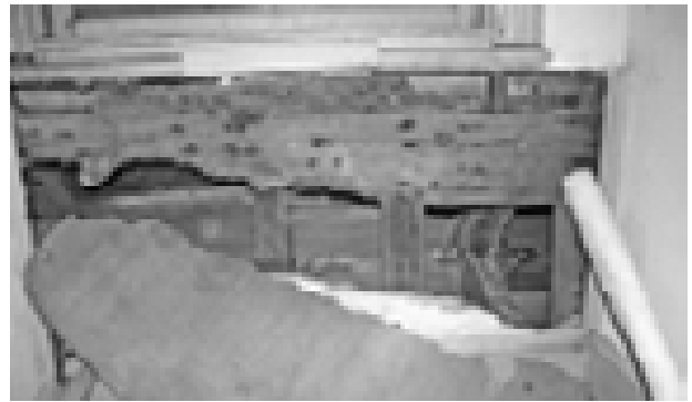
FIGURE 142. View damaged wall below window in Room 202. (T. Jones, NPS, 2005)
