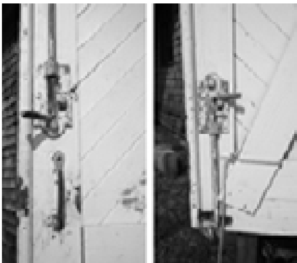
FIGURE 81. View of typical upper (left) and lower (right) sliding bolts on boat room doors. (T. Jones, NPS, 2005)
