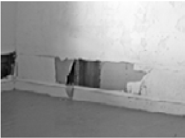
FIGURE 89. View of water-damaged plaster on rock lath in Room 106. (T. Jones, NPS, 2005)
