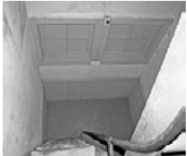
FIGURE 147. View of second floor hall (Room 200) from attic landing. (T. Jones, NPS, 2005)
