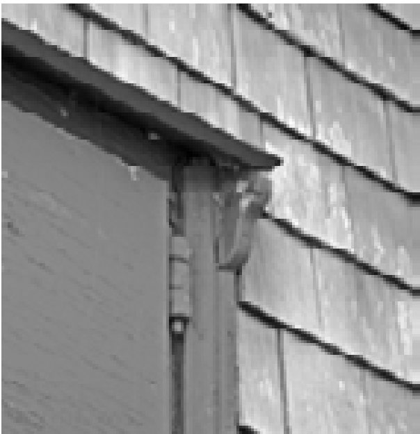
FIGURE 86. View of typical drip cap at Boat Room doors. (T. Jones, NPS, 2005)
