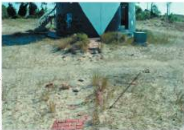
Figure 5-27. The existing historic walk between the lighthouse and the oil shed is in poor condition and is broken by a non-contributing road alignment running through walk. The historic walk should be restored and the non-contributing road removed.
