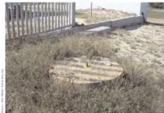
Figure 5-154. Water-related utility features include sinks and septic system features associated with the concrete and metal manhole covers around the Coast Guard Station.
