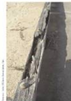
Figure 3-137. Wood has bolted to the edge of the concrete foundation to prevent visitors and vehicles from falling off the edge.
