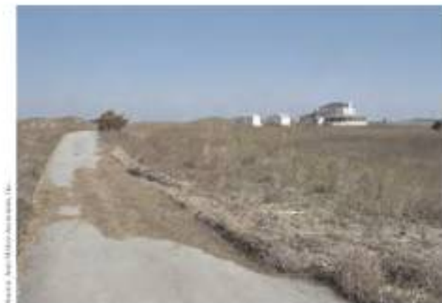
Figure 3-59. Another view of the Concrete Road looking towards Coast Guard. Stormwater has deposited rock across the road surface.
