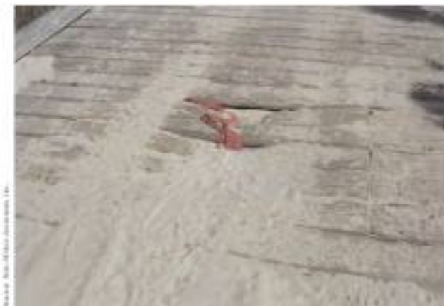
Figure 3-55. A wooden bridge crosses an intermittent driveway as part of a road leading between Back Road and the village precinct. As seen in this photograph, the bridge is in need of repair.
