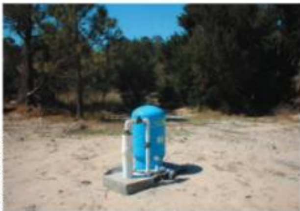
Figure 5-37. New well at lighthouse requiring pumping.
