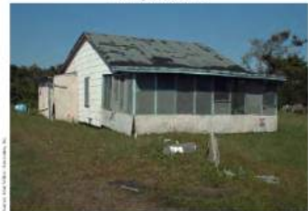
Figure 1-05. The Carrie Annandall Davis (Lawie-Davis) House is significantly deteriorated.
