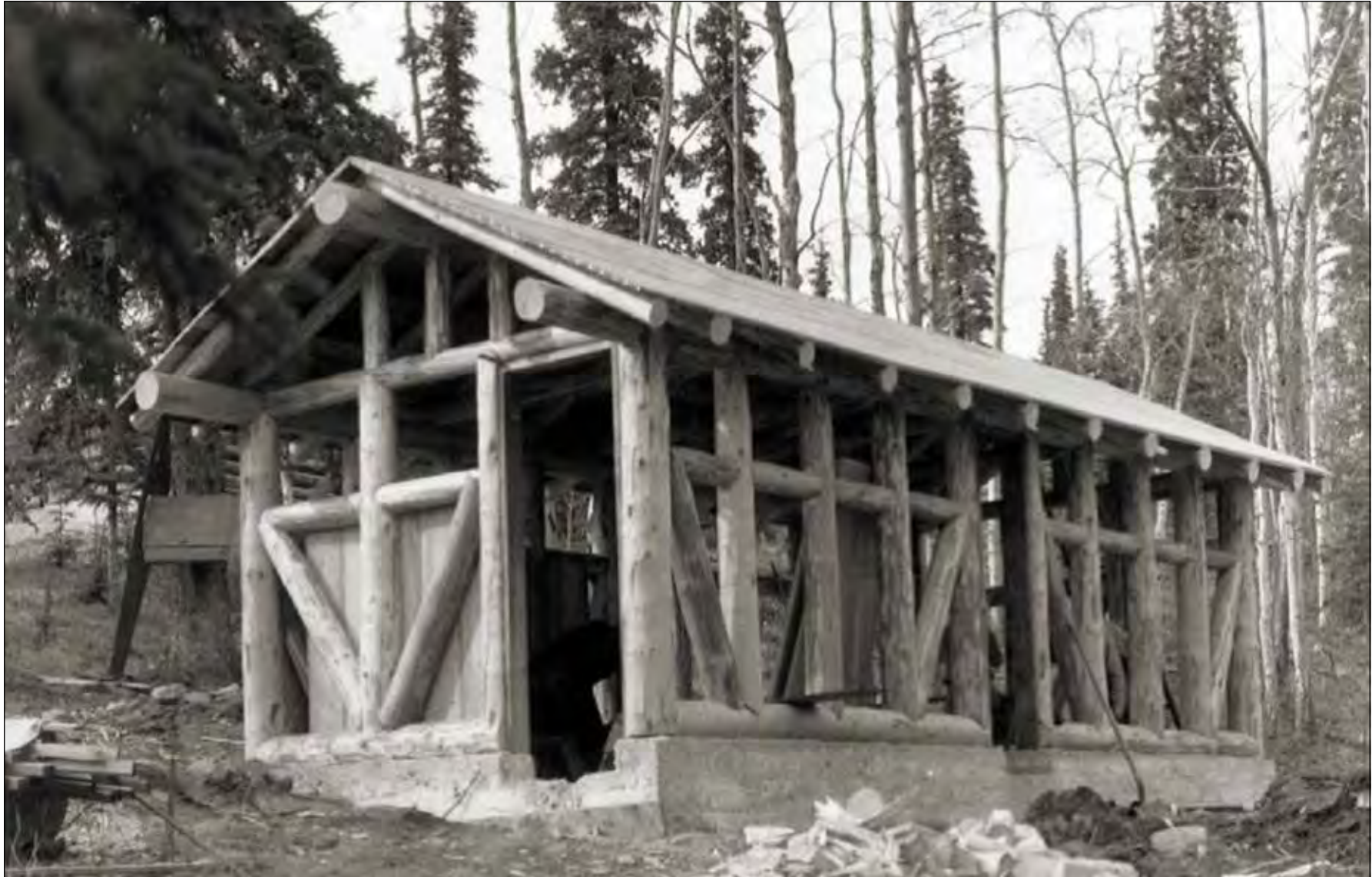
Figure 67. View northwest of the comfort station (Building 112) during construction in 1932(DENA-69-3-43, Harpers Ferry Center)
