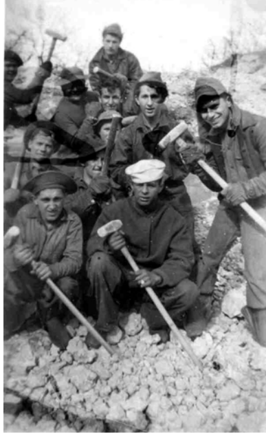
CCC Crew with sledgehammers tearing down the outer wall of the Mortar Battery. Andy Daino is in front center with white hat.
