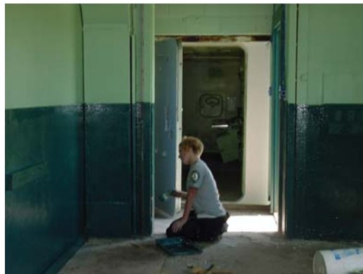
Inside ICC Building 409 during renovations in 2003. Radar van can be seen through doorway.
