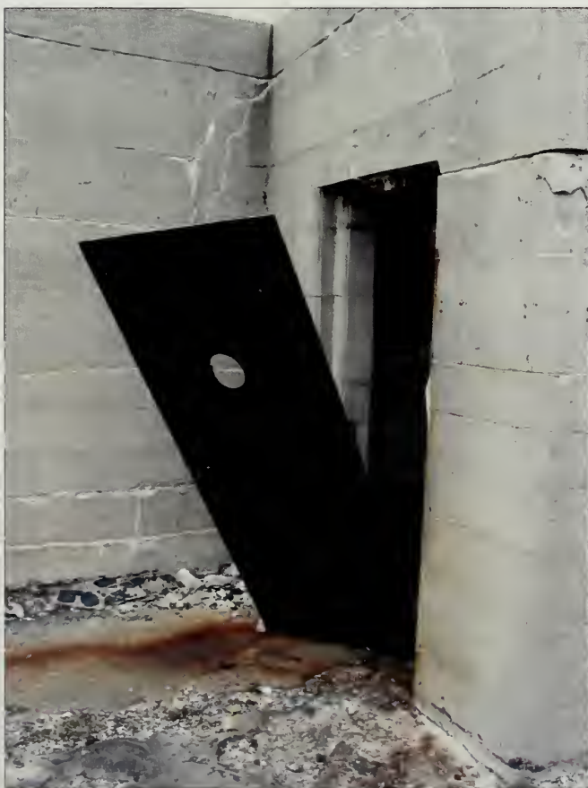
Figure 5.47. View of failing metal door, Nine Gun Battery. Doors and windows should be properly mounted and locked to prevent unauthorized access to interior spaces. While the door in view may be repaired, when a door is damaged or severely deteriorated, a new door should be fabricated to match the existing in materials and finish (Olmsted Center, January 2009).
