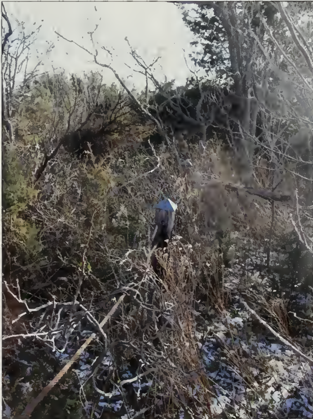
Figure 3.56. Post and wire fence, Battery Kingman. Near the high point above Battery Kingman's emplacement #2, a post and wire fence is installed that is overrun by vines and other vegetation (Olmsted Center, January 2009).
