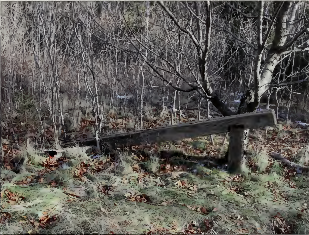
Figure 3.57. View looking east at collapsed wood guardrail, Battery Kingman. Across from both gun emplacements, a series of wood guardrails are installed along the eastern edge of the unpaved road. The guardrails are in fair to poor condition (Olmsted Center, January 2009).
