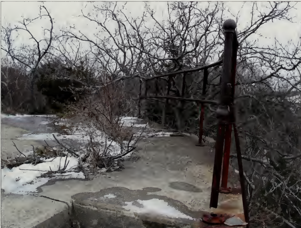
Figure 3.10. View of guardrail south of emplacement #1, Battery Peck. The railings are in fair to poor condition with corrosion covering most pieces. Some assemblies lack any solid material where the vertical members fasten the railing to a solid support (Olmsted Center, January 2009).
