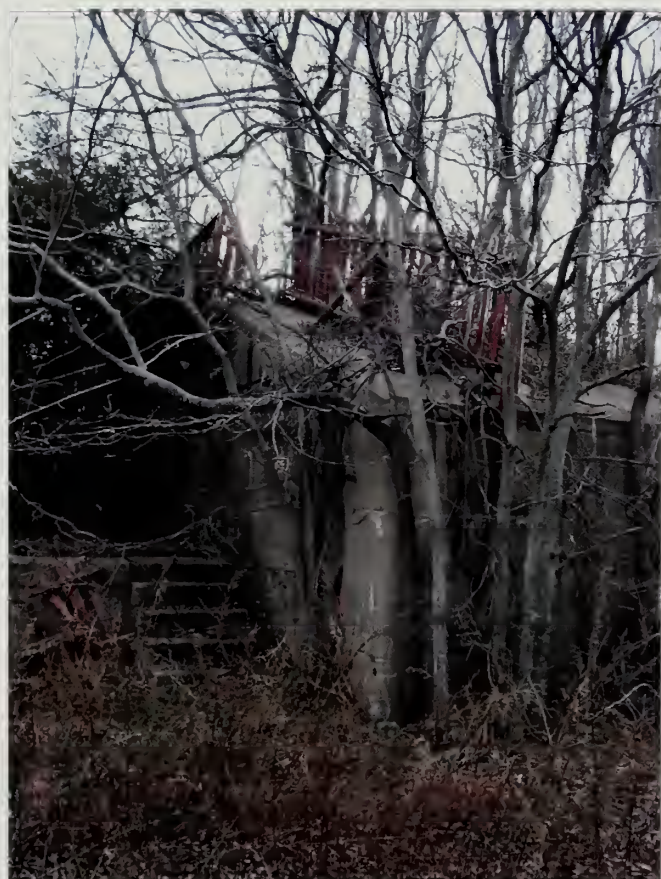
Figure 5.30. View looking northeast at Battery Morris. This image shows dense stands of hackberry ( Celtis occidentalis ) growing directly along the south face of the concrete structure (Olmsted Center, January 2009).
