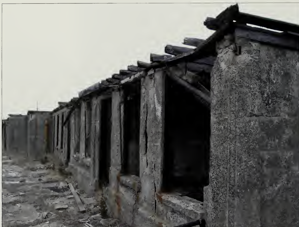
Figure 3.27. Fire control stations, Battery Potter. On the terreplein, two groups of deteriorating concrete structures are located west of the former gun emplacements. The structures served as fire control stations and feature large openings in their east elevations to provide views to the Atlantic Ocean (Olmsted Center, January 2009).
