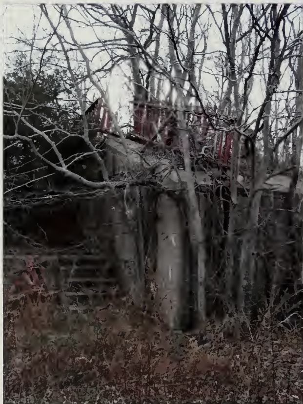
Figure 3.8. View looking northeast at gun platform #1, Battery Morris. A wood picket fence is located to the north and east of the gun platform that is painted maroon red and is in poor condition (Olmsted Center, January 2009).
