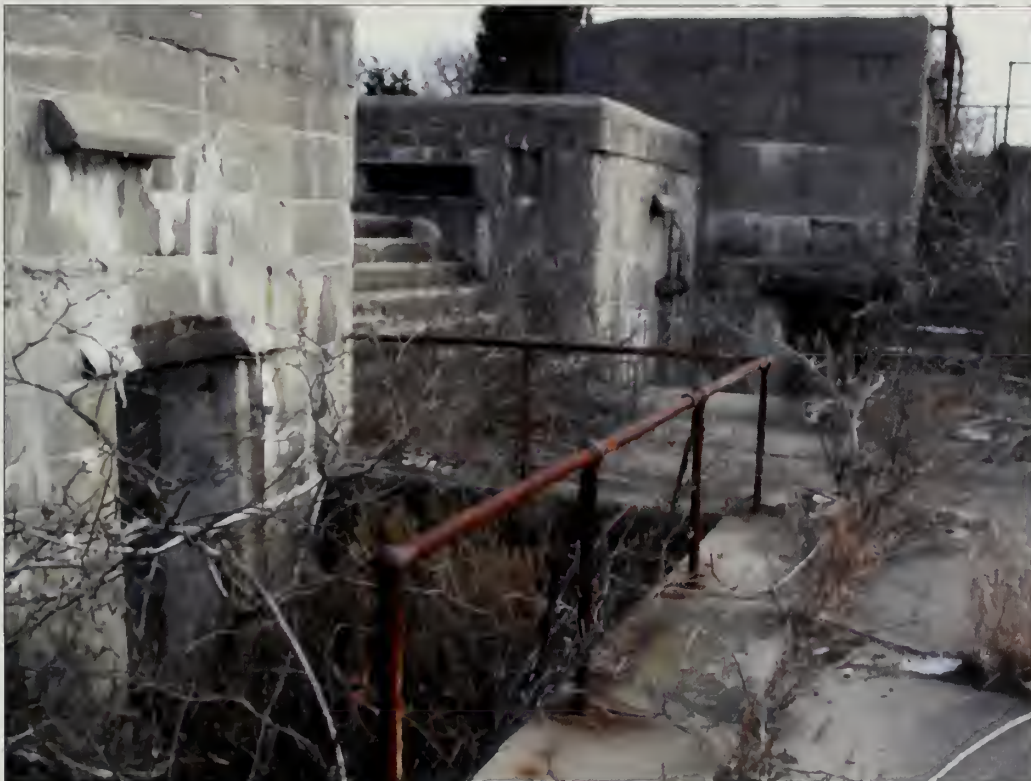
Figure 3.2. View looking northeast at stairwells to magazines, Battery Urmston. Both handrails and guardrails show a heavy degree of corrosion and are staining the concrete below them. Access to existing doors is blocked by vegetation that has grown up in the stairwells (Olmsted Center, January 2009).
