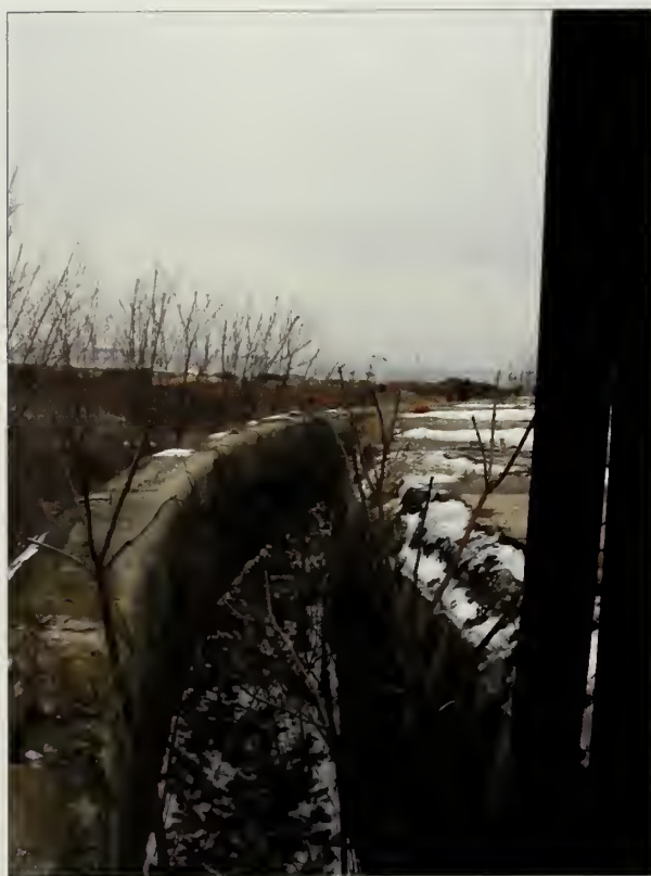
Figure 5.59. View looking east at the chemin de ronde , Battery Potter. Woody vegetation is growing in the chemin de ronde , a designed sentry route located north, south, and east of Battery Potter's superior slope. The vegetation threatens the historic battery's concrete features and surfaces and should be removed. After vegetation removals, the chemin de ronde should be regularly inspected and leaf litter and accumulated debris should be removed to prevent future vegetation growth and to protect the concrete surface (Olmsted Center, January 2009).
