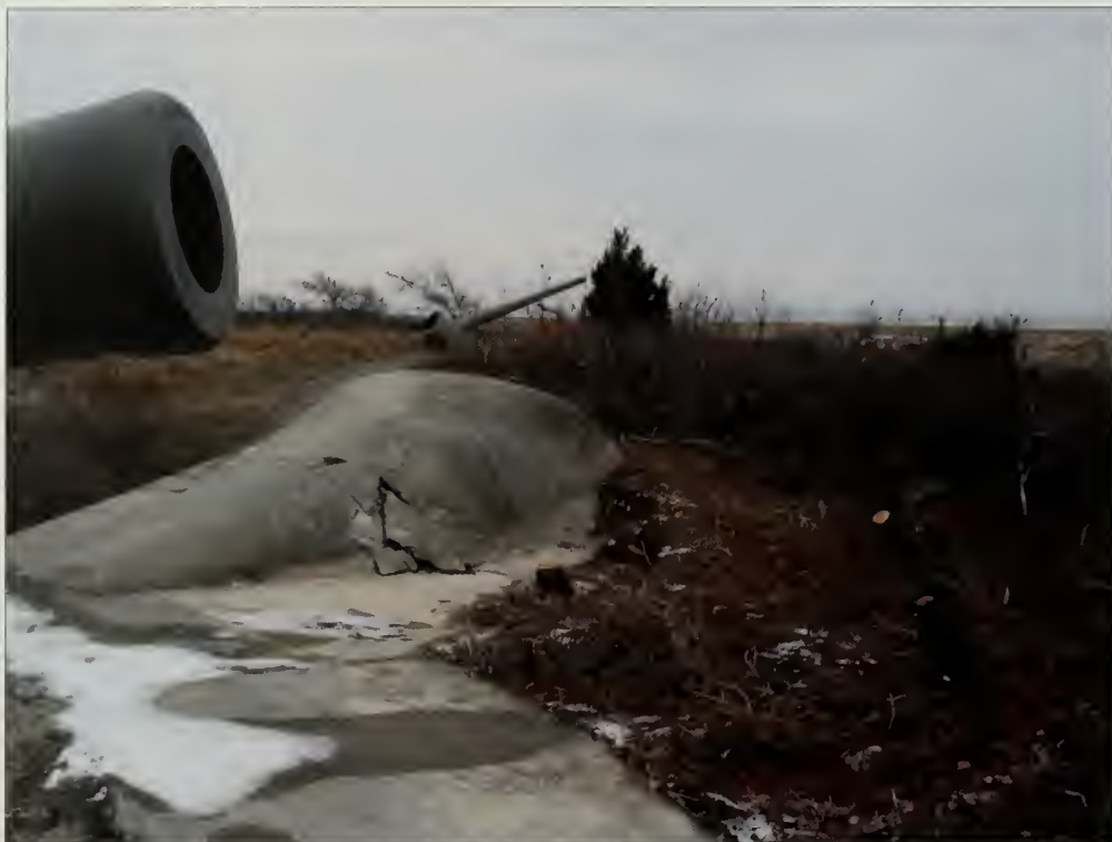
Figure 3.43. View looking north from emplacement #1 to emplacement #2, Battery Gunnison. Spalling is present on a concrete feature due to infiltration of water and freeze-thaw cycles (Olmsted Center, January 2009).
