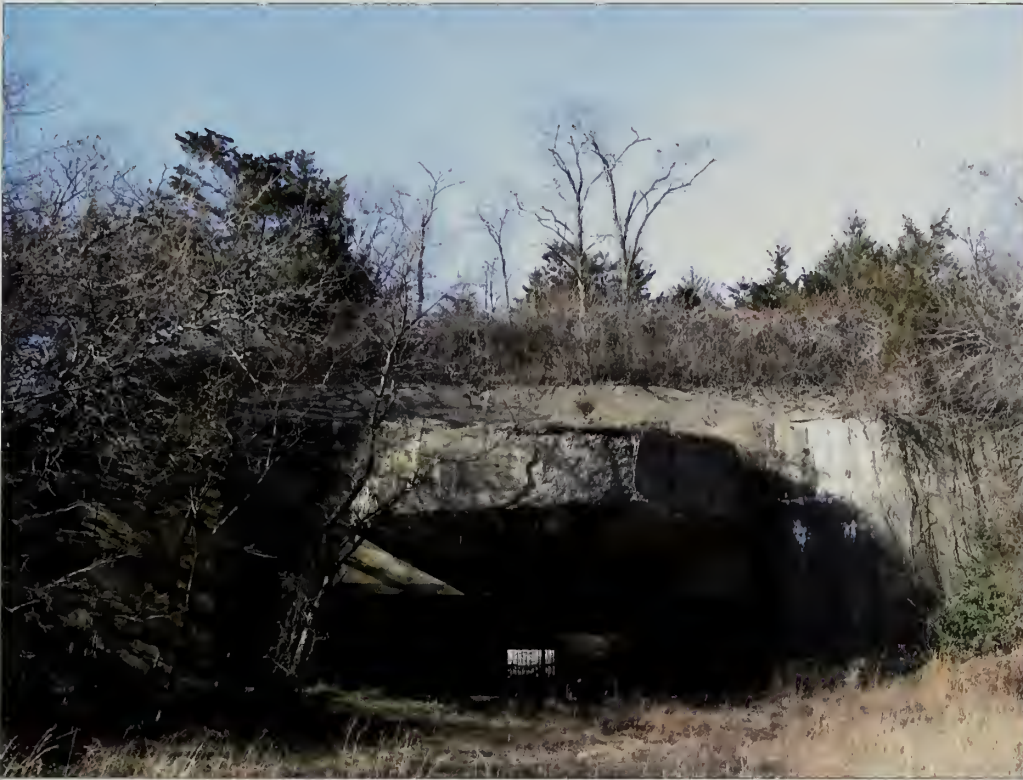
Figure 3.49. View looking west at emplacement #2, Battery Mills. Above the emplacement, large spalling areas on the concrete canopy result from infiltration of water and seasonal freezing and thawing (Olmsted Center, January 2009).
