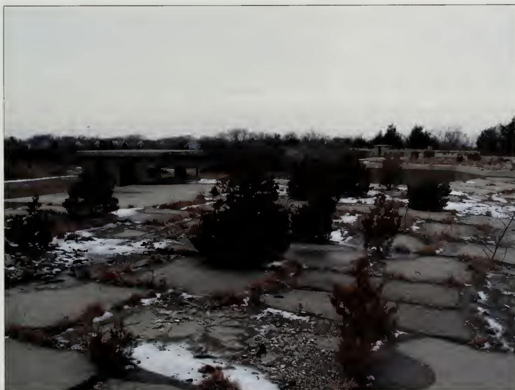
Figure 5.44. View looking west toward battery commander's station Bloomfield, Nine Gun Battery. Eastern red cedars ( Juniperus virginiana ) have become established in the joints of the concrete terreplein and should be removed (Olmsted Center, January 2009).
