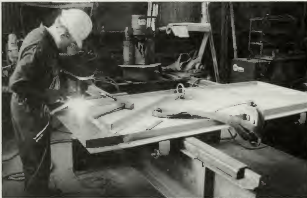
Figure 5.16. Off-site repair of historic metal door for Battery Worth, Fort Casey, Washington. Standing water resulted in the bottom portion of this door being severely deteriorated. The door was removed and is shown being repaired with a new steel plate and angles (From, David M. Hansen, Kimberly Keagle, and Deborah Rehn, Historic Fortification Preservation Handbook , Olympia, WA: Washington State Parks and Recreation Commission, 2003, 3.102).
