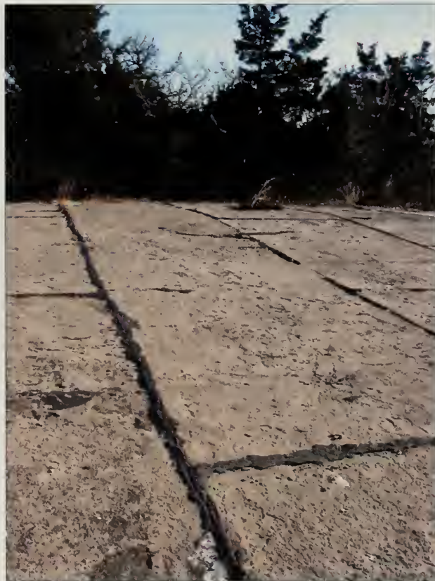
Figure 5.70. Close-up view of existing concrete terreplein, Battery Granger. Existing conditions indicate that joints between concrete panels were once sealed with bituminous material. With the passage of time, this sealant material requires maintenance (Olmsted Center, January 2009).
