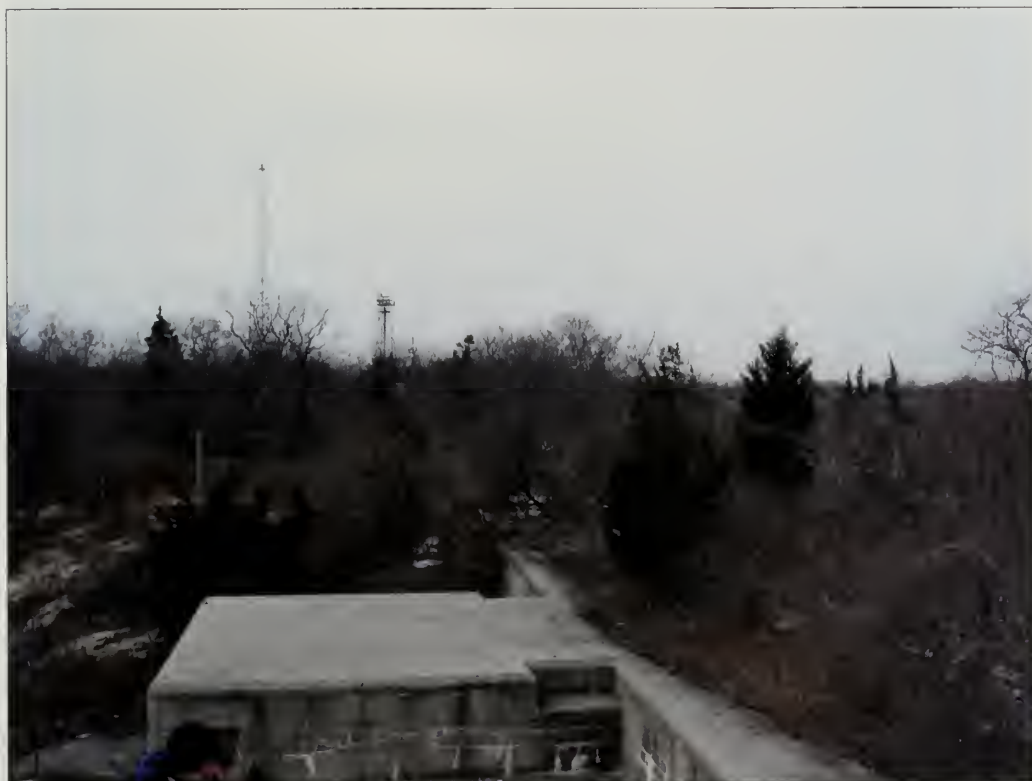
Figure 5.22. View looking west at gun platforms #5 and #6, Battery Urmston. The engineered slope meeting the concrete structure on the west and north sides contains woody vegetation growing on, or within, four feet of concrete structures and should be removed (Olmsted Center, January 2009).
