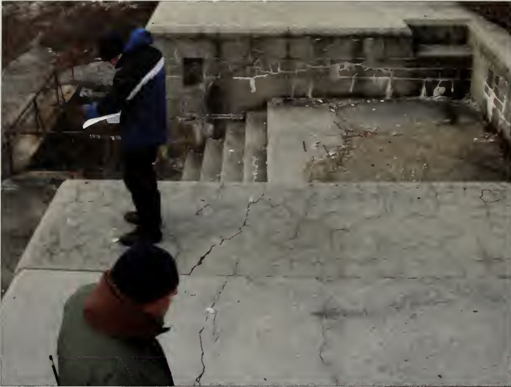
Figure 5.27. View looking down at gun platform #5, Battery Urmston. The tops of the magazines and bomb proofs show less evidence of spalling concrete, yet substantial cracks are present (Olmsted Center, January 2009).
