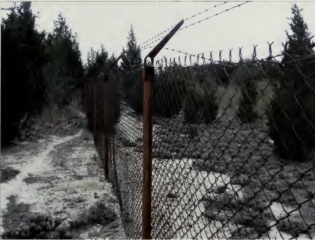
Figure 3.69. Outer fence, NIKE launch site. The launch site features a perimeter fence along its outside boundary and then adds an inner fence that encloses the missile magazines. This section of fence is in fair condition (Olmsted Center, April 2008).
