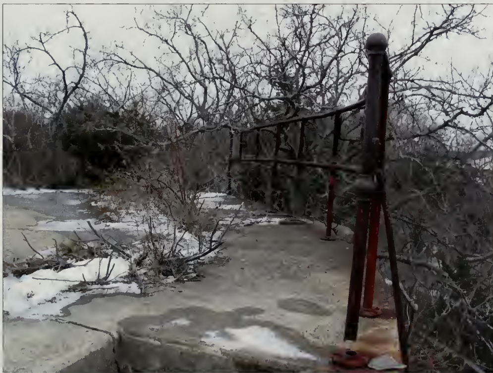
Figure 5.40. View of historic guardrail south of emplacement #1, Battery Peck. Severely deteriorated railing components, such as the vertical post in the foreground, should be removed and replaced with new components that match the original as close as possible. Final painting or a color-galvanized coating should match the historic railing paint finish (Olmsted Center, January 2009).
