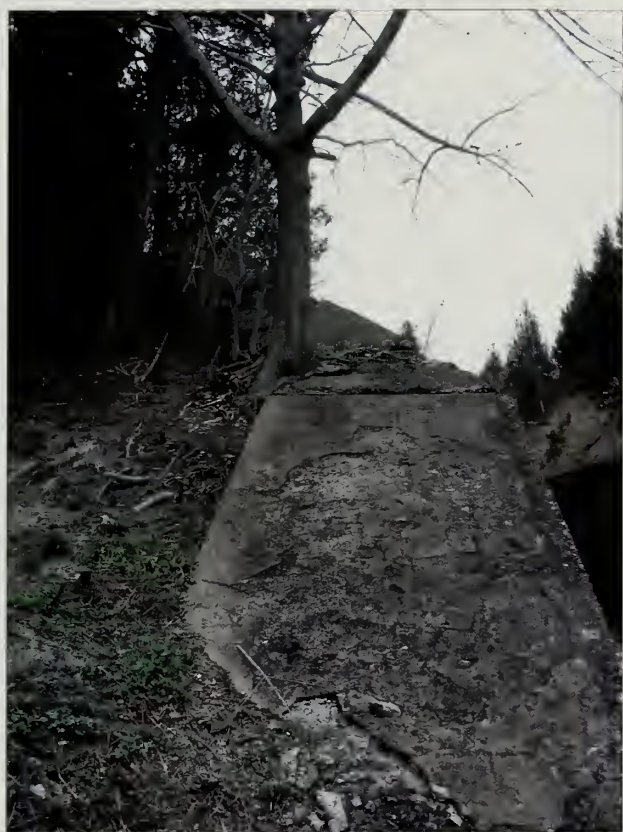
Figure 5.75. View looking southeast at concrete glacis, the Mortar Battery. Here, a tree greater than four-inches in diameter is seen growing directly upon the concrete battery surfaces. Such vegetation must be removed in the interest of long-term preservation of the battery structures (Olmsted Center, April 2008).
