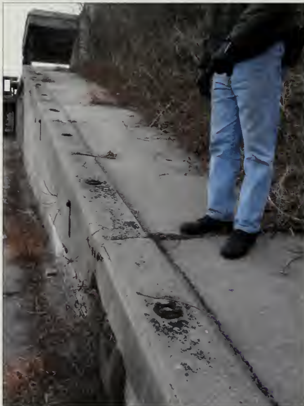
Figure 3.20. View looking northwest at the concrete ramp to gun platform #1, Nine Gun Battery. At transitions between the ground level and gun platforms and also the gun platforms and terreplein, there are stairs and ramps that lack any kind of railing. This ramp has escutcheon plates but lacks a guardrail (Olmsted Center, January 2009).
