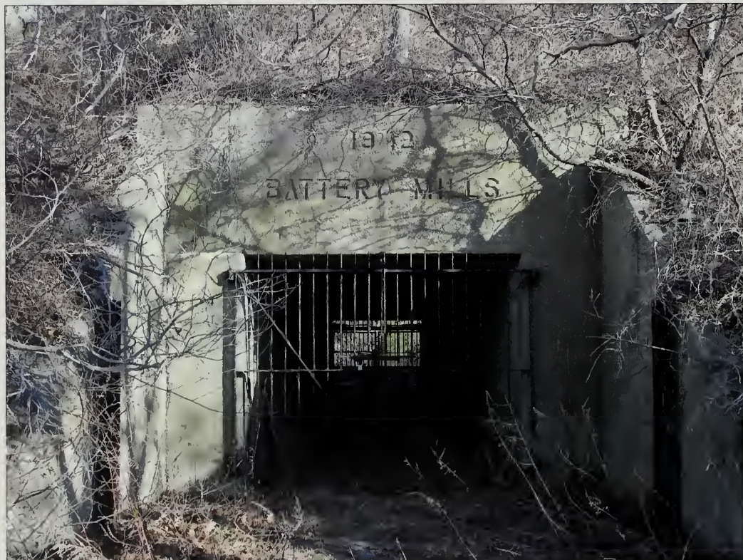
Figure 5.90. View looking east at a bulkhead entry, Battery Mills. All woody vegetation growing on or within four-feet of concrete features like the bulkhead entries should be removed (Olmsted Center, January 2009).
