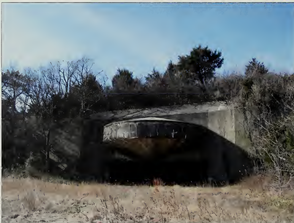
Figure 3.48. View looking southwest at emplacement #2, Battery Kingman. Designed to shield the gun platform from overhead fire, the concrete canopy exhibits efflorescence indicating water is infiltrating the concrete and drawing out impurities to the surface (Olmsted Center, January 2009).
