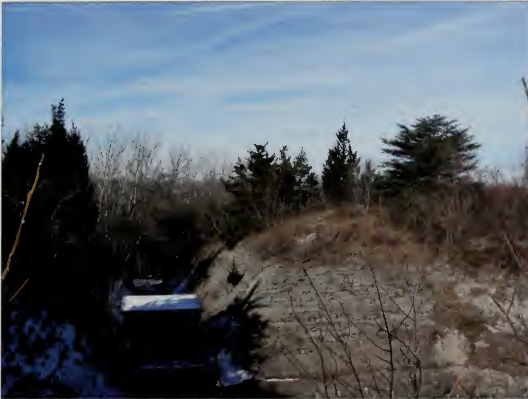
Figure 3.37. View looking west across southwest mortar pit, the Mortar Battery. Efflorescence and spalling are present on the concrete blast slope above the mortar pit. These symptoms of water infiltrating concrete can be seen on additional horizontal and vertical concrete surfaces at the Mortar Battery (Olmsted Center, January 2009).
