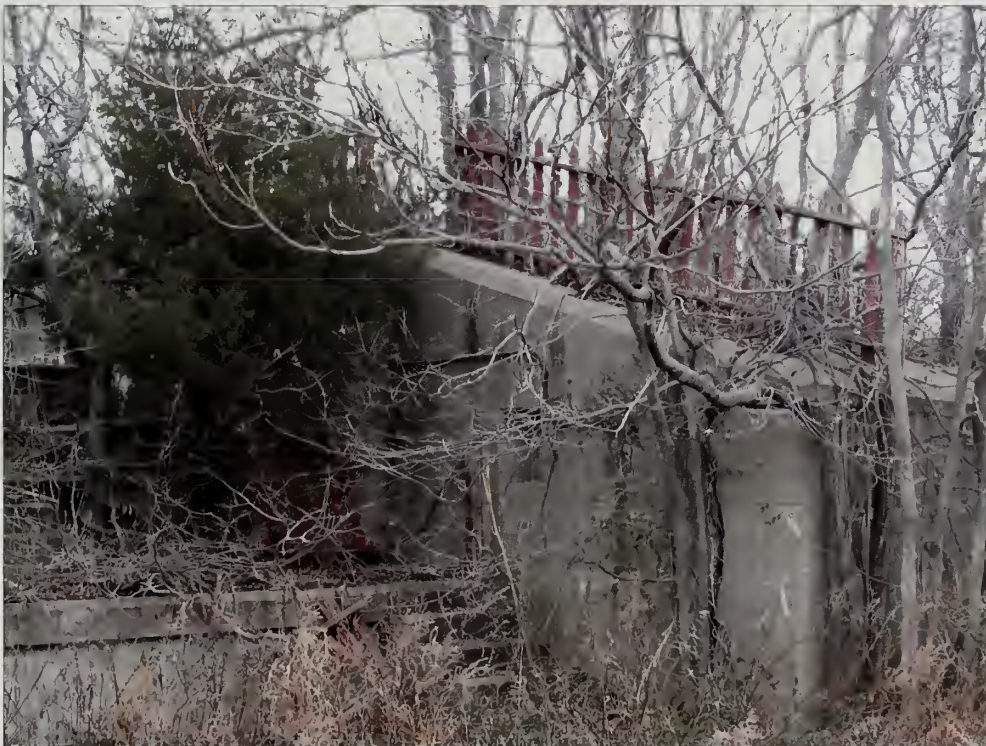
Figure 5.34. Wood picket fence on top of Battery Morris. The entire length of the pictured non-historic fence should be removed. Great care should be exercised not to damage the historic concrete structures and the historic earthwork north of the battery when the posts are removed (Olmsted Center, January 2009).
