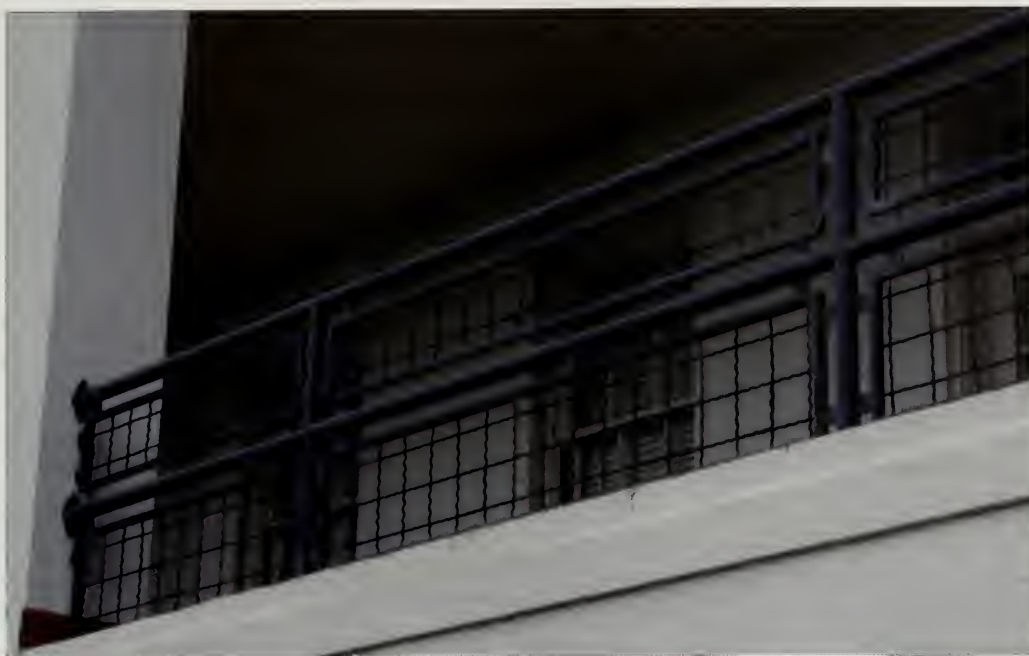
Figure 5.13. Example of the infill approach to retrofitting railing systems for compliance with life-safety codes. In the wide openings between the horizontal pipe rail members, a mesh panel framed by square bar stock has been added. The frame is connected to the existing pipe rails by welding metal tabs between the two (Barbara Judy, Golden Gate National Recreation Area).
