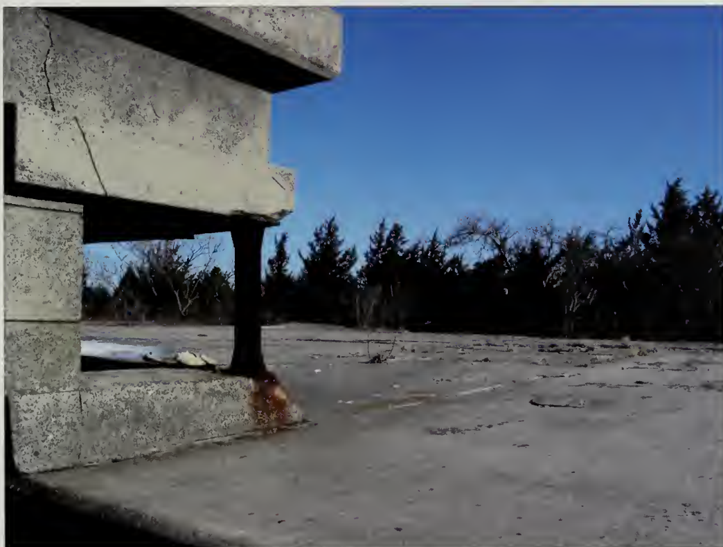
Figure 5.68. Blocked view northeastward from the battery commander's station at Battery Granger. Blocked downrange views to the water makes it difficult for park visitors to understand the historic operation of these coastal defense sites. Note corrosion of ferrous metal building features (Olmsted Center, January 2009).
