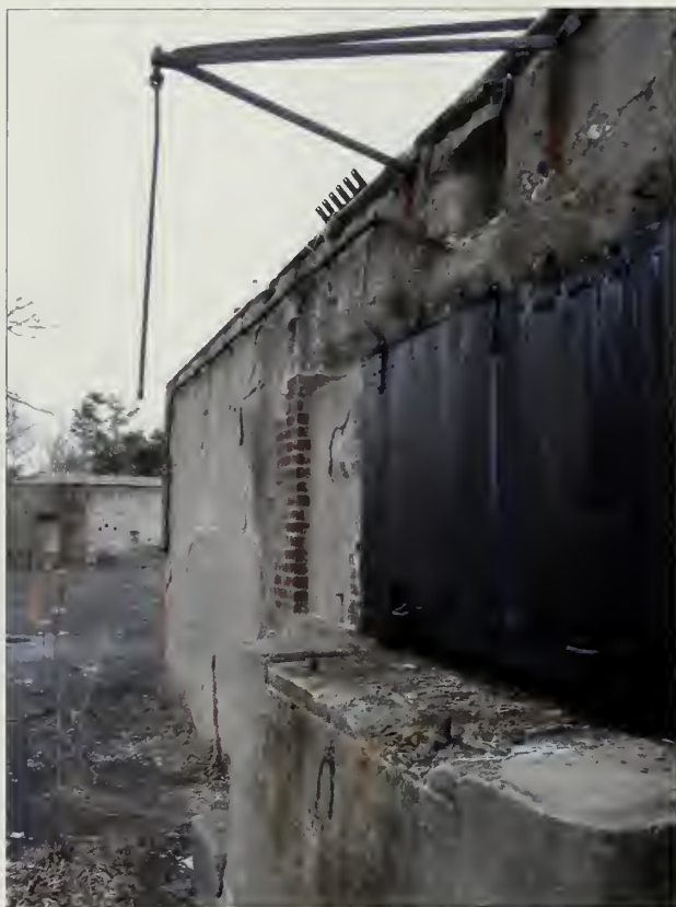
Figure 5.48. View of shell hoist metal door, Nine Gun Battery. Doors and windows should be properly mounted and locked to prevent unauthorized access. If a door is damaged or severely deteriorated, a new door should be fabricated to match the existing in materials and finish (Olmsted Center, January 2009).
