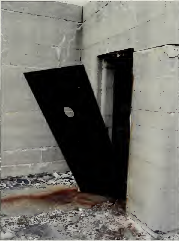
Figure 3.17. View of failing metal door, Nine Gun Battery. Several dozen doors and windows are missing or not properly mounted at the magazines, commander's stations, and other auxiliary rooms at Nine Gun Battery (Olmsted Center, January 2009).
