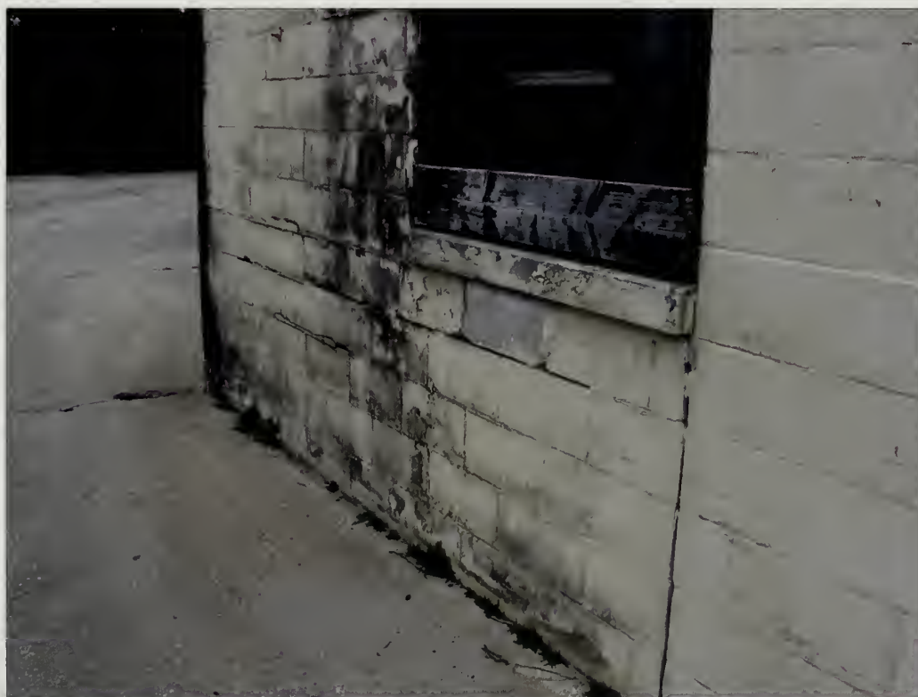
Figure 5.121. View looking northwest at Warhead Building (450), NIKE launch site. Routine maintenance procedures will help stabilize free-standing buildings in the launch site. The water damage seen in this image originates from a metal gutter mounted at the top of the wall that needs to be cleaned and reset so water is carried away from the building (Olmsted Center, April 2008).
