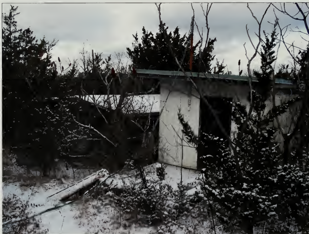
Figure 5.115. View looking northwest at the kennel buildings, NIKÉ launch site. Vegetation removals around existing buildings should focus on the generator building (429) and kennel buildings (457 and 458) as these structures are becoming enveloped by overgrown vegetation (Olmsted Center, January 2009).
