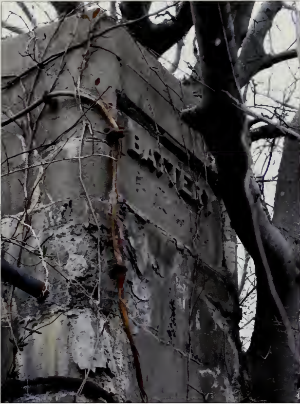
Figure 3.9. View looking northeast at corner of structure, Battery Peck. Efflorescence can be seen on many of the vertical surfaces and spalling is present on both horizontal and vertical surfaces indicating water has penetrated the concrete and is damaging the material (Olmsted Center, January 2009).
