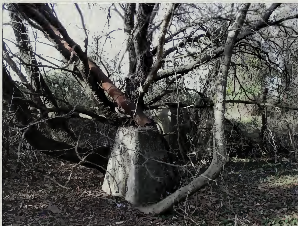
Figure 3.52. View looking northwest from the top of Battery Mills. A tapered concrete box and metal pipe are located near the center top of the engineered earthwork. These structures are most likely associated with ventilation or served as flues for furnaces (Olmsted Center, January 2009).
