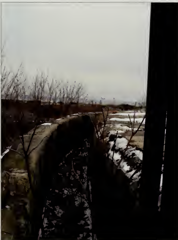
Figure 3.34. View looking east at the chemin de ronde , Battery Potter. The chemin de ronde is presently a collection area for leaf litter and debris that supports the growth of woody vegetation (Olmsted Center, January 2009).
