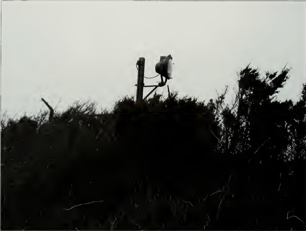
Figure 3.71. Floodlight, NIKE launch site. At the Missile Magazine area, eight floodlights are positioned along the inner fence. Each light features a parabolic fixture mounted with a metal bracket to a wood pole. Six similar lights are located at the Missile Maintenance Area on the engineered earthworks (Olmsted Center, April 2008).
