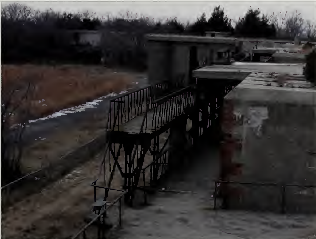
Figure 3.18. View looking west at battery commander's station Halleck, Nine Gun Battery. A cantilevered structure between emplacements #5 and #7, intended to provide access to the commander's station, is in poor condition (Olmsted Center, January 2009).
