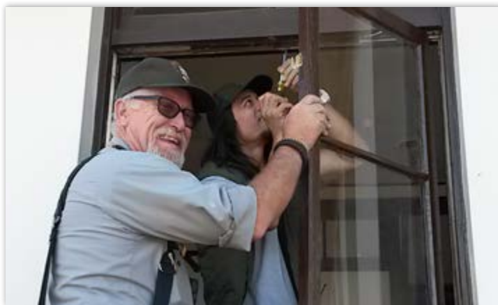
NPS crews repair windows on historic park buildings to help save energy.
