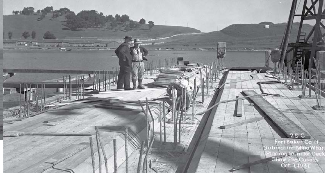
As early as 1937, as part of the pre-war mobilization effort, the army constructed a submarine mine wharf to allow large mine planter ships to dock at Horseshoe Cove. The new wharf, built with concrete and pilings, was a large-scale construction project abutting the 1903 quartermaster supply wharf. Note Fort Baker's open landscape in the background. (Photo circa 1937)
