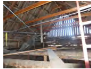
Hay Mow floor missing
