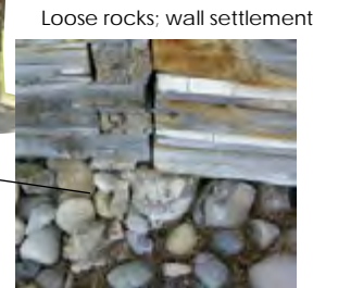
Loose rocks; wall settlement
