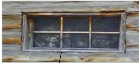
4 Construct sash with muntins matching those on east side. Do not install trim.
