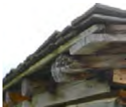
Rafter ends deteriorated
