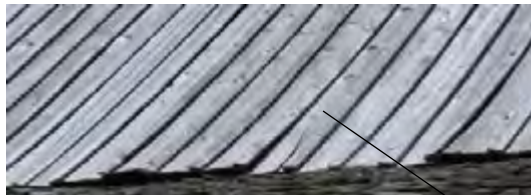
Board and batten roofing with serious check; lifting
