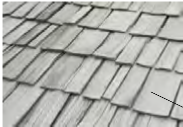
Wood shakes improperly laid, checking. Roof leaks.
