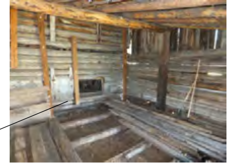
Interior flooring and stalls damaged and deteriorated
