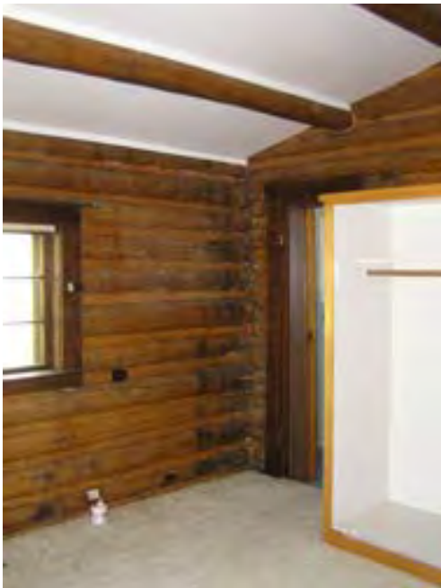
Figure 176 – Looking northwest at the walls in the southwest bedroom. Most of the materials are in good condition. It appears that there is some water staining on the log work.
