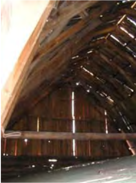
Figure 205 – Looking south at the structure of the gambrel roof and end. Note the openings in the roof and gambrel end. There is some rot in the wood structure. Note the sheet asphalt roof of the structure below.
