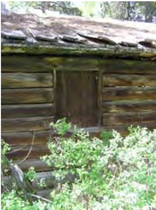
Figure 185 – Looking east at a section of the wall and roof. Note the deteriorated log walls and the warping of the boards on the roof.
