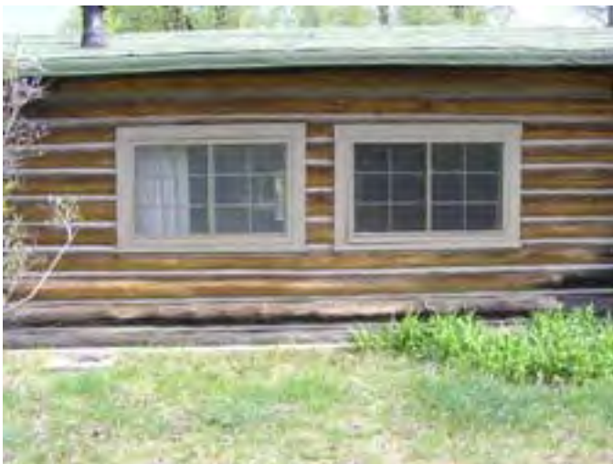
Figure 28 – Looking east at a typical log wall on the west side of the Lodge. The logs are very dry and there is some surface rot on the bottom logs and under the valley areas where water drains onto the logs. The concrete foundation appears to be in good condition. The grade around does not slope away from the building so there is no positive drainage.
