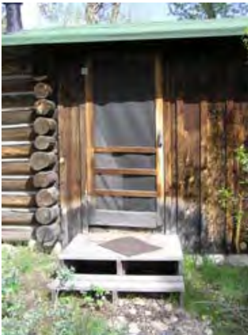
Figure 84 – Looking east at the entrance door to the wood frame addition. The porch and base of the addition and logs have some rot.
