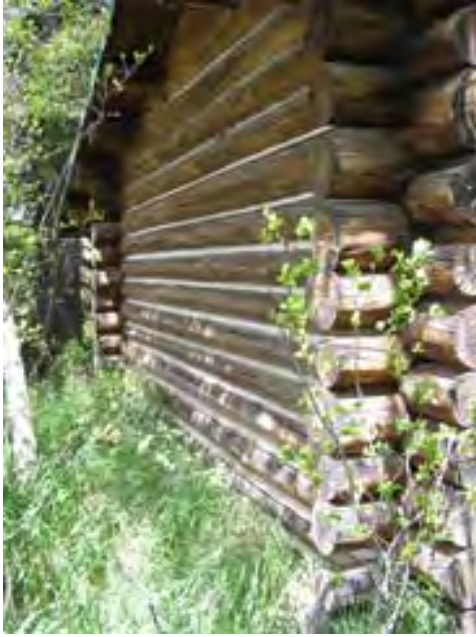
Figure 112 – Looking north along the west side of the building. The problems are typical in this area also.
