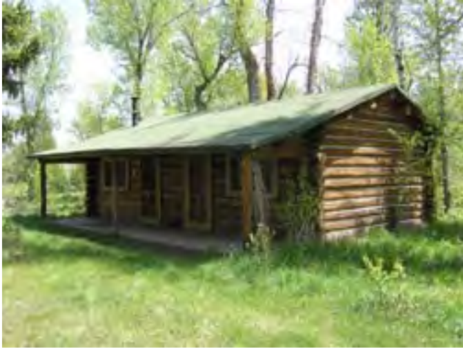
Figure 129 – Looking southeast at the cabin and front porch. The roof is good with some minor damage along the porch eave.
