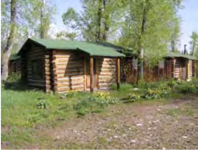
Figure 70– Looking northwest at the cabin. The building is generally in good condition with the exception of rotted sill logs and base of the frame structure. Soil has built up around all sides of the building.
