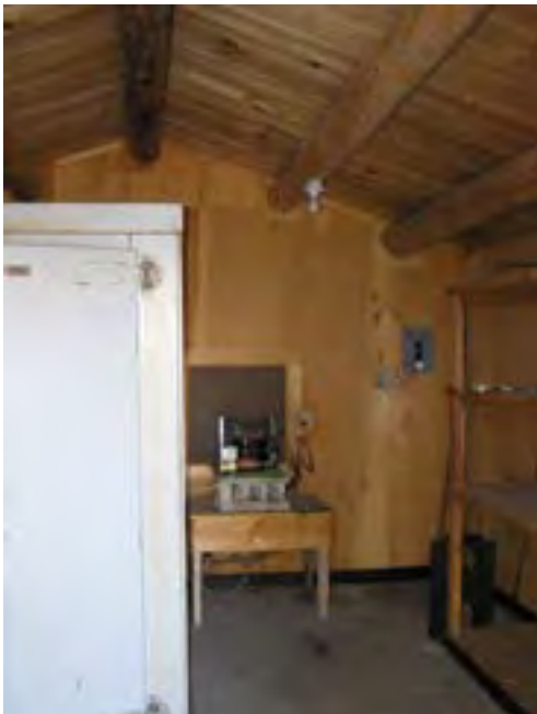
Figure 98 – Looking south at the Ice House interior. The materials are in good condition. The coolers are still in this building.
