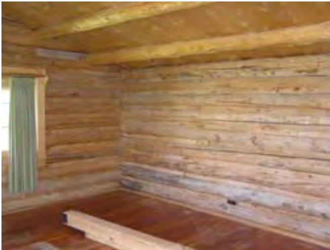
Figure 65 – Looking southeast at the back wall of the cabin. It appears that there has been some water penetration into the back wall as the base logs are stained.
