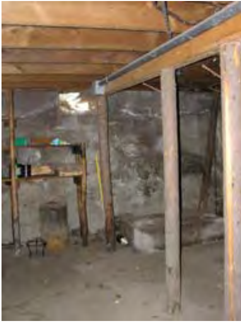
Figure 38 – Looking west at the basement under the kitchen. Note the concrete walls and floor and the added supports for the kitchen floor. There are some water stains on the concrete from some water penetration into the wall.
