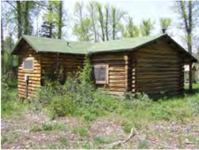
Figure 121 – Looking northwest at the cabin. Note the vegetation and soil build-up around the base, which is causing rot in the sill log and base logs of the wall. The wall logs are dry but the daubing is generally good.
