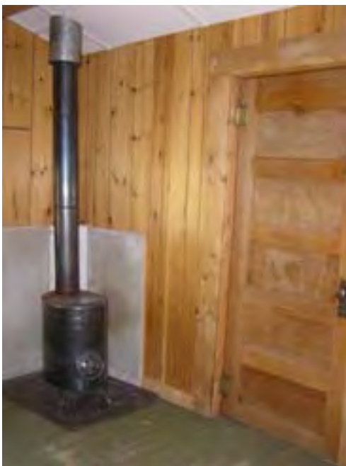
Figure 81 – Looking northeast at the wood stove and wood paneled exterior door in the north bedroom (possible asbestos heat shield behind wood stove).
