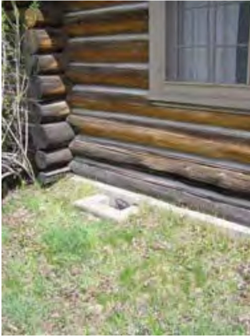
Figure 29 – Looking northeast at a typical corner of the Lodge. Note the rotted bottom logs and the soil that has accumulated against the log ends. Also note the concrete vent to the crawl space that allows air under the building.
