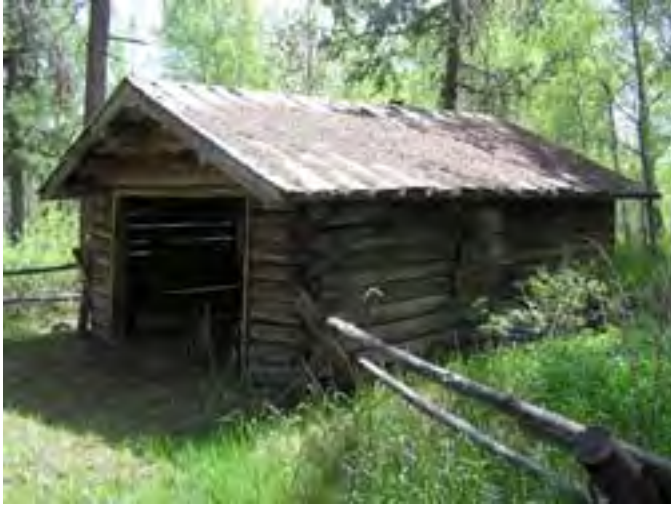
Figure 183 – Looking southeast at the garage building. The board-on-board roof is weathered and showing some leakage of water. The two side walls at the opening have moved out at the bottom.
