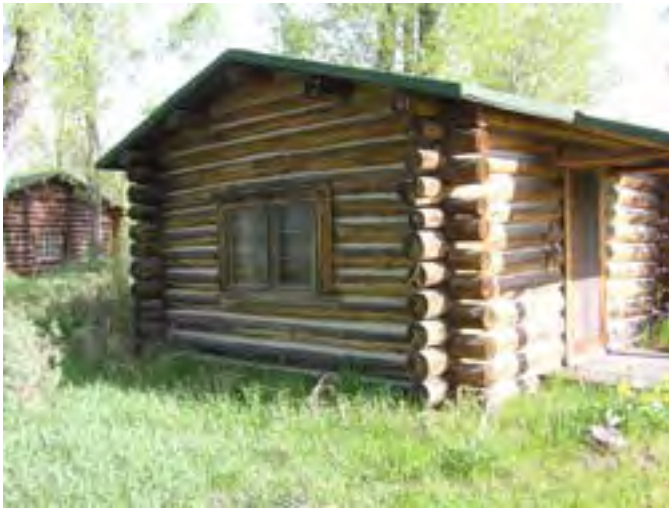
Figure 71 – Looking northwest at the log cabin on the south end of the building. Note the sag in the base due to rotted sill logs.
