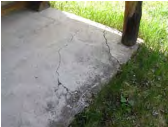
Figure 120 – Looking southwest at the concrete porch and column base. Note the cracks in the slab from the weight of the roof and column. (As the concrete appears to have been poured around the column bases, it is not possible to determine whether or not they have separate footings without destructive investigation.)
