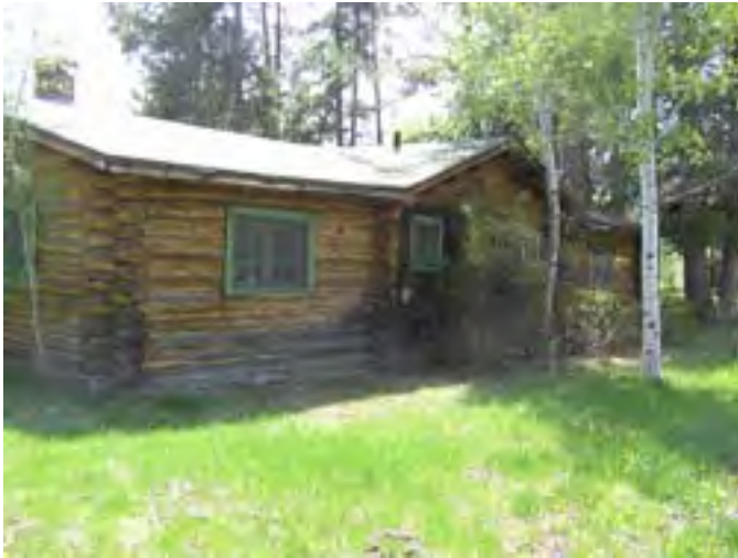
Figure 162 – Looking southeast at the Caretaker's House showing the log sections and the infill in the original recessed porch area. The roof is in good condition with some minor damage on the eaves.
