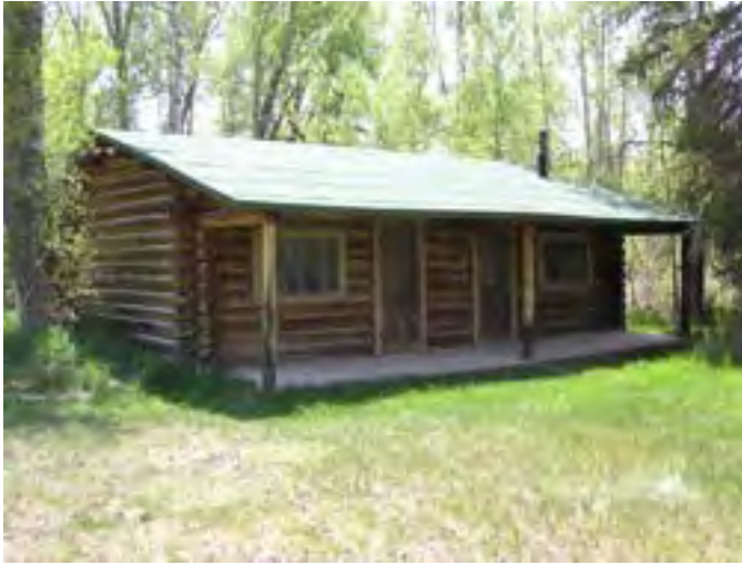
Figure 106 – Looking southwest at the cabin and the front porch and entrance. The roof is in good condition. The doors are in good condition but the screen doors are weathered and the wood is dry.
