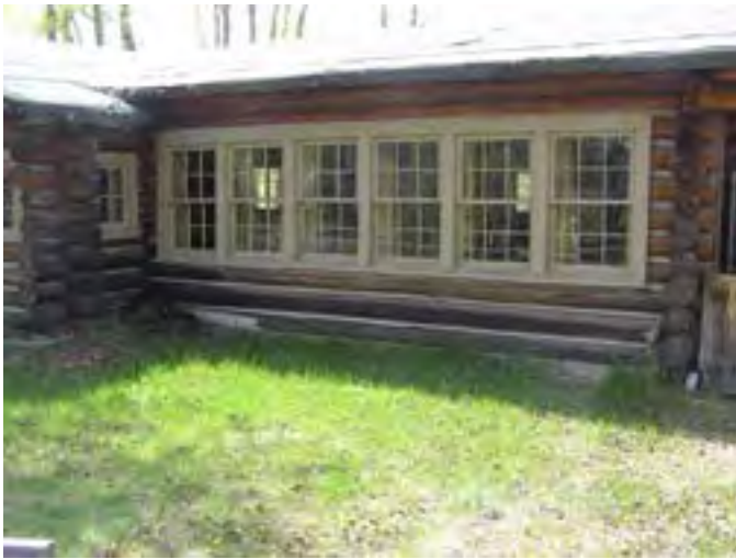
Figure 32 – Looking southwest at the dining room wall and typical wood double-hung windows. The windows are in good condition. The log walls are dry but the daubing is good.
