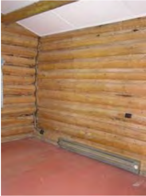
Figure 76 – Looking southwest at the log work and Celotex ceiling of the south bedroom. The interior appears dry.
