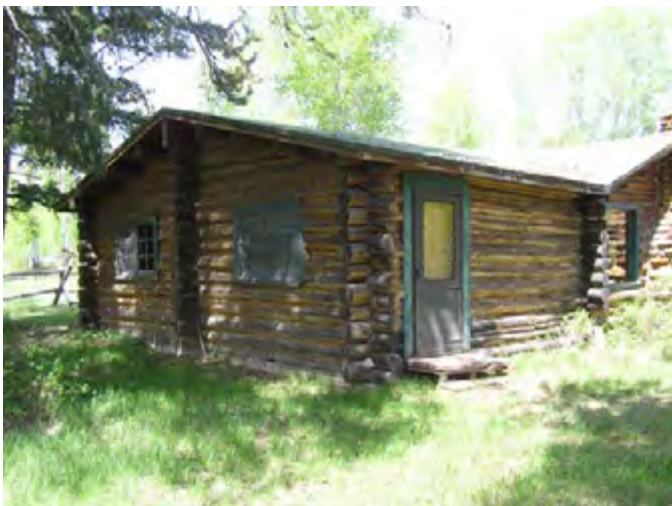
Figure 167 – Looking northwest at the south end of the Caretaker's House. Soil build-up appears to be a problem in this area causing some rot in the sill logs.
