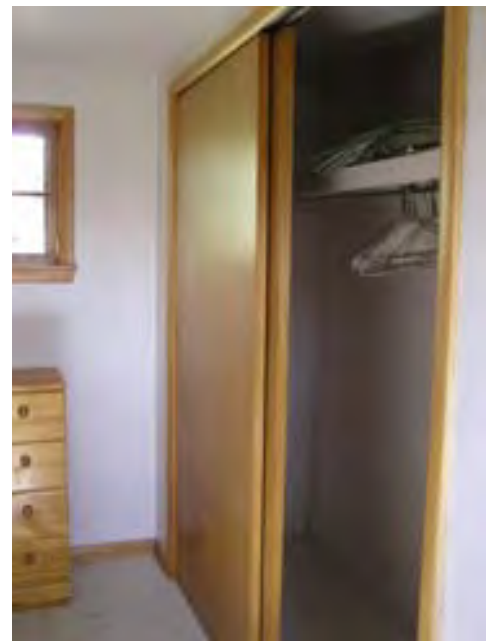
Figure 80 – Looking west at a typical closet in the connecting area of the cabin.
