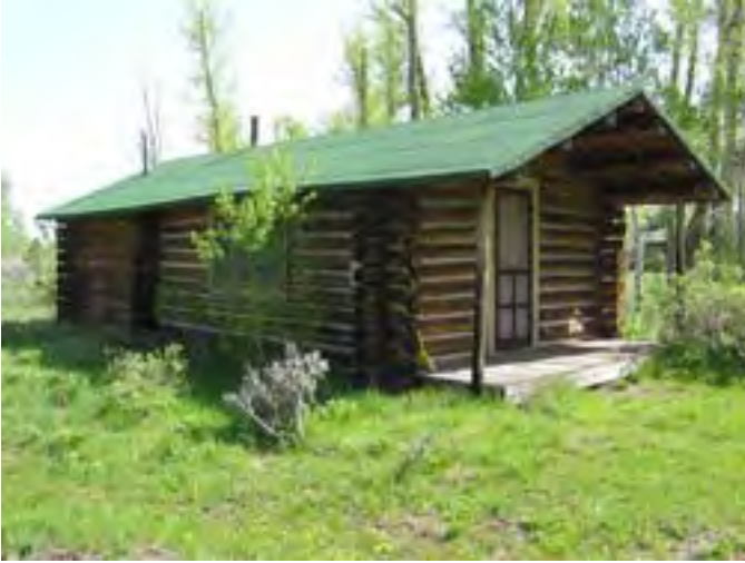
Figure 140 – Looking northeast at Harry's House. The roof is in good condition and the log walls though dry are generally in good condition. There is some rot in the sill logs.
