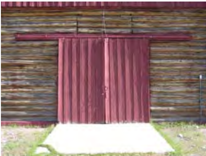
Figure 191 – Looking north at the wood sliding doors. They are warped and in fair condition.
