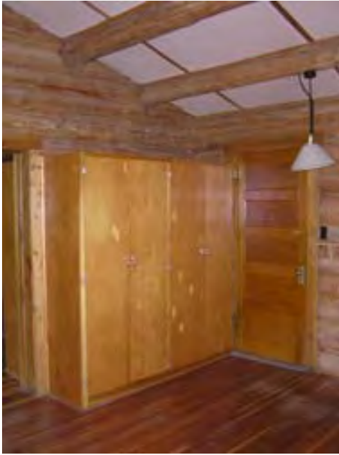
Figure 135 – Looking northwest at the wood paneled entrance door and enclosed closet area. The ceiling is Celotex set between the log purlins.
