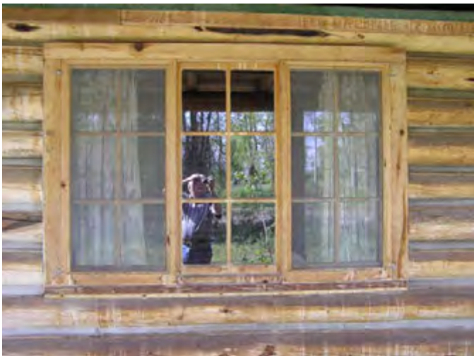
Figure 152 – Looking south at a typical wood casement window on the front of the cabin. The wood is just oiled but is dry.
