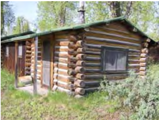
Figure 75 – Looking southwest at the log cabin on the north end of the building. It also has some sagging on the back corner because of the rotted sill logs caused by soil build-up around the base of the building.
