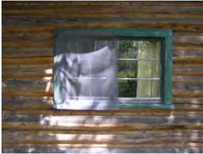
Figure 168 – Looking north at a typical wood sliding window. The window appears to be in good condition with some minor weathering on the sill.
