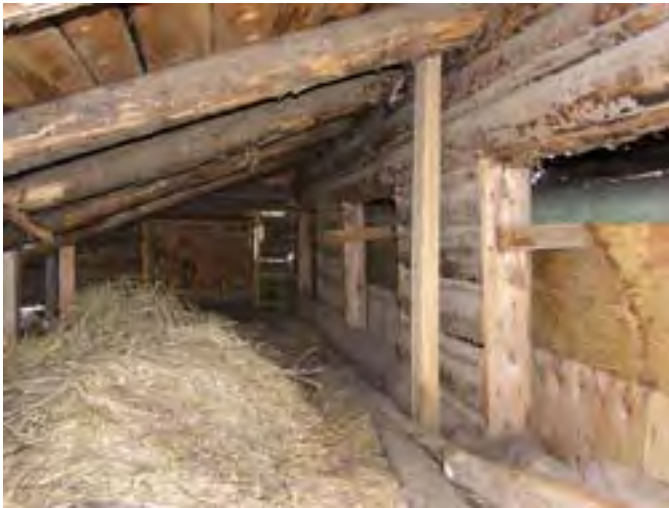
Figure 203. – Looking south at the log rafters in the east wing. There is some damaged structure on the south end allowing water to penetrate and in turn causing rot in the wood materials.
