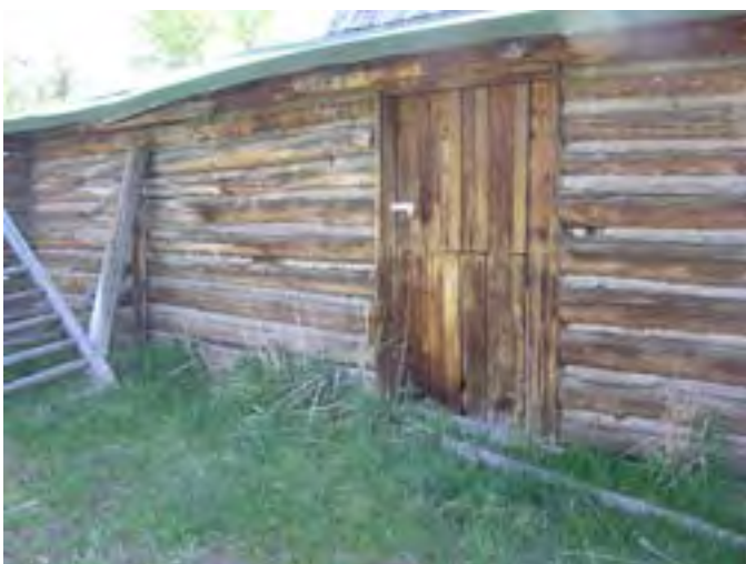
Figure 195 – Looking east at a door in the west wall. The door is in poor condition and there is rot in the sill logs because of the soil build-up around the base on this side of the building.
