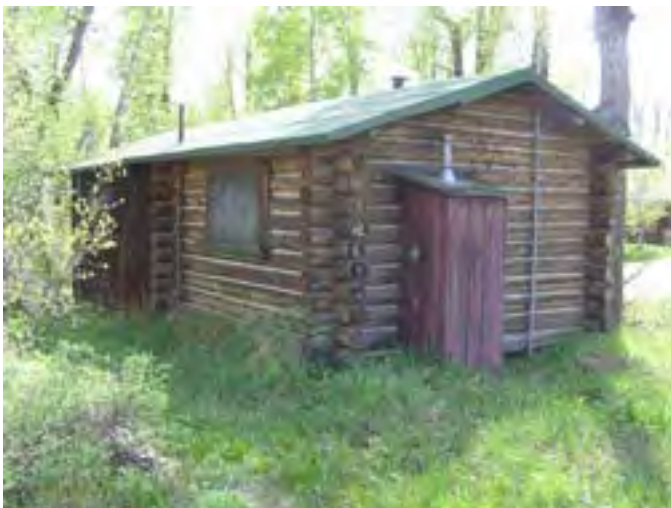
Figure 85 – Looking southwest at the log cabin portion of the building. Note the soil build-up around this end of the building which is causing the sill logs to rot.
