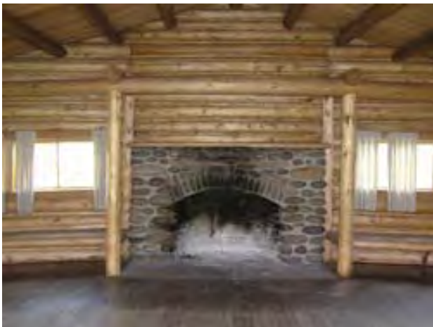
Figure 40 – Looking east at the fireplace and log work in the great room of the Lodge. Most of the woodwork and log work is in good condition. The fir floor is in good condition with the exception that there is a bulge in the center, which appears to have been caused by the outer log walls settling. This is not evident in the other rooms.
