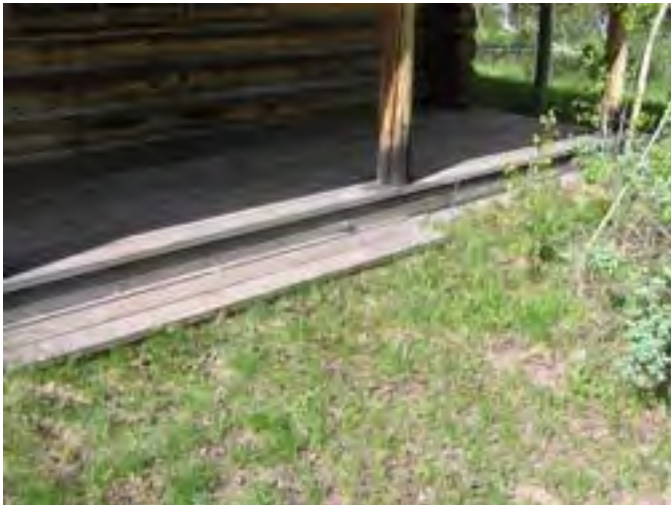
Figure 151 – Looking south at the wood porch. There is some rot in the porch and on the base of the columns.
