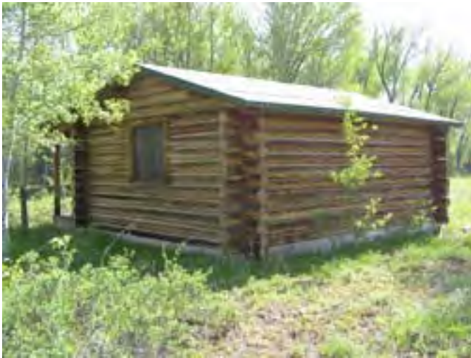
Figure 154 – Looking northeast at the cabin. The logs are dry and there is some rot in the sill log. The daubing appears to be in good condition.
