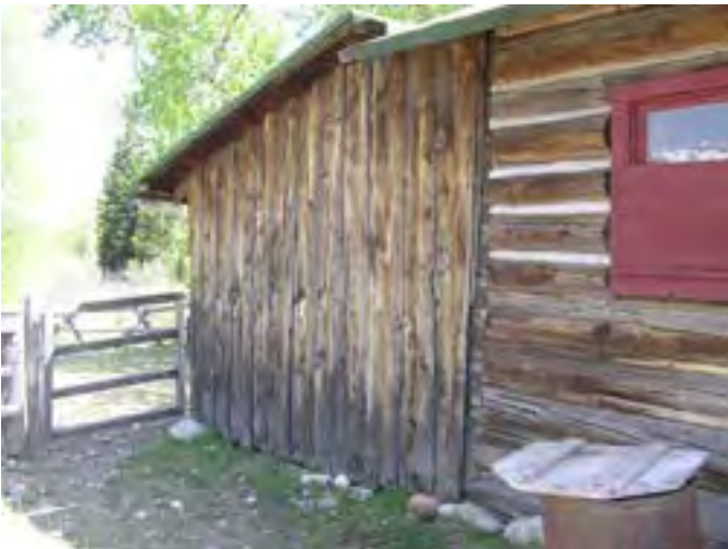
Figure 209 – Looking east at the wood frame board and batten addition on the back of the log volume. The wall is weathered and the bottom of the siding has rotted.
