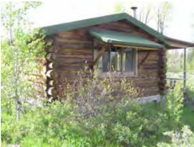
Figure 60 – Looking northwest at the cabin. Note the shed roof over the window. The window is in good condition with some minor sill rot.
