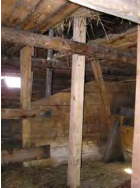
Figure 202 – Looking south at the stalls in the east wing of the Barn.
