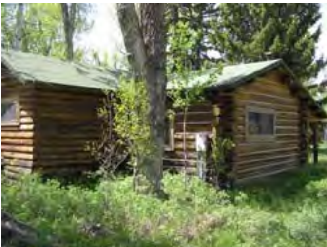
Figure 131 – Looking northwest at the cabin. The wall logs are dry and there is some rot in the sill logs due to the vegetation and soil build-up around the base. The daubing is generally good.
