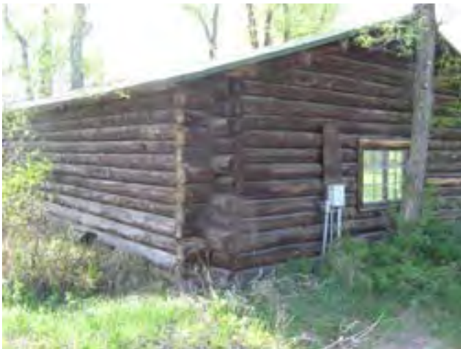
Figure 52 – Looking southeast at the garage. Note the soil accumulation around the building, which is causing some rotted sill logs.
