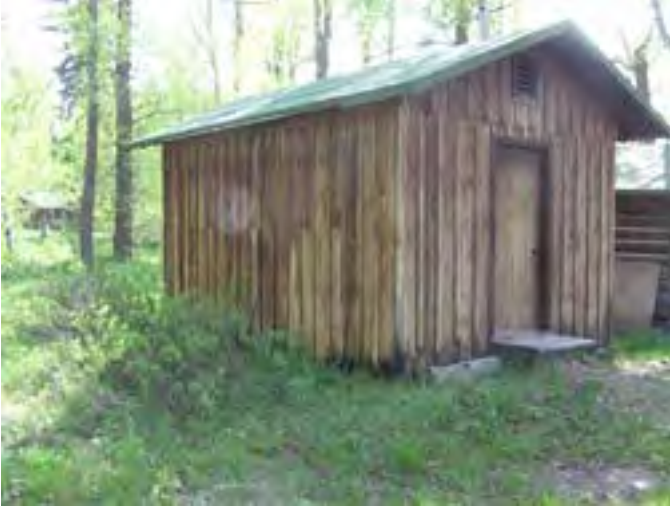
Figure 101 – Looking southwest at the board and batten Mouse House. The wood materials are very dry and there is some rot along the base of the wood siding.
