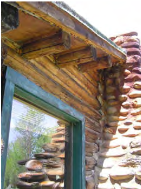
Figure 166 – Looking north up along the eave to the stone chimney. There is some staining where there have been leaks around the chimney area. There is some damage to the roofing material on the eave on this end of the building.
