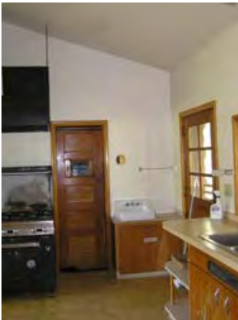
Figure 48 – Looking north at the door to pantry and the door to the right which exits to the back porch.
