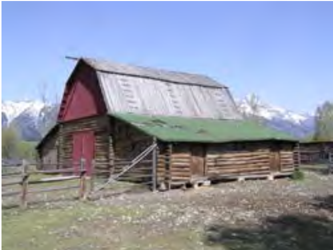
Figure 197 – Looking northwest at the Barn. The upper roof is in poor condition. The wall logs are dry.
