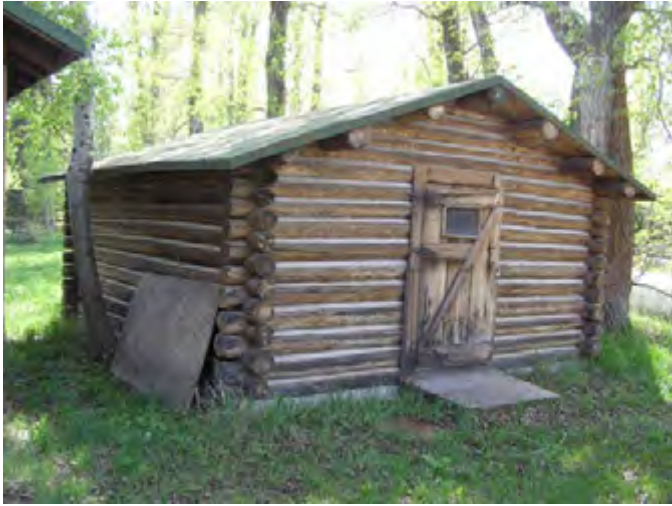
Figure 96 – Looking southwest at the log Ice House. The logs and daubing are in good condition even though the wood is dry. There is some minor surface rot at the base.
