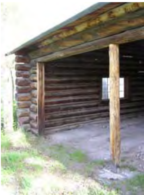
Figure 51– Looking northwest at one of the front wall columns that appears to have been replaced. The base concrete is very minimal.
