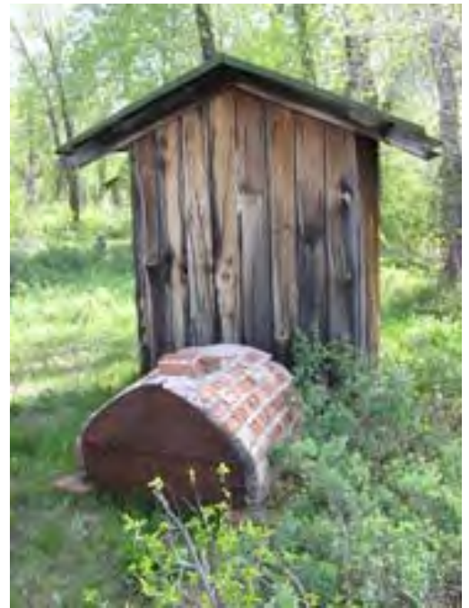
Figure 93 – Looking south at the smokehouse. The brick firebox is starting to break apart on the end closest to the building. Some mortar is missing. Note the weathered boards on the back of the building.
