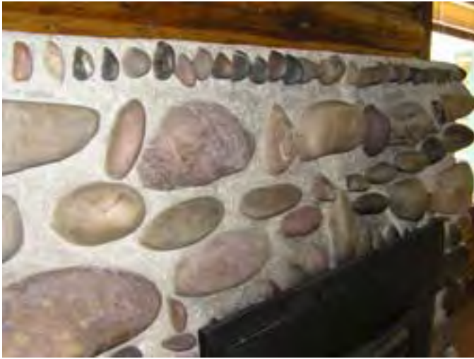
Figure 171 – Looking southeast along a detail of the fireplace. Note the river rock and patterns of the fireplace. It is in good condition.
