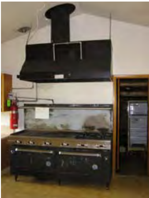
Figure 46 – Looking north at the cook stove in the kitchen. The walls and ceiling have been sheetrocked and there is a fire suppression system in the hood. There is a vinyl floor.
