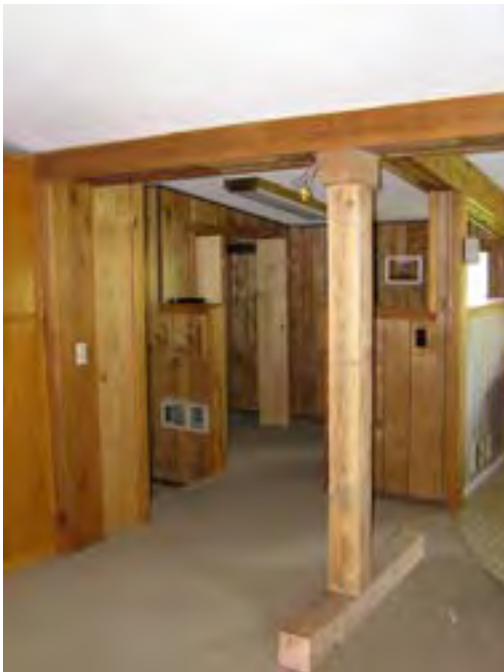
Figure 173 – Looking northeast at the kitchen area into the addition. These areas were modernized in the 1970's and are in good condition.
