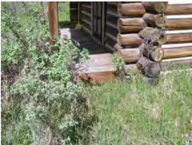
Figure 145 – Looking west at the edge of the porch which is weathered and has some rot. The columns supporting the roof rest outside the porch on concrete and stone piers.
