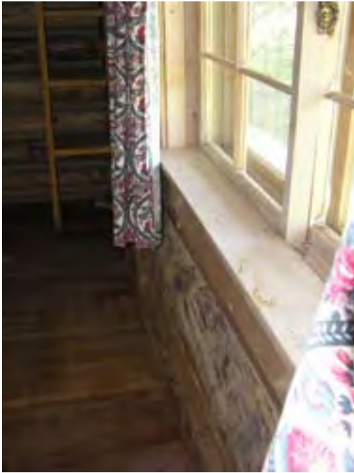
Figure 115 – Looking west along the window sill. Note the water stains on the sill and the dry wood.
