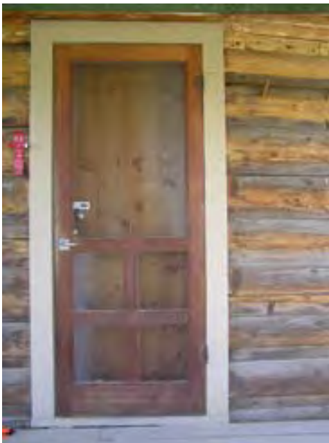
Figure 59 – Looking south at the main entrance door and screen door. They are in good condition.
