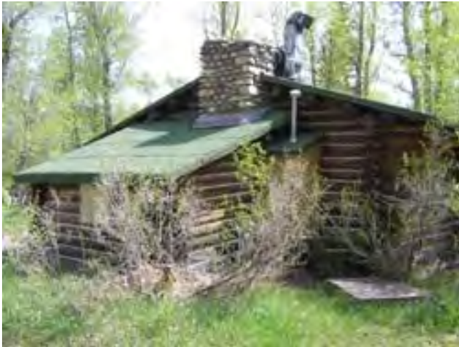
Figure 30 – Looking southeast at the Lodge with the added shed roof structure that surrounds the stone fireplace. This shed roof structure has settled because of rotted base logs and has pulled away from the Lodge wall and fireplace. Also note the water heater addition on the building which is also rotted at the base.
