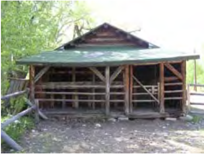
Figure 210 – Looking south at the open end of the shed-roof addition. A pole fence closes off the shed where tack was kept. There is some rot in the base of the floor and the posts of the fence. Most of the wood is very dry.
