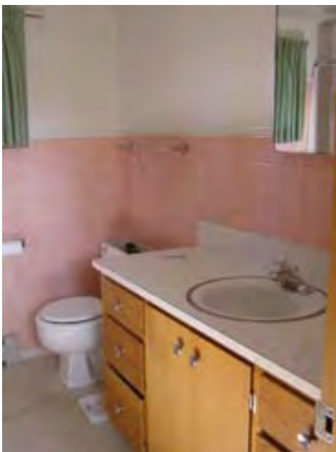
Figure 78 – Looking at the bathroom in the connection piece. The materials are in good condition.
