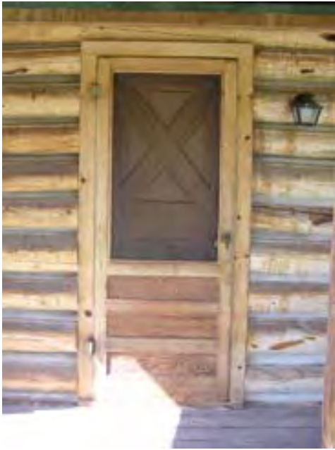
Figure 153 – Looking south at the entrance door and screen door. They are in good condition but the wood is dry.
