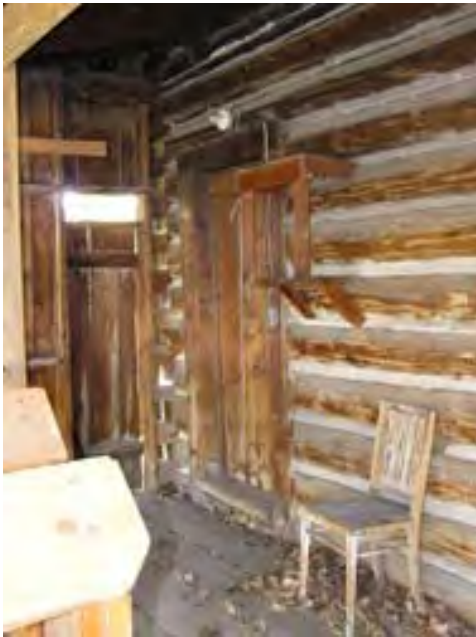
Figure 211 – Looking east along the back wall of the log Tack Room. Note the door that leads to the north room of the log volume.
