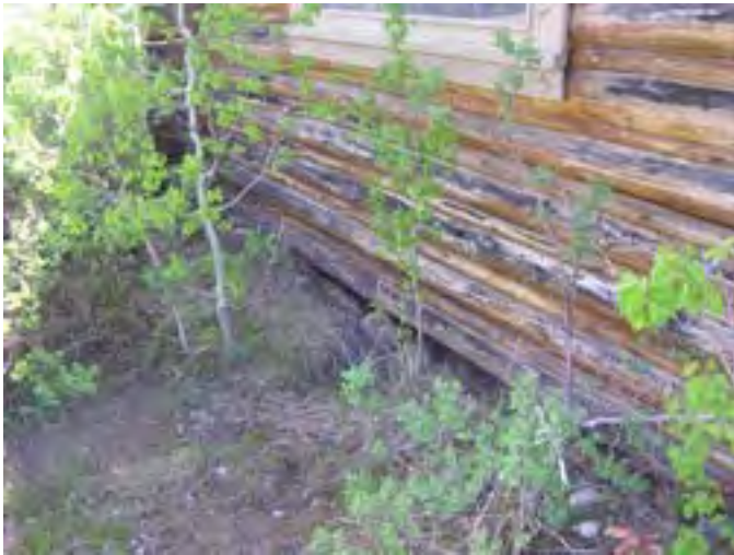
Figure 144 – Looking south at the base of the rear log wall. Note the rotted sill logs and wall logs.
