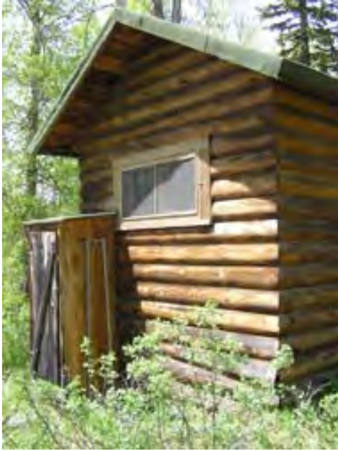
Figure 132 – Looking northwest at the back of the bathroom addition with a small structure for the water heater. The wood materials are weathered and dry and the base has some rot.
