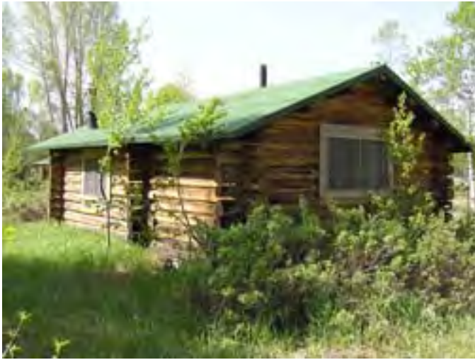
Figure 143 – Looking southwest at the cabin. Note the shrubbery and soil build-up around the building.
