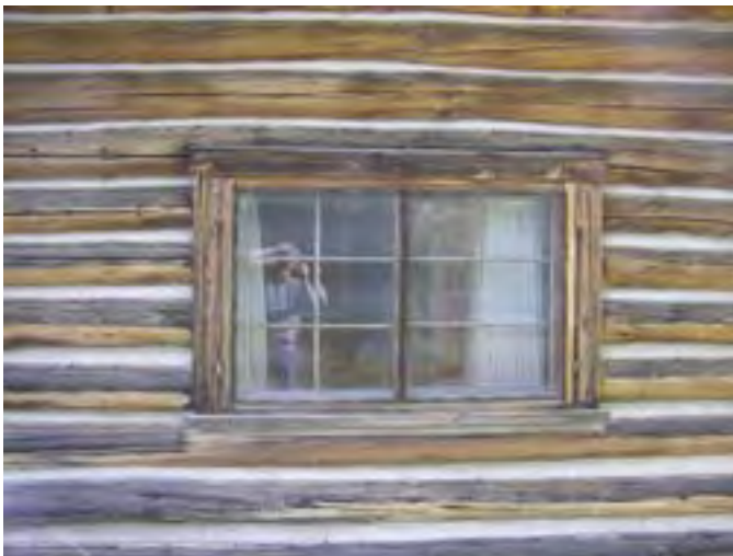
Figure 72 – Looking at a typical wood sliding window on the cabin. The glazing is poor and the wood is dry. There is some rot in the sill.
