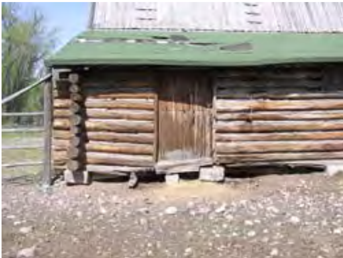
Figure 198 – Looking west at a section of the shod roof wing of the Barn. Note the damaged sheet asphalt roof where there is some damage to the structure below. Also the base logs are rotted and the logs are not properly supported at the base. The door is in poor conditional.
