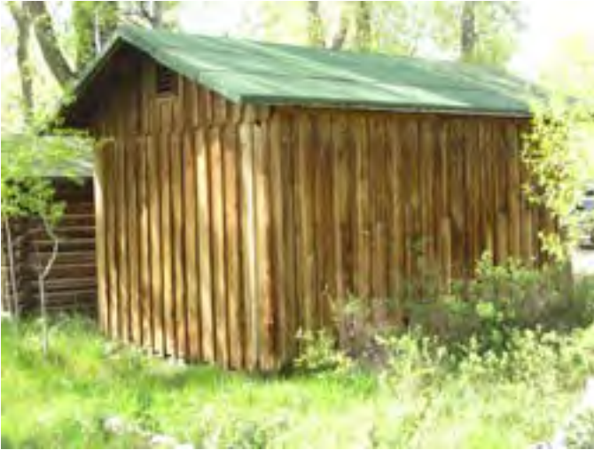
Figure 102 – Looking northwest at the building. The roof appears to be in good condition.
