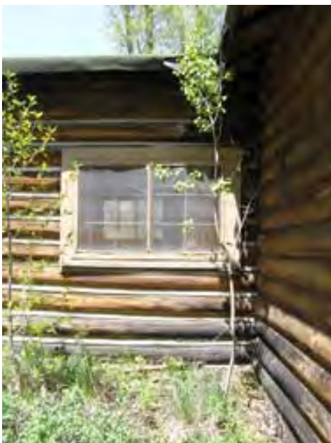
Figure 123 – Looking north at the back wall of the cabin. Note the soil build-up and the rotted and weathered sill and base logs. The window is weathered and needs repair work.
