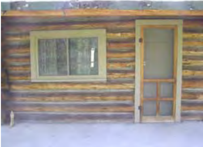
Figure 119 – Looking south at a typical wood sliding window and wood paneled door into each of the units. They are in good condition with the exception of the screen doors, which are dry and stained.
