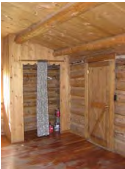
Figure 63 – Looking northwest at the front door and closet. The materials are in good condition.
