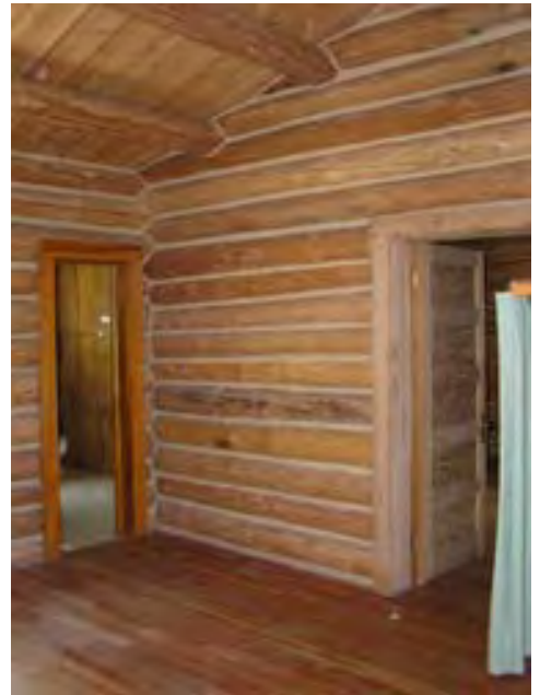
Figure 113 – Looking southwest at the interior of the east bedroom towards the bathroom and the connecting door to the west bedroom. The fir floor has some minor wear areas. The wall and ceiling materials are in good condition.
