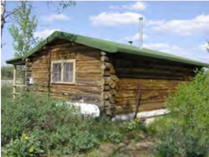
Figure 61– Looking northeast at the cabin. Note some surface rot in the sill logs.
