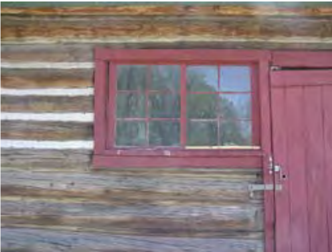
Figure 208 – Looking east at the door and window on the west side of the building. They are in good condition with some weathering of the window sill and base of the door.
