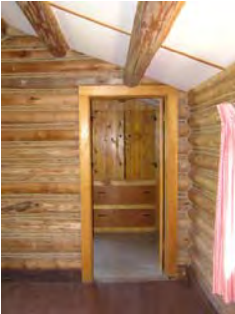
Figure 147 – Looking north from the bedroom to the doorway into the bathroom addition. The materials appear to be in good condition.
