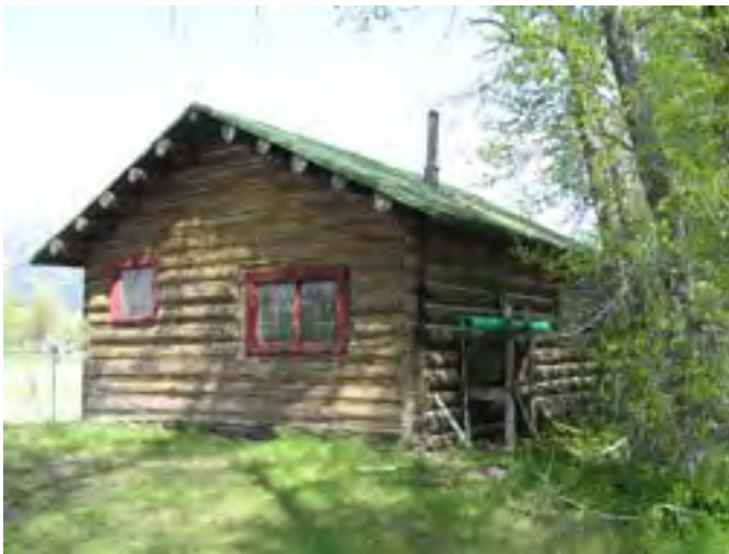
Figure 214 – Looking northwest at the Tack Room. Note the soil accumulation around the south and east sides of the building. The sill logs and some wall logs are rotted in this area.
