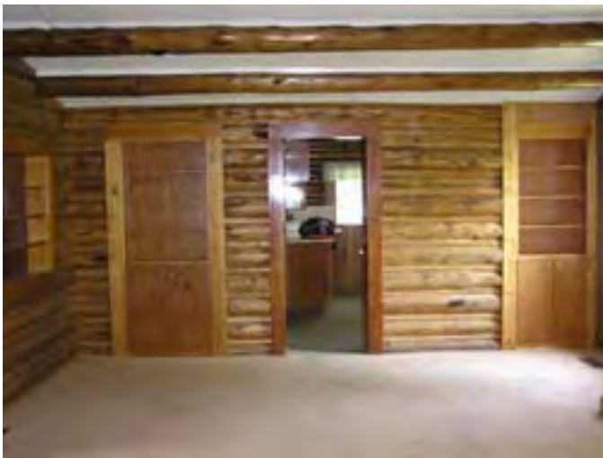
Figure 172 – Looking north at the wall of the great room and the entrance to the kitchen. Note the infilled doors with bookcases. The walls are in good condition.
