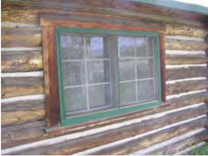
Figure 86 – Looking west at a typical window in the log cabin. Note the dry logs and dry wood around the window. The daubing is generally in good condition with some minor missing daubing.
