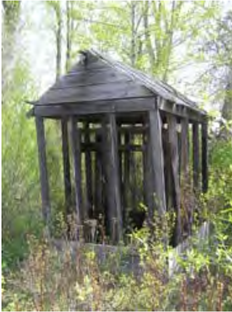
Figure 68 – Looking south at the Curing House. The screen is damaged and most of the wood is rotted. There is no roof covering on the building.
