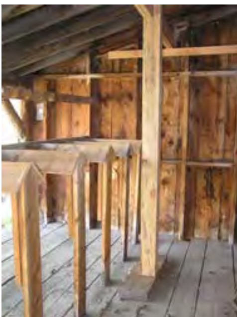
Figure 212 – Looking east at the tack area in the shed. Most of these materials are weathered but in good condition.
