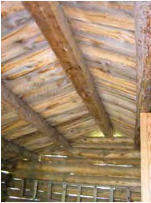
Figure 187 – Looking south at the board ceiling spanning the purlins. Note some dry rot in the wood.
