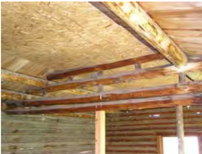
Figure 56 – Looking east at the roof structure and the supports in the middle section of the roof. Note the sag in the roof logs.
