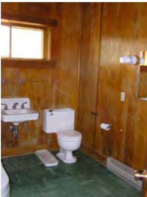
Figure 137 – Looking southwest at the bathroom. There is electric baseboard heat throughout the cabin.
