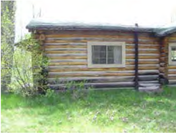
Figure 35 – Looking west at the bedroom wall. Note the rot in the lower base logs and soil around the base of the building in this area.
