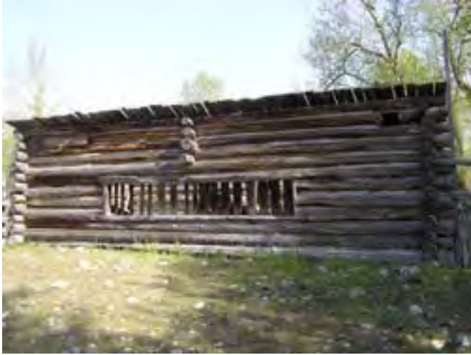
Figure 219 – Looking north at the front façade of the Chicken Coop. This log wall is in good condition although it is weathered and dry.
