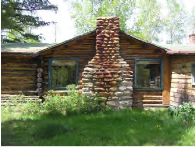
Figure 165 – Looking west at the stone chimney and log walls. The windows are in good condition with some minor weathering on the sills. A couple of the log ends of the inner walls have rotted and broken off.
