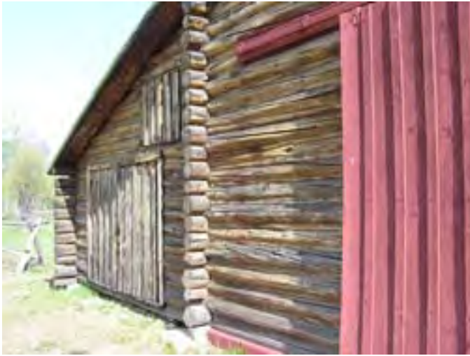
Figure 193 – Looking northwest along the front of the building showing the log work. The center section has a concrete foundation that helps to support the front wall and is in good condition. The shed roof structure has some settlement under the doors that are in poor condition.
