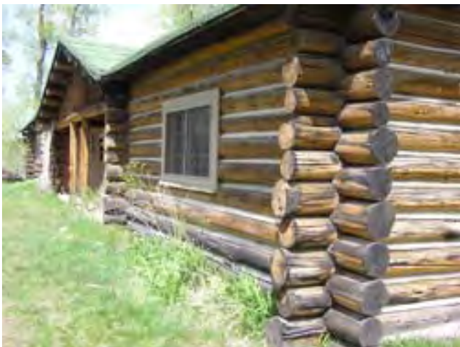
Figure 37 – Looking northeast at the Lodge building. Note the soil accumulation which has contributed to the rotted sill logs and base log at the corner.
