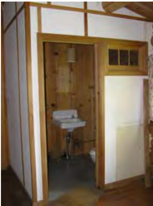
Figure 42 – Looking north at the added bathroom in the east bedroom of the Lodge. The materials are in good condition.
