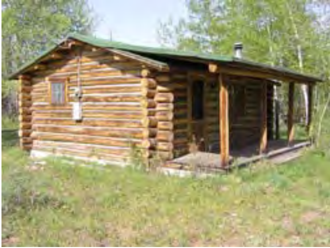
Figure 150 – Looking southwest at the cabin and front porch. The cabin sits up on a concrete foundation and generally the grade is good around the building. The roof is in good condition.
