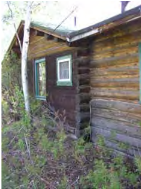
Figure 169 – Looking north along the log wall to wood frame infill in the original porch. The wood siding is weathered and logs have some surface rot.
