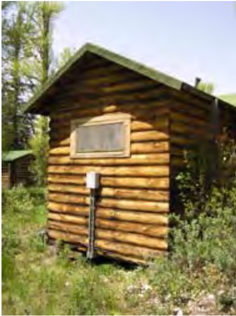
Figure 122 – Looking north at the back wall of the addition. The wood is dry and weathered, and the window needs some glazing work.
