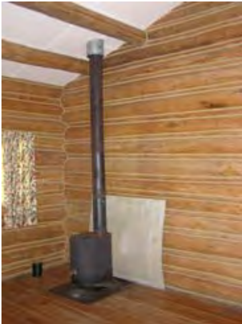
Figure 125 – Looking northeast at the interior of the east bedroom. Note the wood stove and log walls. The free-standing heat shield behind the stove may contain asbestos. The ceiling has a Celotex infill between the log purlins. The wall and ceiling materials are in good condition and the fir floor has some minor wear but is in good condition. Possible asbestos heat shield behind wood stove.
