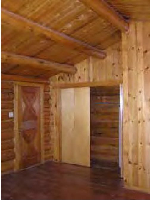
Figure 156 – Looking northeast at the wood entrance door and closet. The fir floor has some minor wear but all in all the materials are in good condition.
