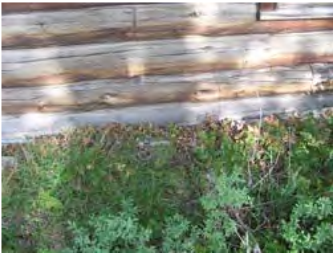
Figure 54 - Looking west at the base of the east wall. Note the soil accumulation and the rot in the sill log. The daubing is poor.
