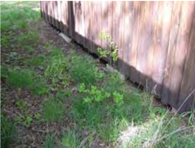
Figure 103 – Looking northeast at the base of the building. Note the concrete piers along the wall, which is in good condition.
