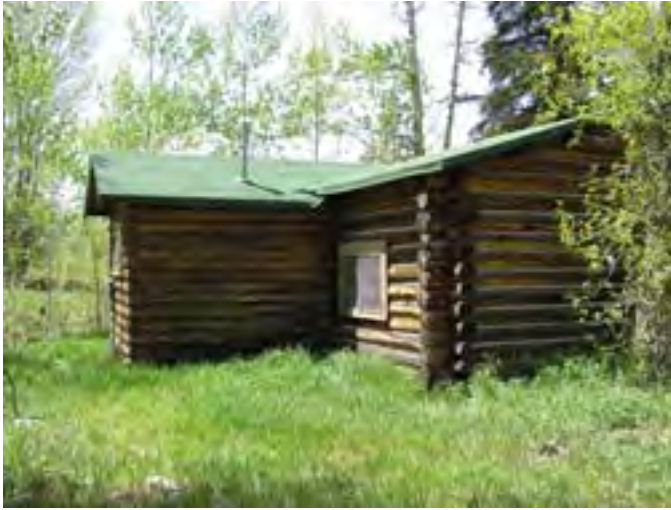
Figure 109 – Looking west at the back of the building with the bathroom addition. Most of the logs and the roof are in good condition. The sill logs and some of the wall logs are weathered and rotted.
