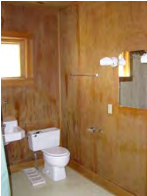
Figure 116 – Looking south at the bathroom addition to the cabin. The fixtures and materials are in good condition.
