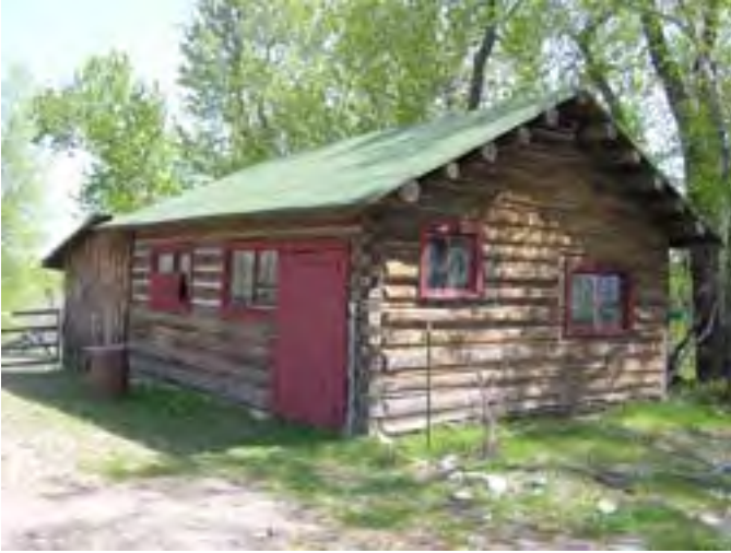
Figure 207 – Looking northeast at the Tack Room. The wall logs are in good condition with the exception of some rotted sill logs on the east side. The roof is in good condition.
