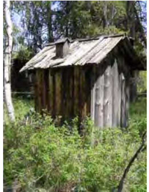
Figure 180 – Looking northeast at the outhouse. Note the accumulated soil and vegetation around the back of the building.
