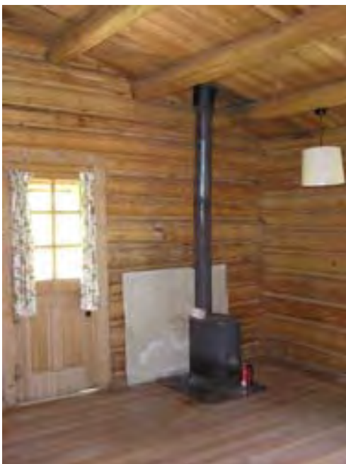
Figure 43 – Looking southwest at the west bedroom and its wood stove and chimney. The materials are in good condition.
