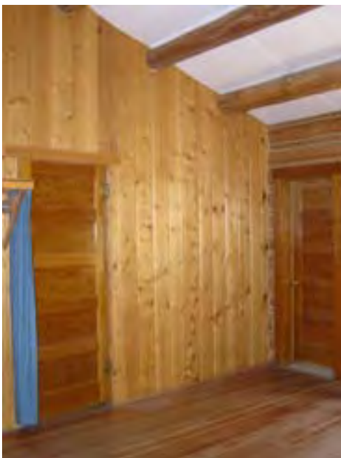
Figure 126 – Looking southeast at the interior of the west bedroom. Note the wood paneled doors to the other bedroom and bathroom. The materials are in good condition.
