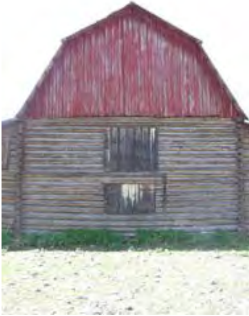
Figure 196 – Looking south at the gambrel end of the roof and log structure below. The boards and battens are warped and weathered. The doors in the lower section are in poor condition.
