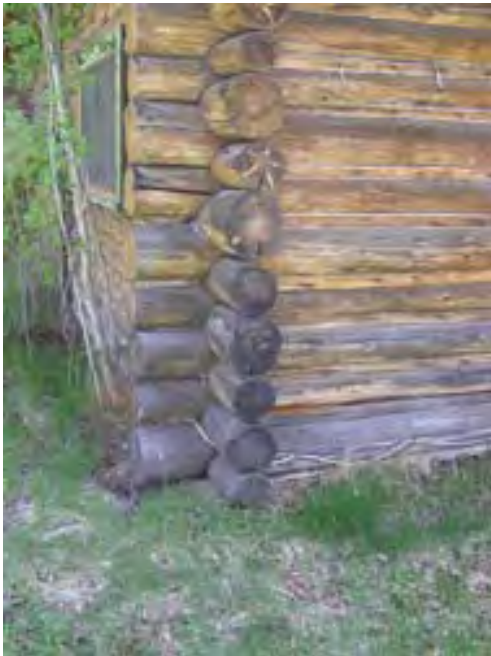
Figure 163 – Looking southeast at the log corner notches. Note the rotted sill log and surface rot on the upper logs due to the soil build-up around the base.
