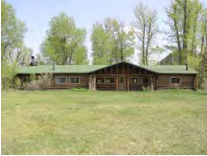
Figure 23. Looking east at the façade of the Lodge. The building is generally in good condition.
