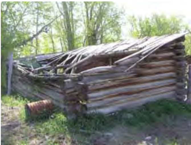
Figure 220 – Looking east at the end of the Chicken Coop. Note the collapsed roof causing the walls to fail also.
