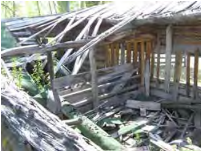
Figure 221 – Looking east at the interior of the collapsed building.
