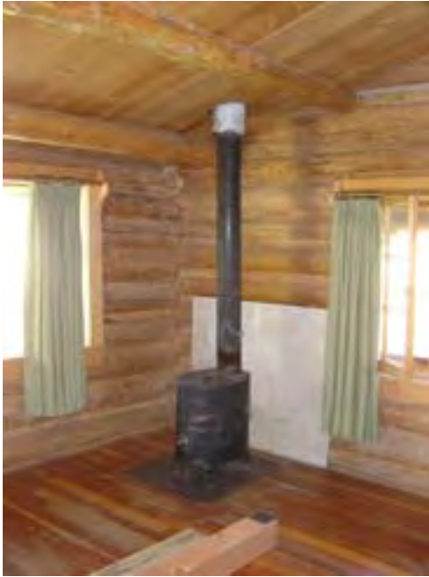
Figure 64 – Looking northeast at the wood stove and window area (possible asbestos heat shield behind wood stove).
