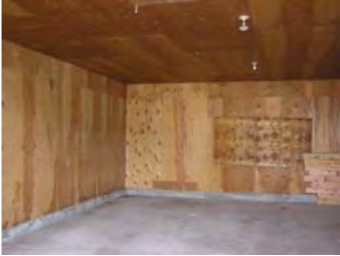
Figure 199 – Looking north at the room within the gambrel center section of the Barn. There is a new concrete floor, framed walls and plywood paneling. There is a roof with sheet asphalt on top in the loft area.
