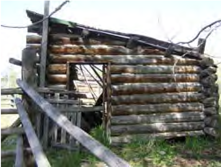
Figure 222 – Looking west at the wall of the Chicken Coop. There appears to be rot in all of the sill logs and upper parts of the walls which did support the roof.
