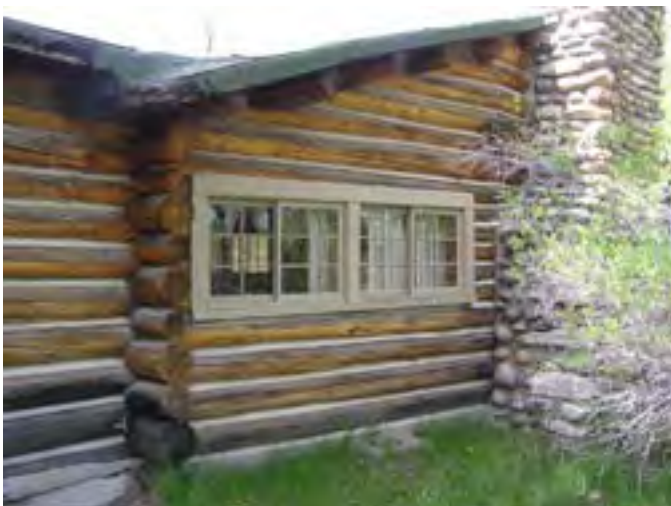
Figure 34 – Looking west at the log wall of the great room with the stone chimney. There are some rotted base logs especially at the intersection of the bedroom and the great room. The roof is damaged in this area and there is some separation of the logs and stone chimney.
