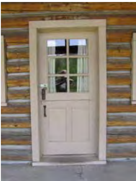
Figure 25. Looking east at the main entrance door which is in good condition.
