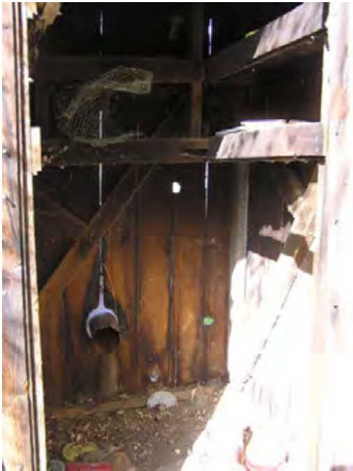
Figure 94 – Looking north at the interior of the smokehouse. The wood interior is also deteriorating.
