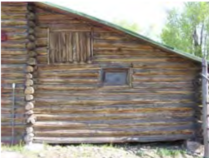
Figure 192 – Looking north at the east shed roof structure. The sill logs span the gap between the concrete piers that are showing some deterioration.
