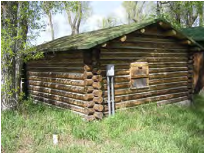
Figure 97 – Looking northeast at the Ice House. The roof is in good condition with some minor damage on the west side. The building sits up on a concrete slab and the grade around the building is good except for the southwest corner. There is some rot in the sill logs.
