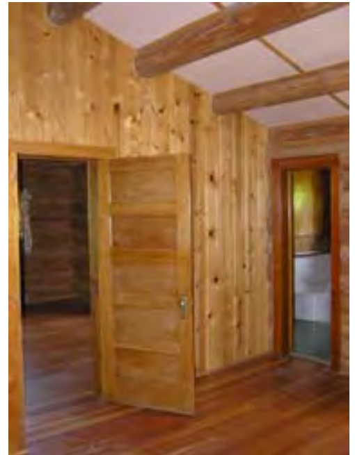
Figure 136 – Looking southeast at the connecting door and opening to the bathroom from the west bedroom. Note the good condition of the materials.
