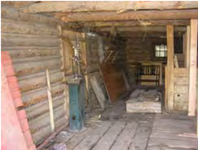
Figure 200 – Looking north at the interior of the west wing. There is some rot in the floor and the structure for the roof needs to have additional supports to take care of the snow loads on the building.
