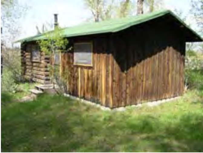
Figure 83 – Looking northeast at the cabin and at the frame addition to the log cabin on the south side. Note the dry wood on the addition. The roof appears to be in good condition.
