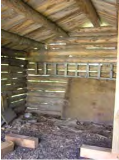
Figure 186 – Looking south at the interior of the Garage. Note the open areas between the logs and the log purlins. Water stains on the board sheathing indicate that the roof leaks.
