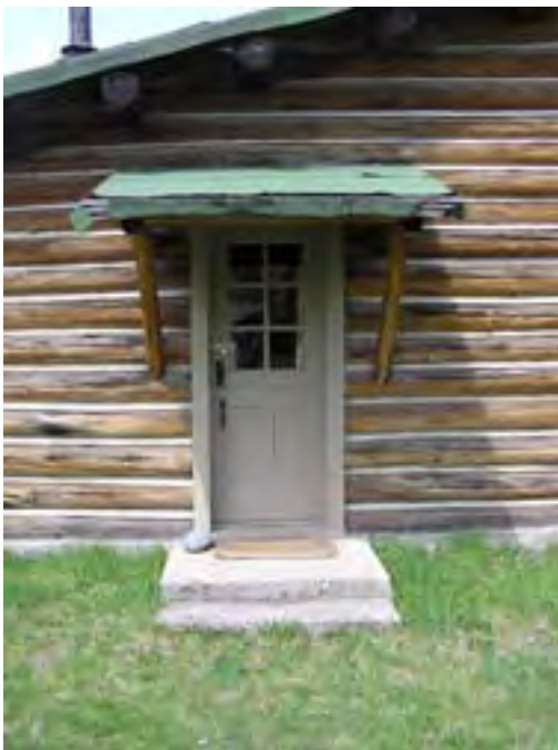
Figure 36 – Looking north at one of the typical shed roofs over the exterior doors in the bedrooms. Note the damaged sheet asphalt roof.
