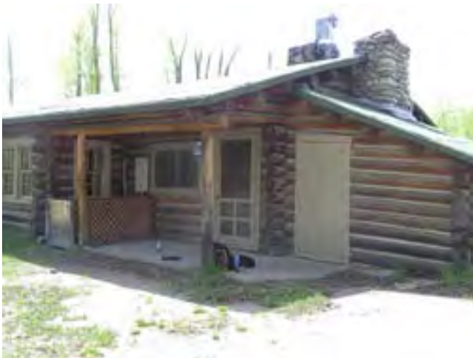
Figure 31 – Looking southwest at the back porch area. The stone chimney over the shed roof addition has some missing mortar and the flashing around the chimney is poor. The sheet asphalt roof has some damage.
