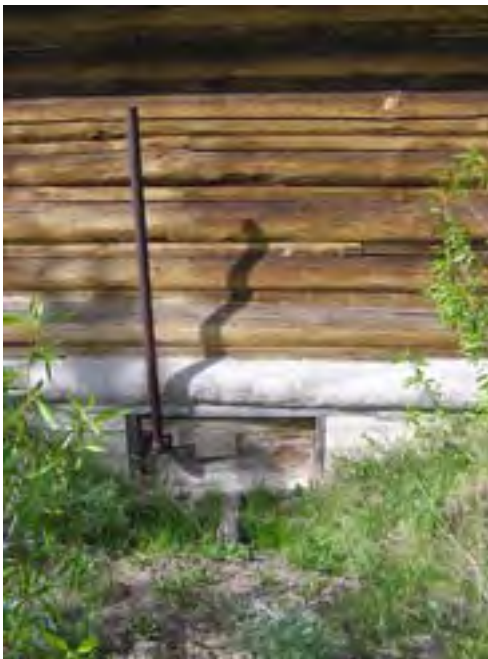
Figure 62 – Looking north at a base detail of the cabin. It appears that the sill log has been replaced with a concrete surface that is rounded like a log. Note the vent area to the crawl space.
