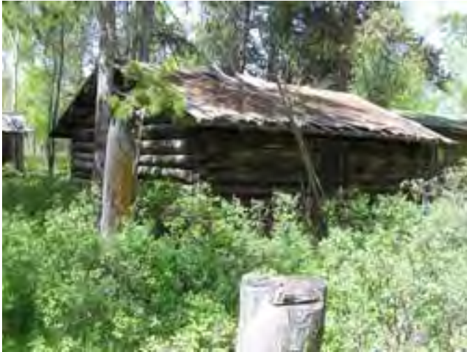
Figure 184 – Looking northwest at the Garage. The vegetation and soil build-up around the building has caused the sill logs to rot.
