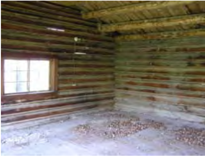
Figure 55 – Looking northwest at the interior. The logs are missing some daubing and the thin concrete floor is broken up.
