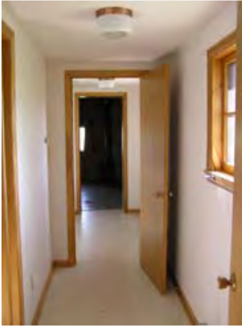
Figure 79 – Looking north at the hallway connecting the two log volumes. The sheetrock walls and ceiling and vinyl floor are in good condition.
