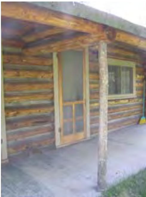
Figure 130 – Looking southwest at the front porch and typical door and window. The screen door wood is dry and stained. Note the concrete slab and wood infill where some piping evidently comes into the cabin.
