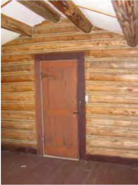
Figure 146 – Looking south at the bedroom and the main entrance door. Note the fir floor, log walls, and Celotex ceiling. These materials are in good condition with some staining around the vent pipe in the bathroom.
