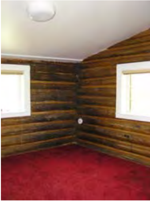
Figure 174 – Looking northwest at the bedroom in the northwest corner of the house. The walls and windows are in good condition. The sheet rocked ceiling is also in good condition.
