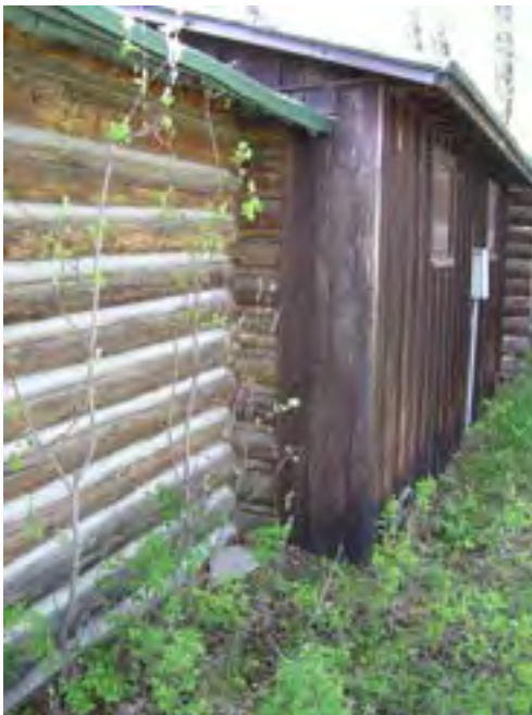
Figure 74– Looking south at the connection between the log cabin and the wood frame connecting rooms. Note the different roof planes and the water penetration into the corner.
