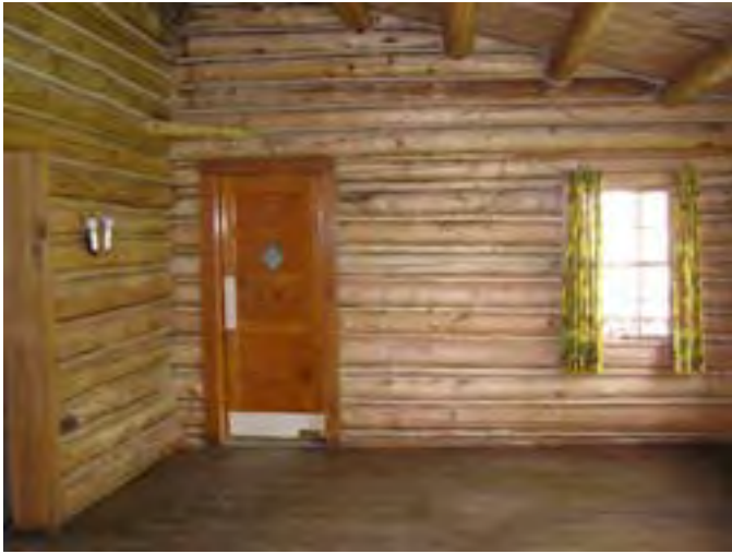
Figure 44– Looking north from the dining room towards the door to the kitchen. The materials are in good condition.
