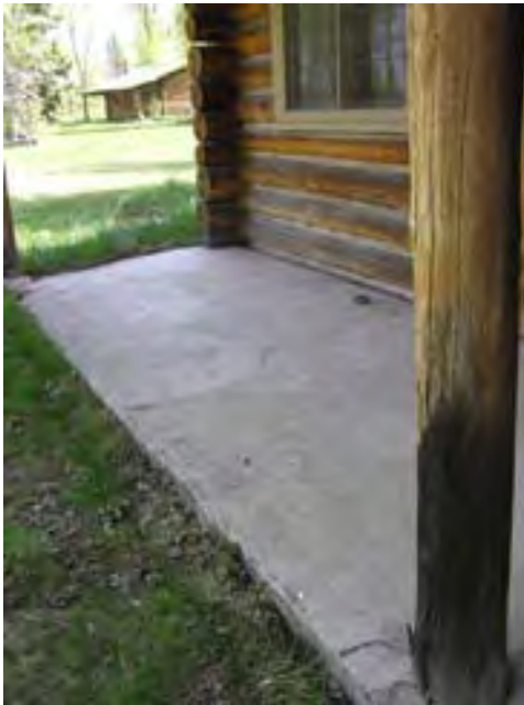
Figure 107 – Looking east at the concrete porch. There is some cracking around the column bases. Also there is a gap between the slab and the base log. Also note the surface rot on the bases of the columns.
