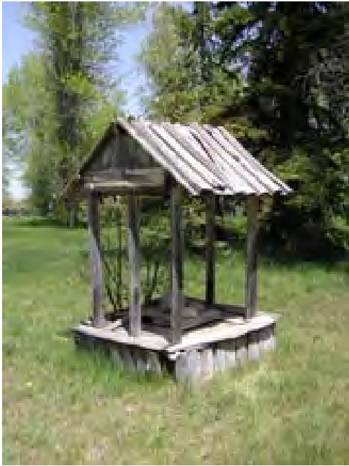
Figure 159 – Looking southeast at the well housing. The structure is weathered and there is rot along the base. The board and batten roof is in poor condition.
