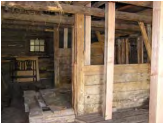
Figure 201 – Looking north at some of the original stalls for horses and dairy cows in the west wing.
