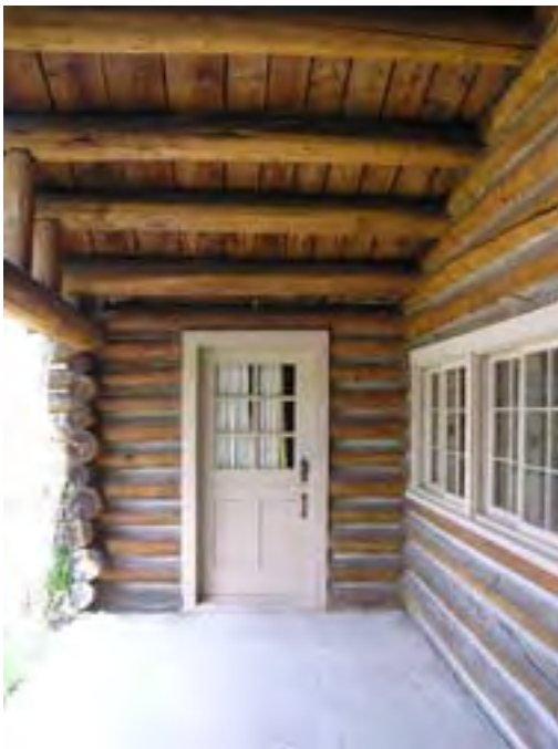
Figure 27. Looking north at a door into the living room from the front porch. Note the roof structure is in good condition.
