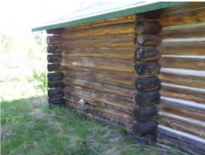
Figure 142 – Looking northeast along the Main Cabin and log addition to the north. The logs are dry but there is some rot in the sill logs because of the soil build-up. The daubing in the original building is good and wood chinking in the addition appears to be good.
