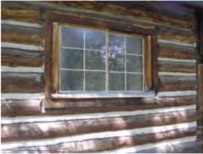
Figure 213 – Looking west at a typical wood sliding window on the Tack Room. The window is in poor condition. The log walls are dry but the daubing appears to be generally in good condition.
