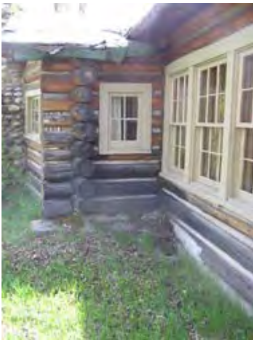
Figure 33 – Looking south at the intersection of the dining room and great room walls. Note the soil that has accumulated on this side of the building and the rotted base logs. Also, note the damaged sheet asphalt roof.
