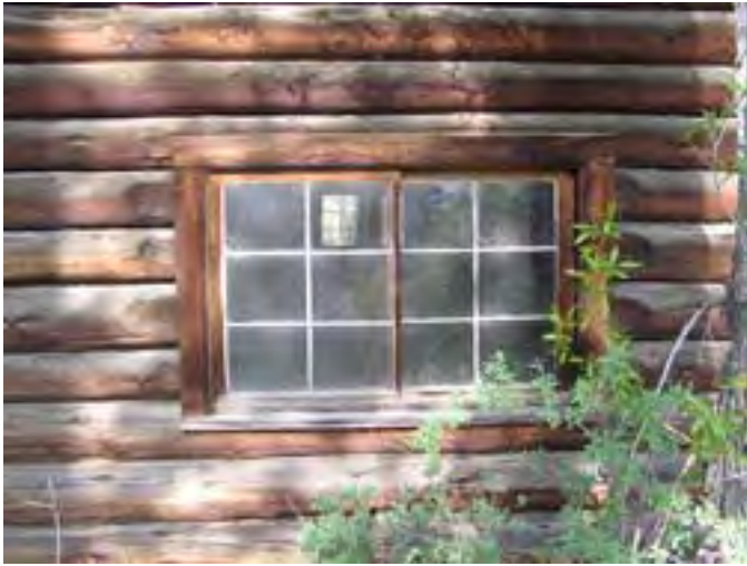
Figure 53 – Looking west at the wood window sash on the east side of the garage. The glazing is deteriorated and the wood is dry. The sill has some rot.
