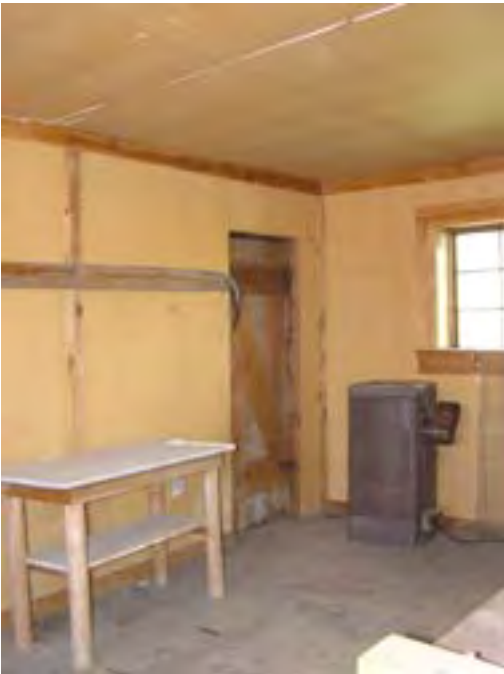
Figure 217 – Looking east at the north room in the log volume. Note the Celotex walls and ceiling.
