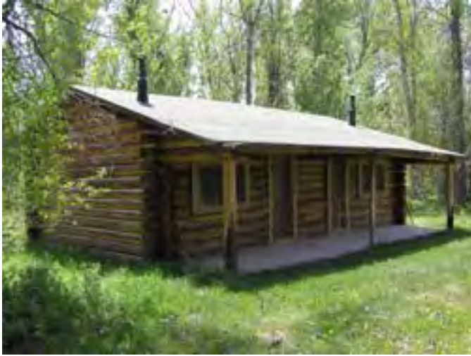
Figure 118– Looking southwest at the cabin and front porch. The roof is in good condition with some minor damage on the eave of the porch roof.
