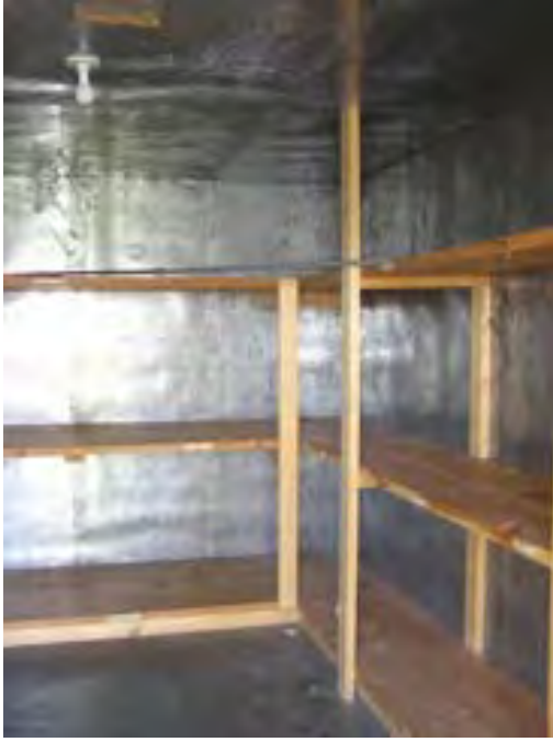
Figure 104 – Looking south at the interior of the building which has been lined with galvanized metal to keep out the mice. The materials are in good condition.
