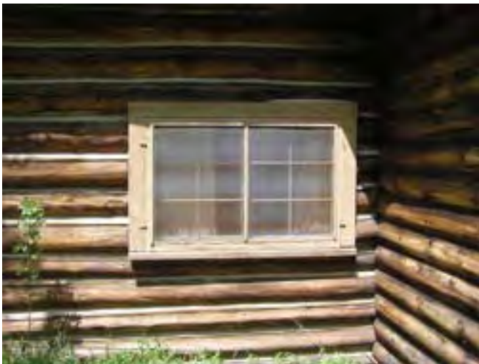
Figure 111 – Looking north at a typical wood sliding window with screen. Note the dry and weathered wood on the sill of the window. The paint is also peeling in some areas.
