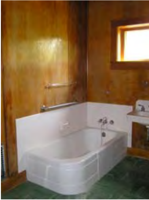
Figure 138 – Looking southeast at the bathtub in the bathroom. This area is dry and there does not appear to be any mould. The vinyl tile floor is in good condition.
