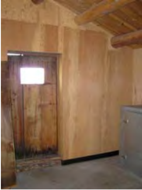
Figure 99 – Looking north at the interior and entrance door. The materials are in good condition but there is some rot on the base of the door from exterior water.
