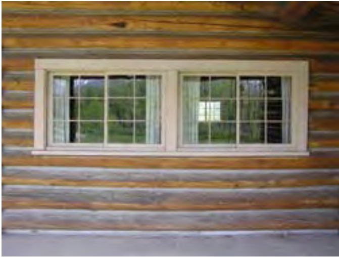
Figure 26. Looking east at a typical set of wood sliding windows in the entrance porch area.
