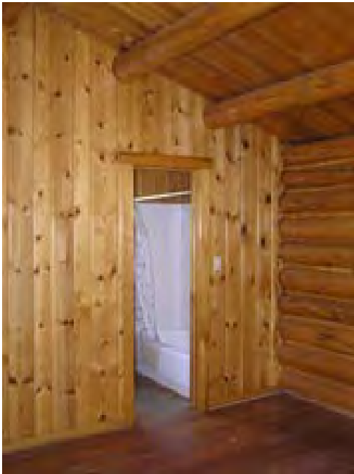
Figure 157 – Looking southeast at the bathroom and the integral fiberglass tub/shower beyond. These areas are also in good condition.
