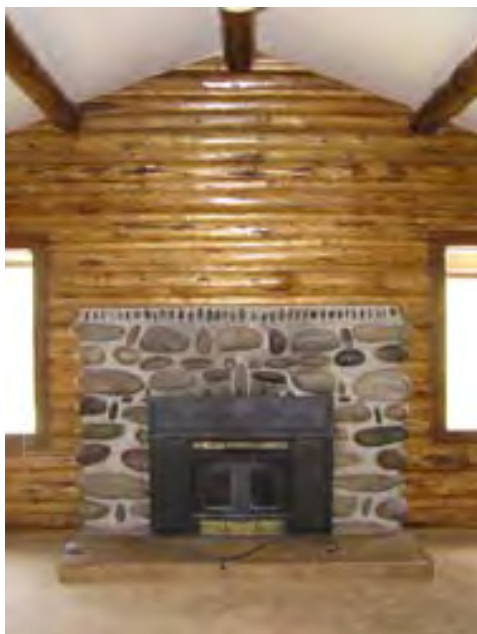
Figure 170 – Looking east at the fireplace and log wall of the great room. The log walls, celotex ceiling and log structure appear to be in good condition. The floors are covered with carpet.
