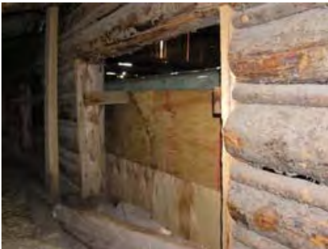
Figure 204. – Looking west at the frame structure that was built in the center section of the Barn. Note the sheet asphalt roof over the structure.
