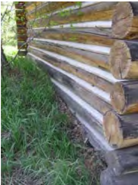
Figure 108 – Looking south along the east side of the cabin. The logs and daubing are in good condition but the wood is dry and there is some rot in the sill logs. Note the grade buildup against the logs.
