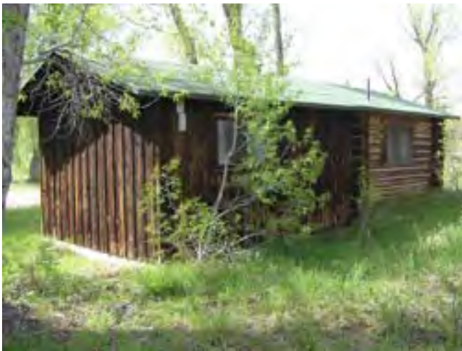
Figure 87 – Looking northwest at the frame addition to the building. Most of the addition sits up on the concrete foundation but the grade is poor on the east side.
