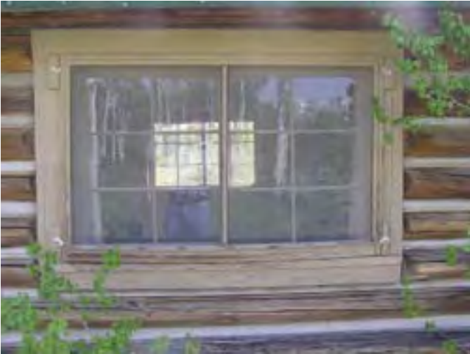
Figure 141 – Looking east at a typical wood sliding window and screen. Note the peeling paint and weathered wood on the sill of the window.
