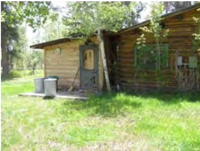
Figure 164 – Looking south at the house and kitchen wing addition. There is some rot in the sill logs and the base of the addition. The wood including the logs and wood chinking is dry but in good condition.
