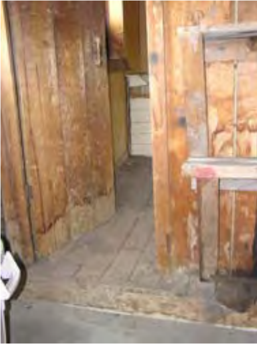
Figure 216 – Looking north at the doorway to the north room in the log volume. Note the transition from concrete floors to a wood floor. There are water stains on the base of all of the woodwork.
