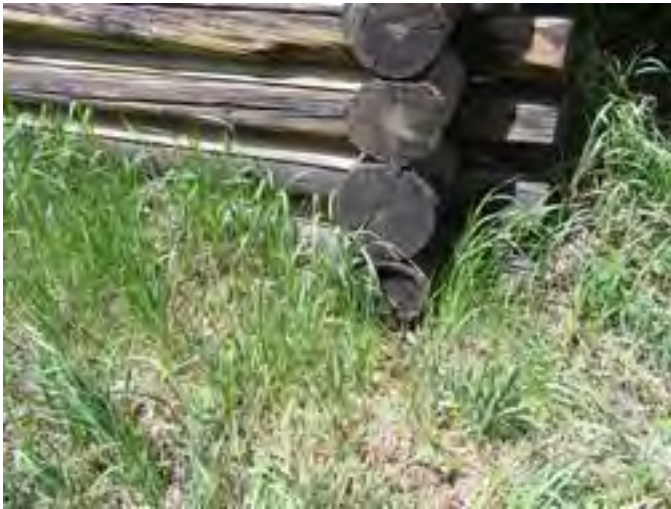
Figure 110 – Looking north at a corner of the back wall of the cabin. Note the soil built up around the sill logs and weathered and rotted wall logs.
