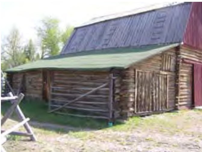
Figure 194 – Looking northeast at the Barn. There is some settlement in the log walls which show up in the eave of the roof. The sheet asphalt is in good condition but the board and batten roof of the central section is in poor condition.
