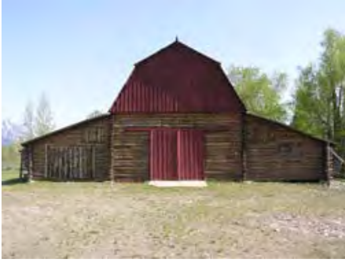
Figure 190 – Looking north at the front façade of the Barn. The log base and board and batten upper portion of the gambrel roof end are generally in good condition. There is some warping of the boards.
