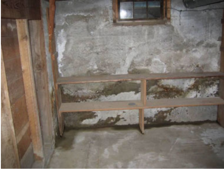
Figure 28 Evidence of damp
