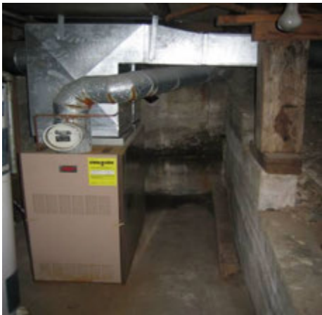
Figure 52 Oil burning furnace
