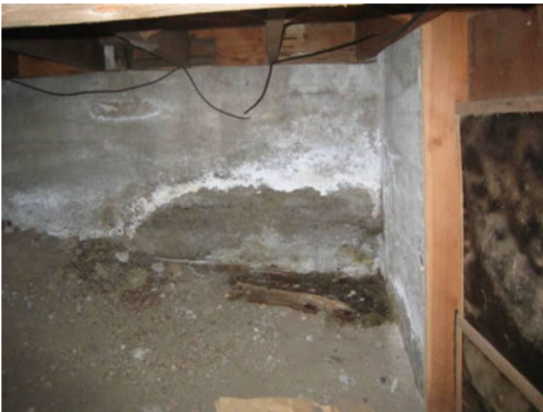
Figure 29 Evidence of Efflorescence
