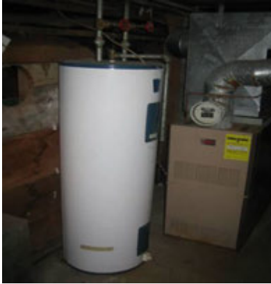
Figure 55 Electric water heater
