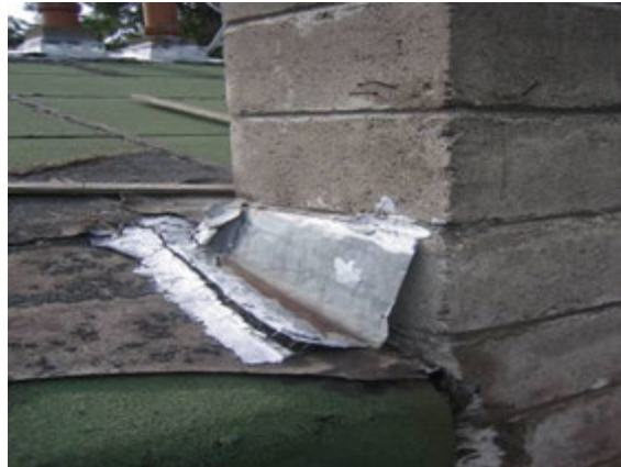
Flashing deteriorating at cinder block flue
