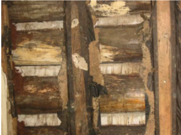
Figure 34 Bedroom #3 west wall – resistance drilling sample locations #2-6
