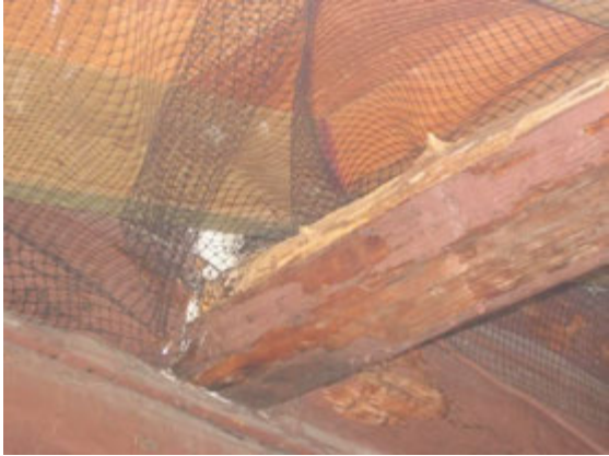
Figure 38 Bedroom #2 purlin rot at bearing point
