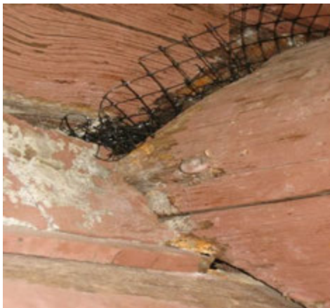
Figure 35 Bedroom 3 saddle notch rot – Resistance drilling #15
