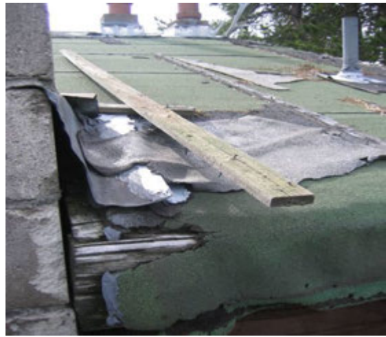
Flashing deteriorating at cinder block
