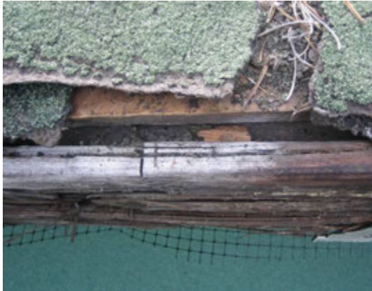
Figure 43 Fascia rotting and roofing not covering
