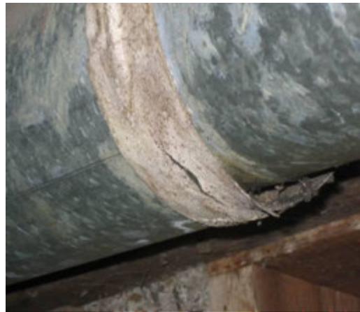
HVAC duct joint
