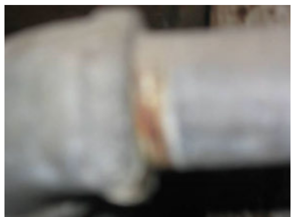
Rust at galvanized water pipe joint
