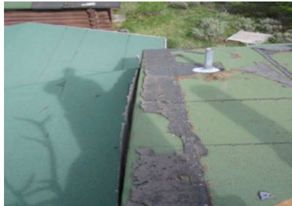
Layers of rolled roofing deteriorating
