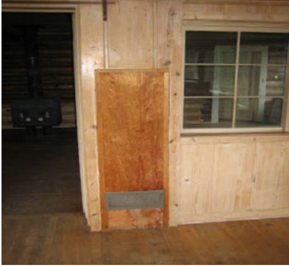
Figure 53 Wall heater in east enclosed porch
