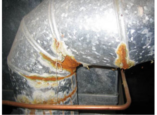
HVAC duct rusting 2
