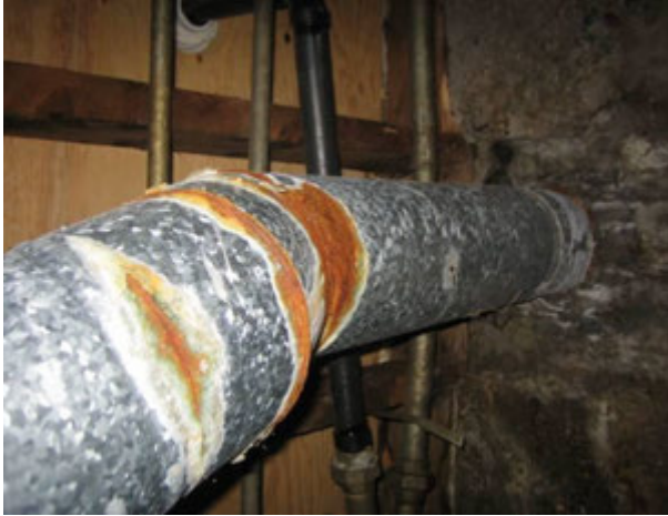
Figure 51 HVAC duct rusting
