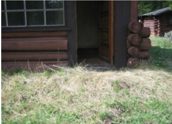
Figure 30 Negative drainage at bedroom 3 (Northwest Corner)
