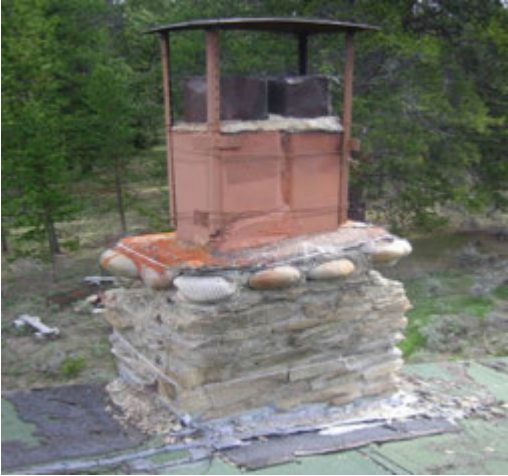
Figure 46 Flashing deterioration at fireplace
