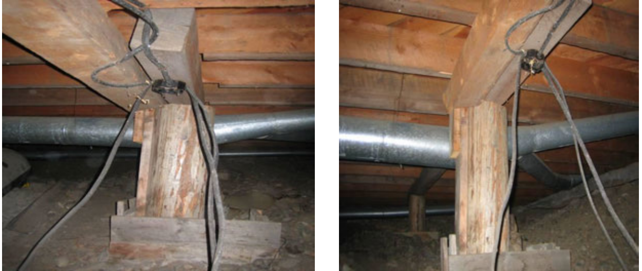
Figure 27 Improperly bearing beam
