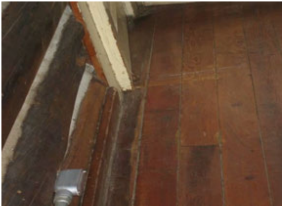
Figure 39 Bedroom #1 floor heaving
