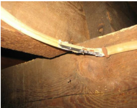
Figure 56 Bare wiring chewed by rodents
