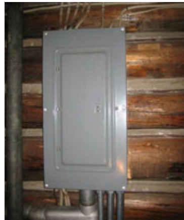
Updated electrical panel
