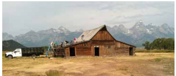
Volunteers replacing the roof on the TA Moulton Barn on Mormon Row.
