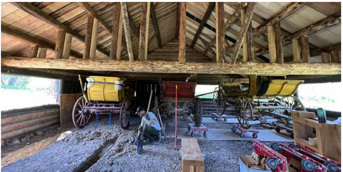
The historic wagons had to move sideways and underneath the beam of the Transportation Shed to exit the structure that needed repairs.
