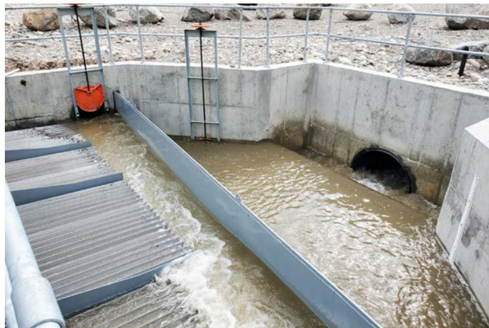
The improved Spread Creek structure is designed to prevent fish entrapment. Fish are caught by the fish screen and funneled back into the creek through the pipe with the red flap (irrigation water is routed out the larger opening).
