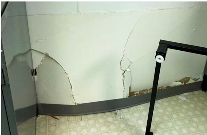
The damaged interior wall of the collection room at Colter Bay.
