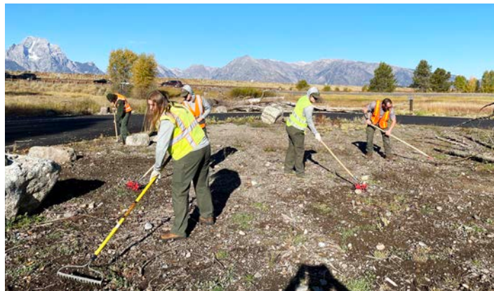
Vegetation staff rake in newly scattered native plant seed in a site disturbed by construction at Jackson Lake Dam.
