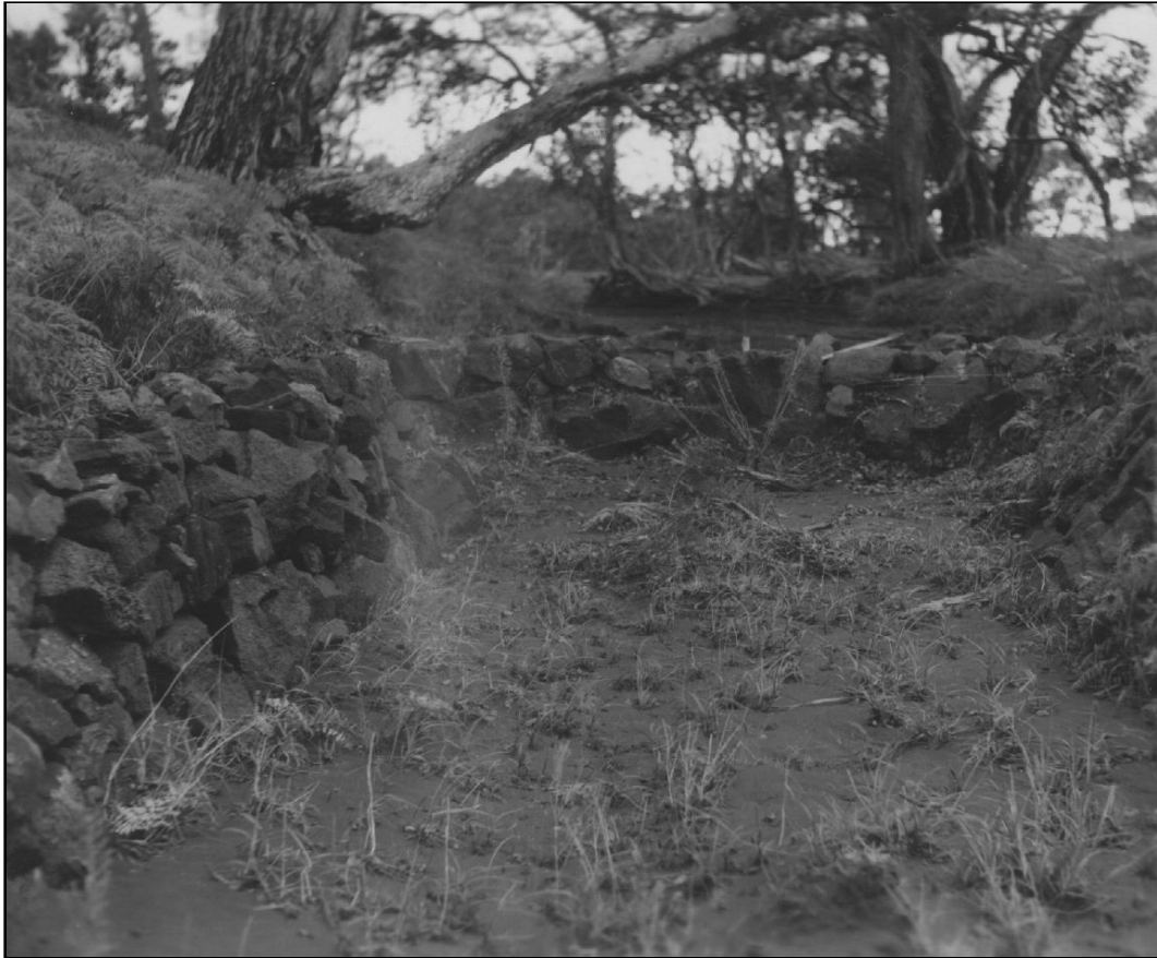
Figure 24. “Hilina Pali erosion control project deposition and vegetation above check dam, 8 months after installation.”
