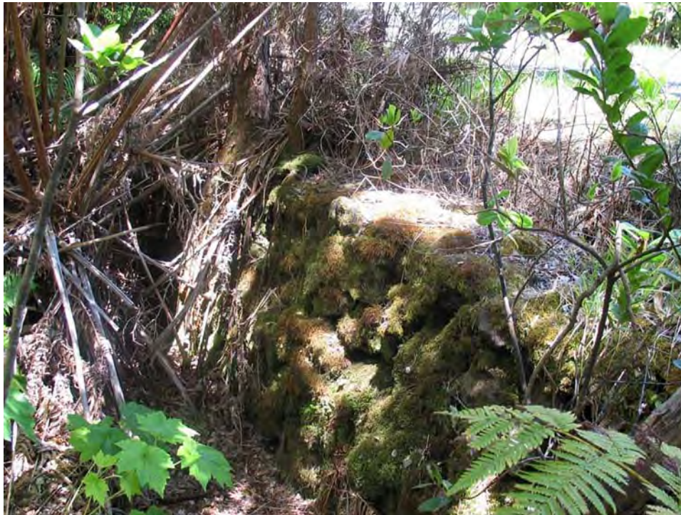
Circulation #3. Several remnants of retaining walls mark former road alignments of Crater Rim Drive. The wall remnants, which date to before the 1920s, are mostly hidden in the dense vegetation near the current road south of Thurston Lava Tube. (PWRO 2005)
