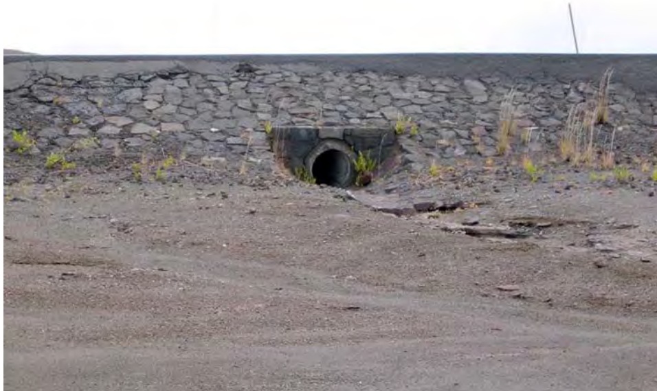
Circulation #1. Contemporary photo of the mortared-stone embankment facing and raised roadbed with culvert, located in the Southwest Rift Zone. Asphalt covers the top of the embankment from successive road paving. (PWRO 2005)
