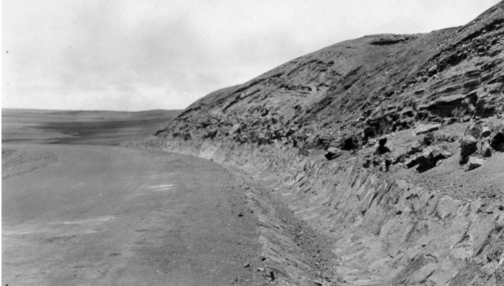
History #9. This stone-lined ditch was built by the CCC after heavy rains damaged the newly-built Uwekahuna-Bird Park road. This ditch is located on the grade just west of Halemaumau. (HAVO Landscape Architect's Reports 1934)
