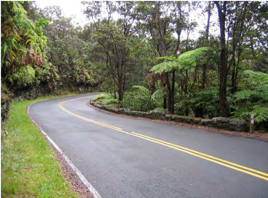
Buildings and Structures #6. The guard wall at the Thurston Lava Tube parking lot is lower than when it was constructed, either from settling, a build-up of paving matrix, or a combination of both. Compare with photo History #7. (PWRO 2005)
