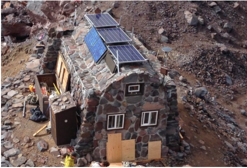
Figure 18 The installation of new solar panels for the microwave communications bridge to Camp Schurman
