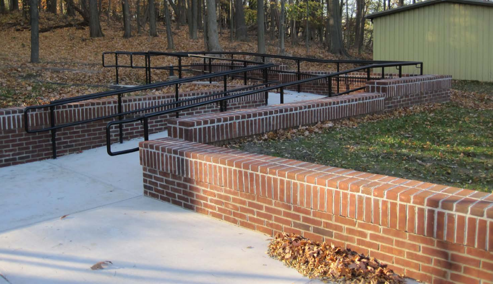
Completed accessible walkway and brickwalls with handrails at Morrystown National Historical Park.
