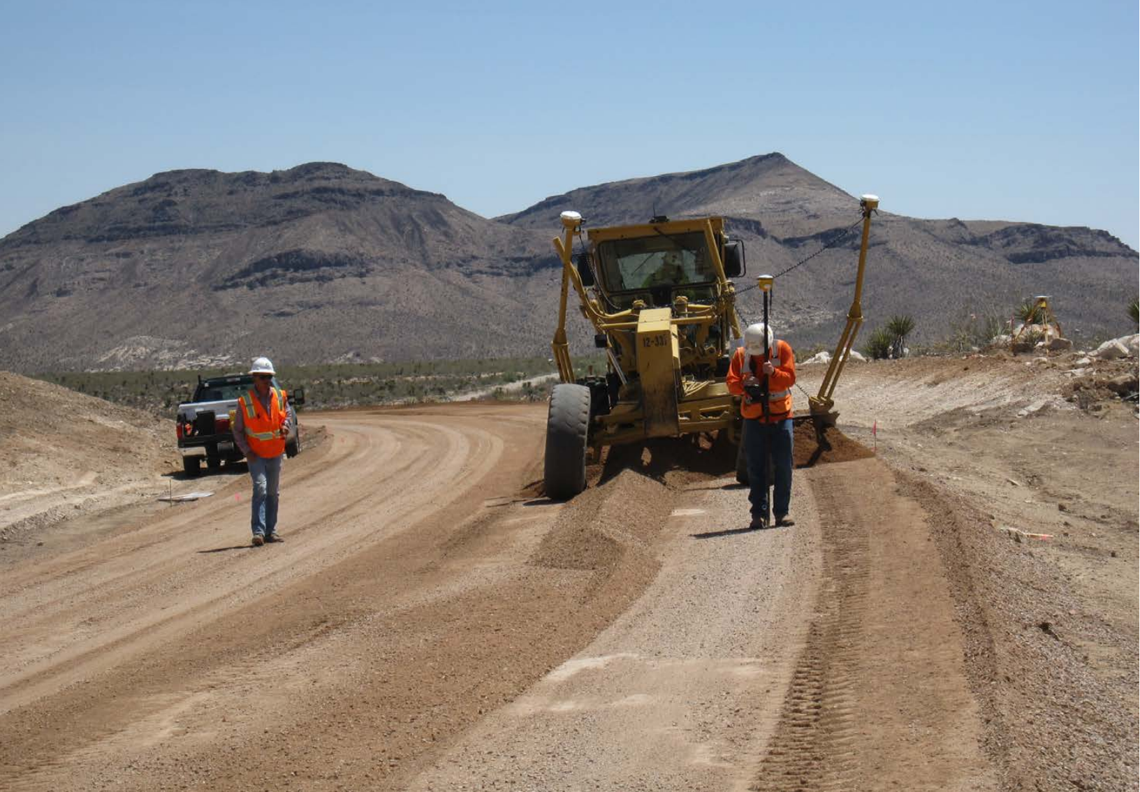
Safety improvements, including full reconstruction of high accident locations on Route 10 Kelbaker Road, at Mojave National Preserve. The new roadway provides a safe, consistent 24-ft paved top width with 10.5-ft lanes with 1.5-ft shoulders.
