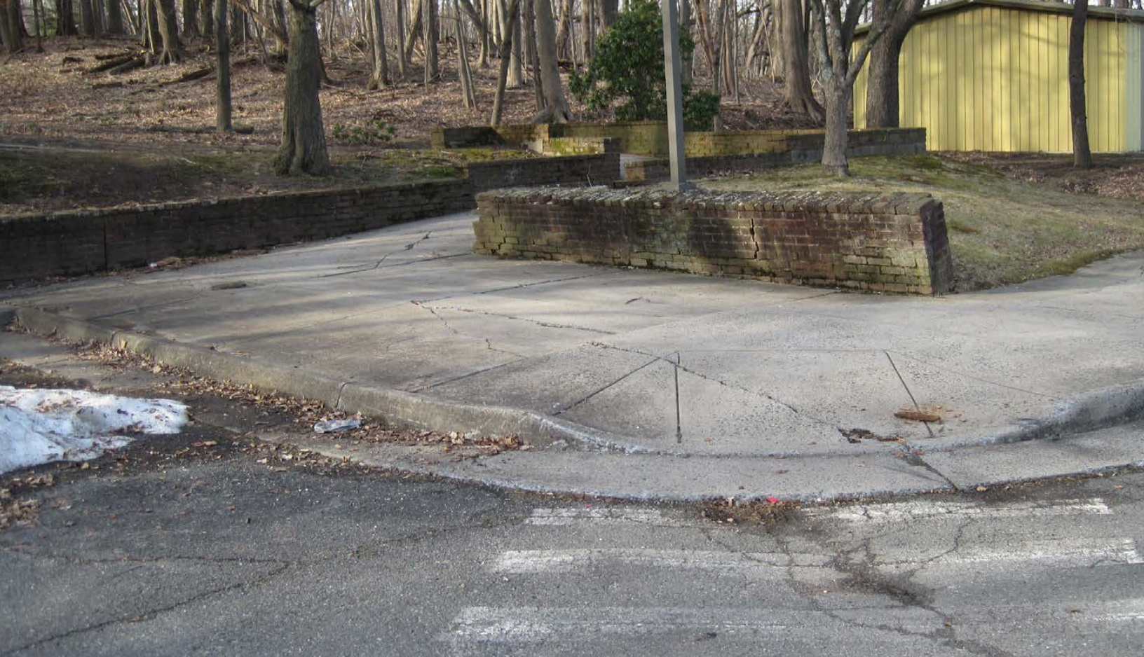
Deteriorated brick walls and inaccessible walkway at Morristown National Historical Park.
