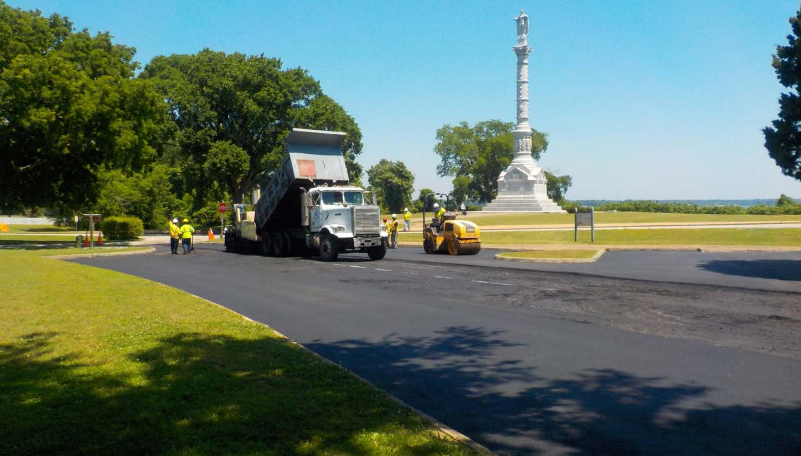
Final pass asphalt applied in the Victory Monument parking lot in Colonial National Historical Park.
