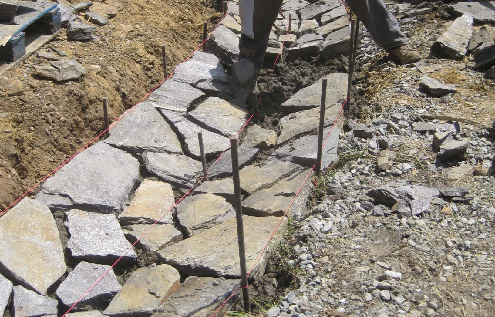
New stonework at Blue Ridge Parkway will improve drainage and extend the life cycle of the roadway.
