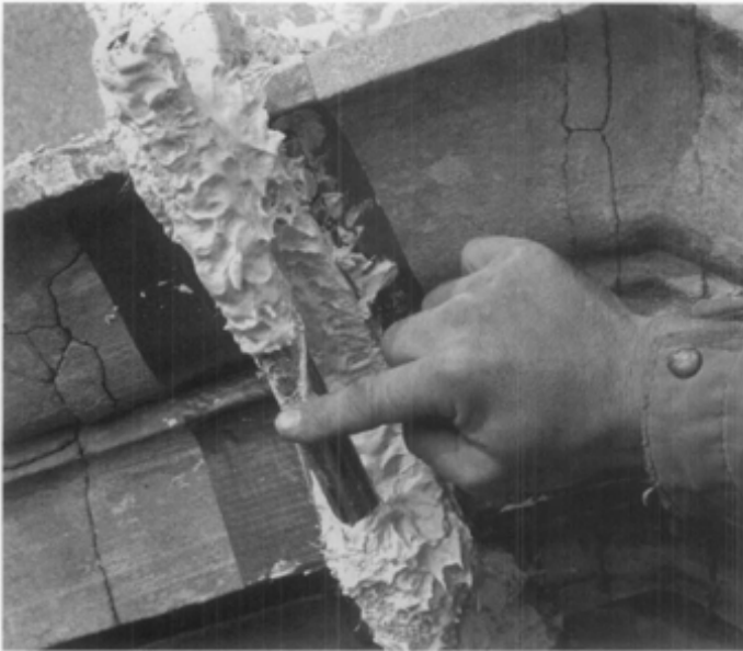
Figure 19. Molds for the replication of cast stone may be made on site using rubber materials and reinforcement. The molded profile of this window pediment will be used to run a plaster mockup, from which a production mold will be made. Photo: Michael Devonshire.
