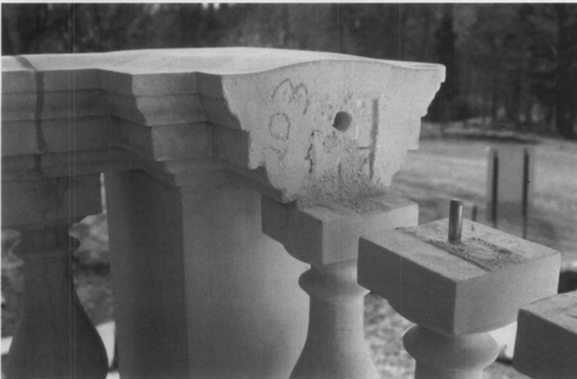
Figure 18. Long or thin cast stone elements require reinforcement. When possible, reinforcement of new cast stone should be made of stainless steel.
