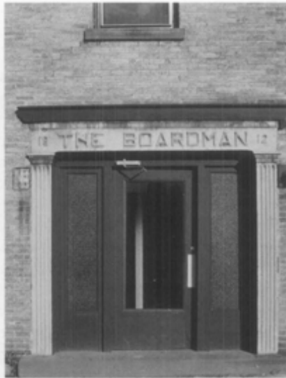
Figure 6. Cast stone was commonly used for molded trim in conjunction with brick or natural stone. This brick building in Rochester, New York, uses cast stone for the entry surround, and natural stone for unornamented window sills, thresholds, and water table units.
