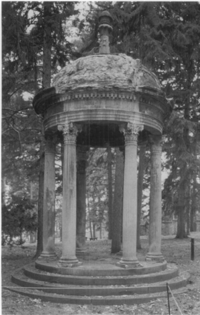
Figure 10. Scaling of cast stone units signals problems with the cementing mix and method of manufacture. Serious deterioration of cast stone, such as this, warrants replacement.
