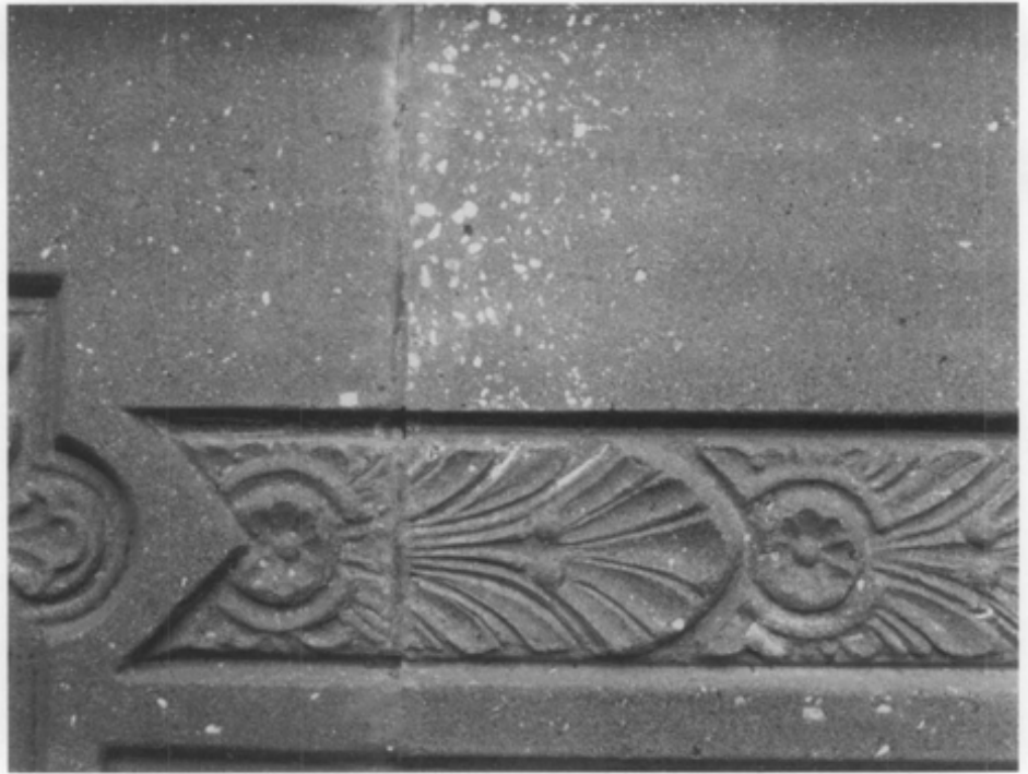
Figure 17. Unlike natural stone, cast stone generally may not be tooled in place to reduce lippage of uneven surfaces at joints. Tooling often exposes coarse aggregate from below the surface.
