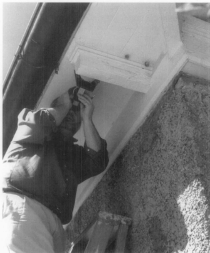
Figure 13. Paint studies may not only help establish the chronology of paints and paint colors used on a building but also may aid in the dating of existing architectural features. Examination of the paint layers on these modillions utilizing a hand-held microscope enabled an investigating team to confirm in the field which modillions were original and which were later replacements. Photo: Charles Fisher, National Park Service.
