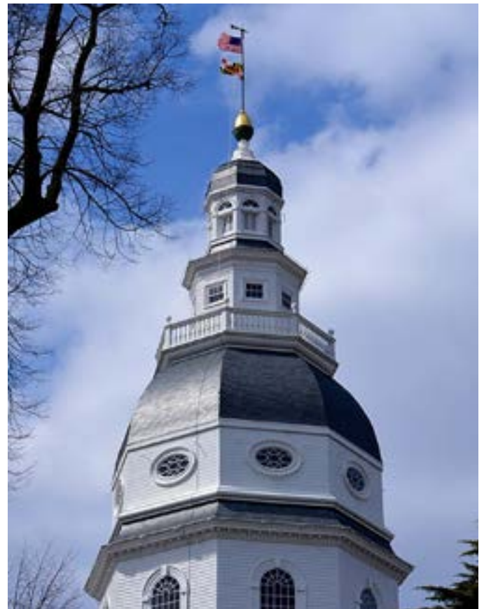
Figure 7. The c. 1788 wrought-iron lightning rod on the Maryland State House dome measures 28 feet in height, 2-1/2 inches square at its base, and is pointed at its top. The rod passes through a decorative copper-paneled wood acorn that is nearly 4 feet in diameter. The acorn helps provide stability to the rod that, in turn, is secured to the pedestal or base of the acorn. While based on the Franklin system, this rod had a decorative flare, including a weathervane and ornamental base. Prominently located in Annapolis along the Chesapeake Bay, an area of frequent summer lightning storms, the building has been struck by lightning as recently as 2016, surviving undamaged. Photo by Niagara (Own work) [CC BY-SA 3.0 ( http://creativecommons.org/licenses/by-sa/3.0/ )], via Wikimedia Commons.
