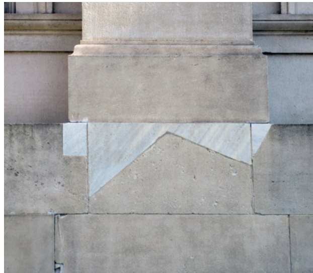
[3] Not Recommended: Although the Dutchman stone repair has been well executed, the replacement stone is not a good color match.
