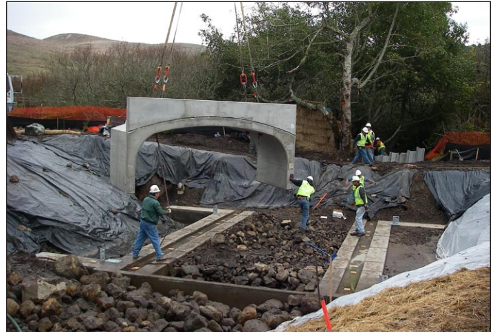
Workers place a piece of the bottomless culvert at the Estero Road crossing.
