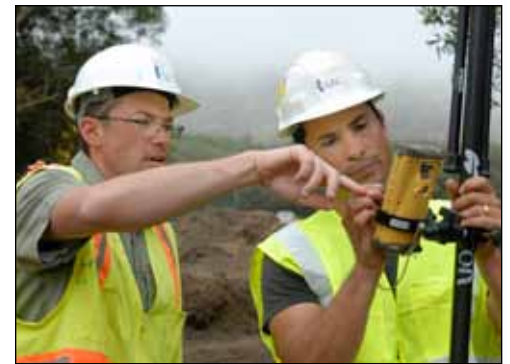
Construction staff check grading elevation in 2009. Where to dig and to what level was decided with the help of previous coring data.
