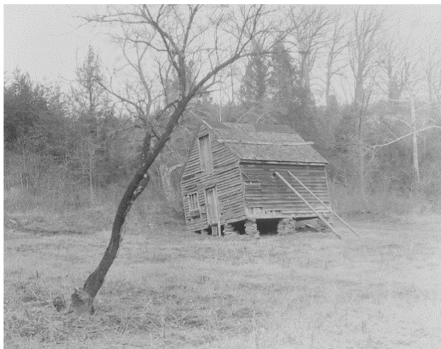
Figure 5.1 Photo of a Dilapidated Building at Missouri Mill Taken by Charles Gerner, NPS, on an Explorative Trip to Assess the Potential of the Area as an RDA
