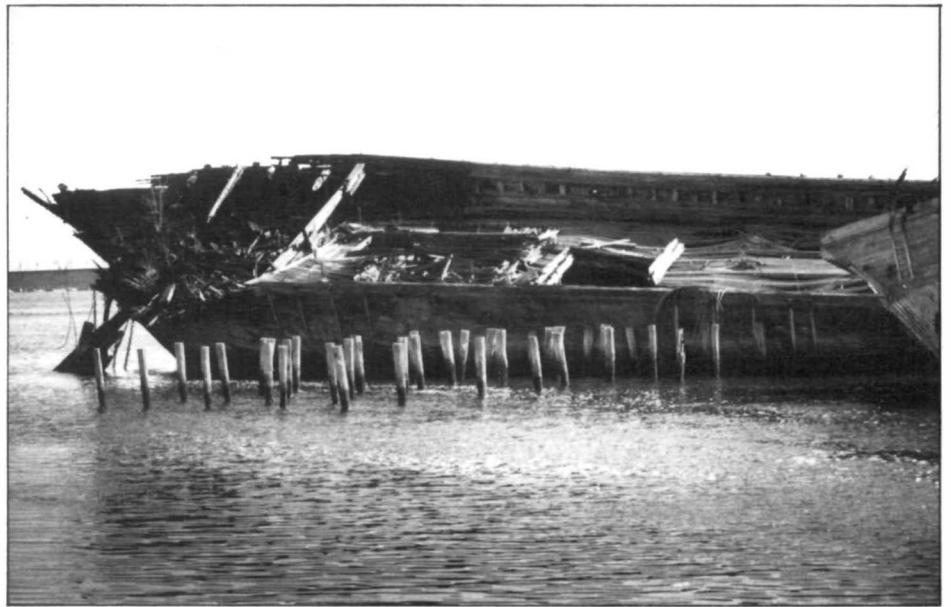
FIGURE 5: The deteriorating hulks of the four-masted schooners Hesper , and Luther Little lie off Wiscasset, Maine. (Photo credit: James P. Delgado, NPS)
