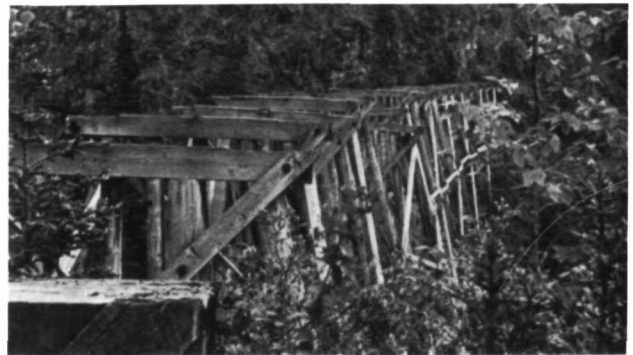
Engineering structures associated with transportation lines, whether currently used or not, should be included in the survey. The Copper River and Northwestern Railway, Chitina vicinity, Alaska, was constructed to gain access to the interior copper country and thus, is closely associated with a major economic activity in this area. The National Register of Historic Places listing includes 25 miles of railroad bed, sections of track, trestles, and associated buildings. (Alaska Division of Parks)
