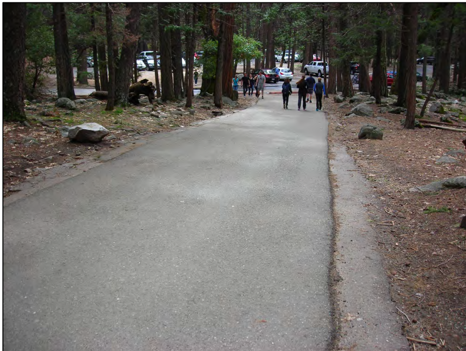
Photo F-4. Bridalveil Fall Trail: Contributing Structure in the Yosemite Valley Historic District. View looking southwest toward connection with parking lot.
