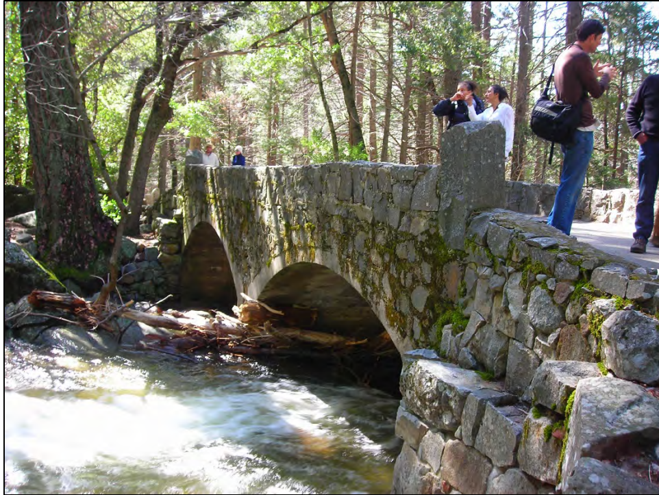
Photo F-7. Bridalveil Fall Bridge #2: Contributing Structure to Yosemite Valley Historic District. View looking southwest from streambank.
