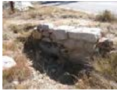
Partially blocked culvert.
