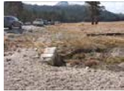
Culvert set too low in meadow.
