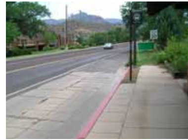
Pavement Condition at Bit & Spur Shuttle Stop
