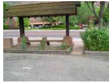
Faded Parking Paint and Shuttle Stop Shelter
