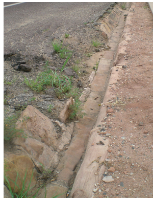
Eroding gutter at Terrace Brook Lodge
