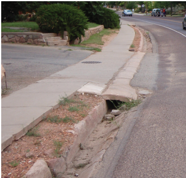
Debris in gutter and deterioration of the rock ditch wall at the elk ranch
