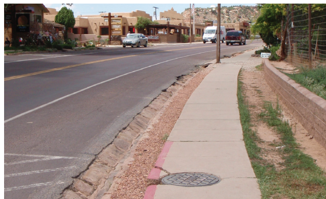
Sidewalk cracking at manhole cover
